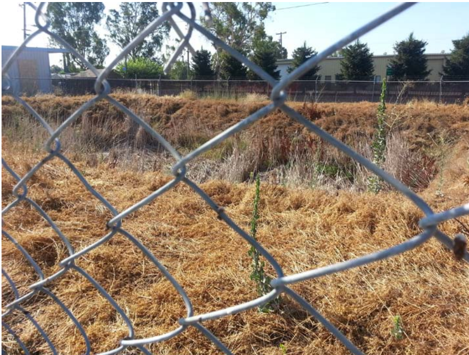
Storm water retention pond
