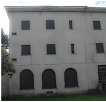
Cracks on the eaves molding over the façade on the right side. (Source: Martín Capeluto / MSME)
