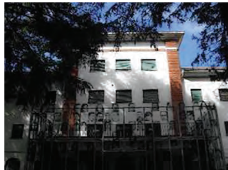
Fissures and detachment of the render on a lintel at the Second Floor, situated over the axis of the central volume of the main façade. (Source: Martín Capeluto / MSME)
