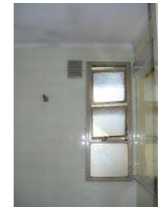
Functional damage on windows on the First Floor: in a dormitory (left) and in a bathroom (right). (Source: Martín Capeluto / MSME)
