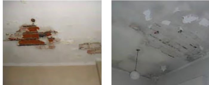
Reinforcement bars rusting together with the lack of its protective coating on slabs located at the Ground Level. (Source: Martín Capeluto / MSME)
