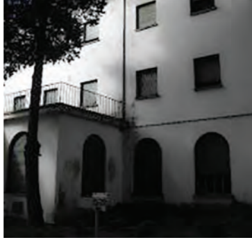
Cracks without detachments on the eaves molding over the left volume of the principal façade. (Source: Martín Capeluto / MSME)
