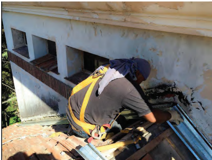
Repair of tiled roofs through valley flashing details to improve waterproofing. (Source: Martín Capeluto / MSME)
