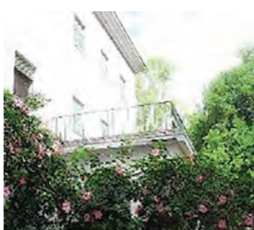
Fractures with partial detachments of the cornices in the lower volume over the right side of the main façade (Source: Martín Capeluto / MSME)
