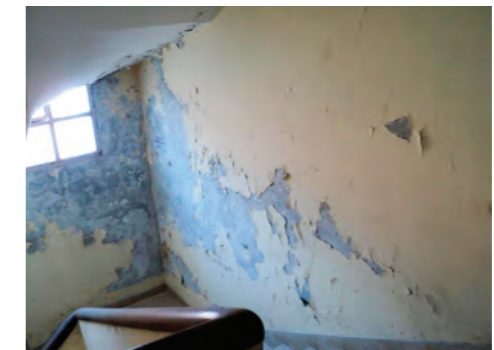
Interior building surfaces: before (above and center) and after (below) cleaning and consolidation procedures. (Source: Martín Capeluto / MSME)
