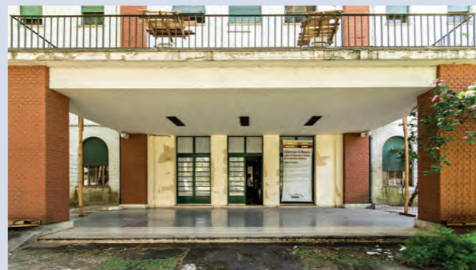
Semi-covered entrance, first signposting posters. (Source: ESMA Museum and Site of Memory)
