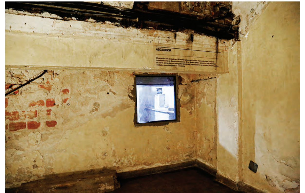
Basement Room. Open shaft in the wall to inspect the constructive marks left by the existence of the elevator. The finding was left visible and protected by placing a glass panel. (Photo 32: Camilo del Cerro / MSME)
