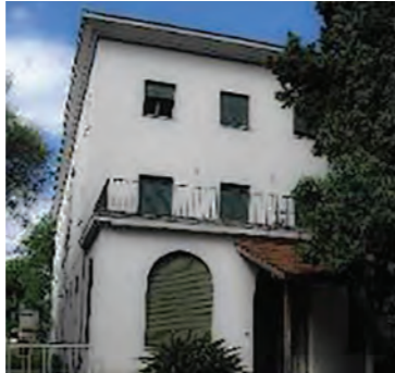
Fractures with partial detachments of the cornices in the lower volume over the left side of the main façade. (Source: Martín Capeluto / MSME)
