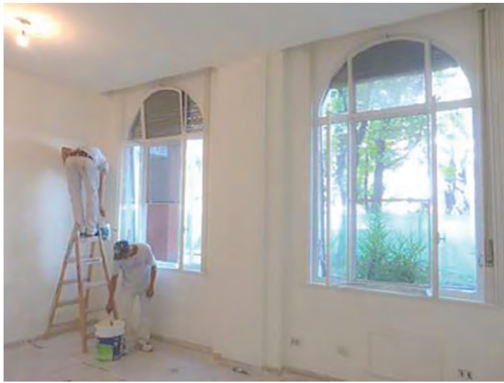
Renovation of paint coatings in the Meeting Room on the Ground Floor. (Source: Martín Capeluto / MSME)
