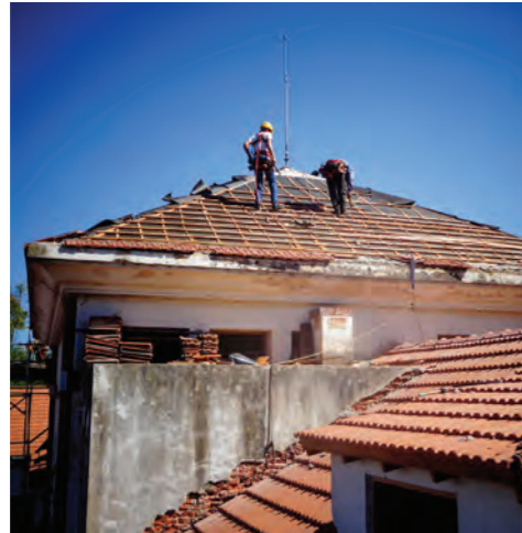
Recovery of materials (roof tiles, rafters and wooden boards) and selective replacement of damaged materials. (Source: Lucía de Lisi)
