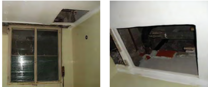
Reinforcement bars rusting together with the lack of its protective coating on a beam located in a dormitory on the First Floor. (Source: Martín Capeluto / MSME)
