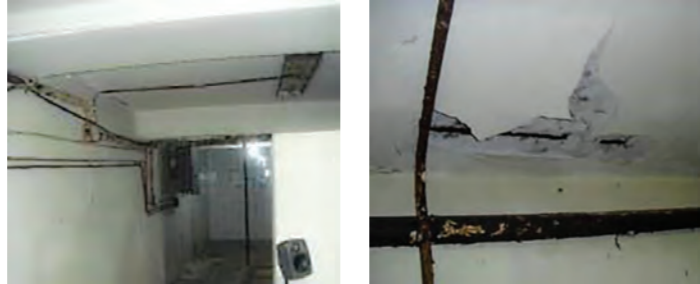
Reinforcement bars rusting together with the lack of its protective coating on slabs located at the Basement Level, underneath the main hall. (Source: Martín Capeluto / MSME)
