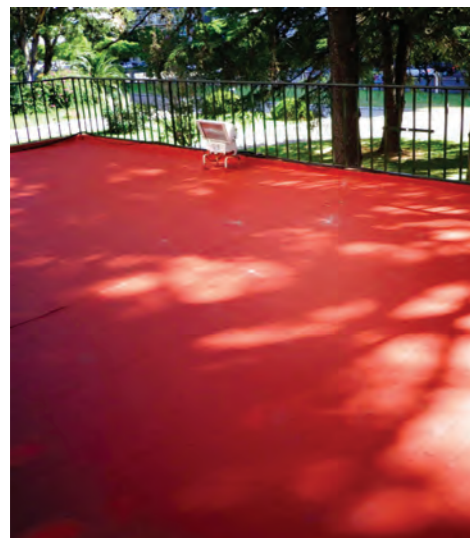
Placement of waterproof insulation in the accessible terraces (left), and in the service terraces (right) over and without removing the original building fabric. (Source: Lucía de Lisi)
