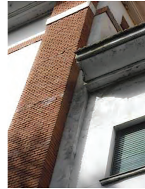
Horizontal cracking in the brick veneer seen on the main façade, at the intersection of the central and side volumes. (Source: Martín Capeluto / MSME)
