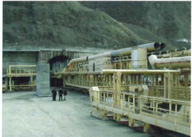
TBM Robbins is ready to start driving of the first headrace tunnel
