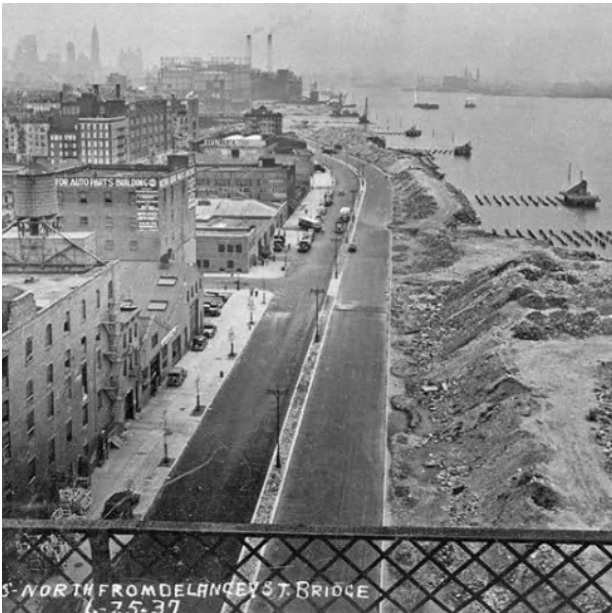
The construction of ‘East River Drive,’ later renamed as FDR Drive (NYPL, 1937)
