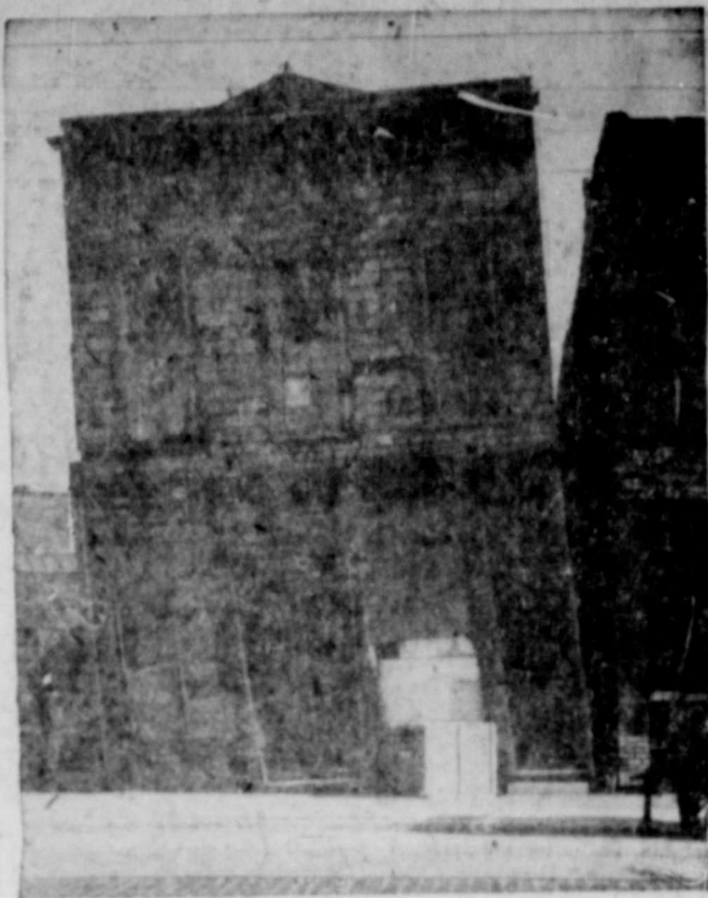
Caught in the high seas of the housing shortage, residents of this tenement must really feel like they're out in a storm, considering the way the building lists. It's on Chicago's Blue Island Avenue, and its sag doesn't seem to bother either the tenants or the landlord.
