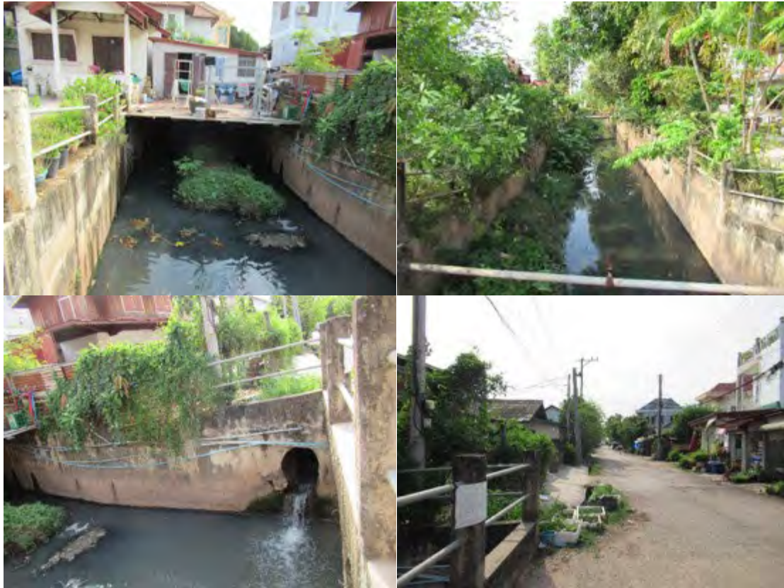
Condition of drainage in Ban Akart area
