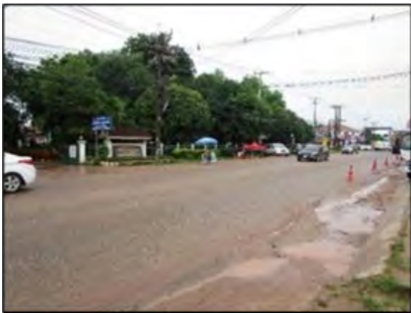
Hospital No Parking Lot, No Chevron Marking
