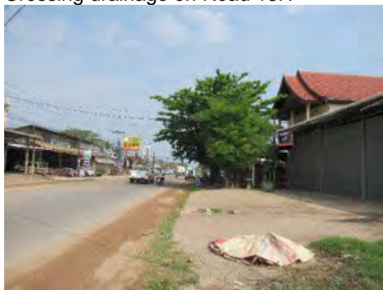
Condition of the road in the north next to the crossing drainage no. 2
