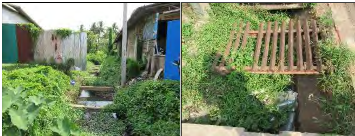
Figure 12: Example of Poorly Maintained Local Drainage System
