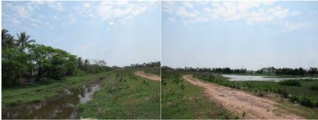
Condition of Nong Or canal
