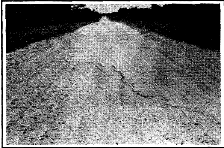
COMPLETE LOSS OF ASPHALT
