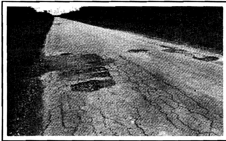
BAD CRACKING AND POTHOLES
