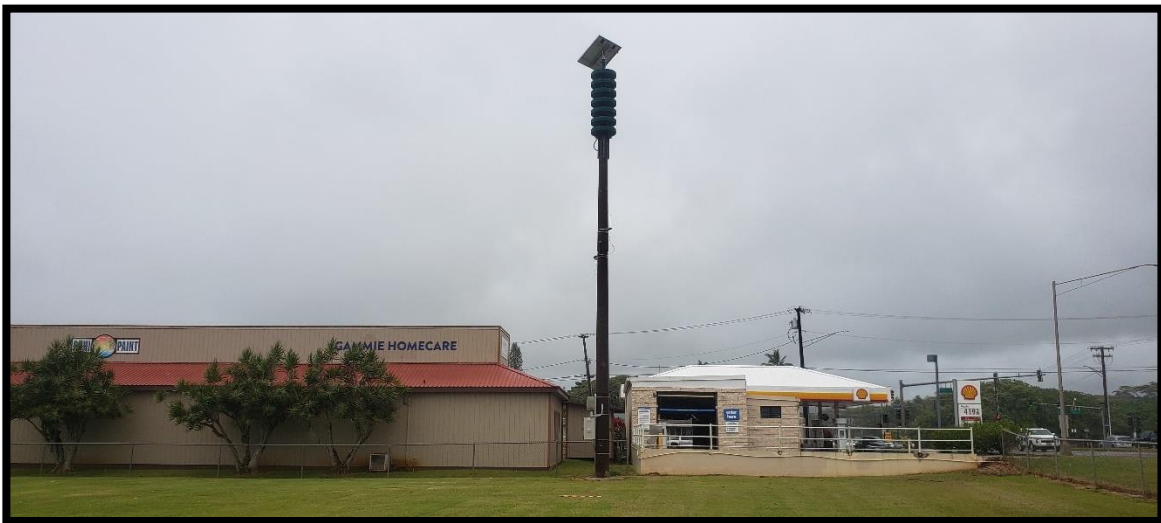
Figure 26. Overview photo of the Puhi town emergency alert and warning siren looking west
