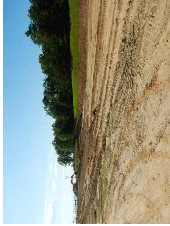
Photograph 12. View from the center of ATCT 2a to the southeast site corner (6/2/2020).
