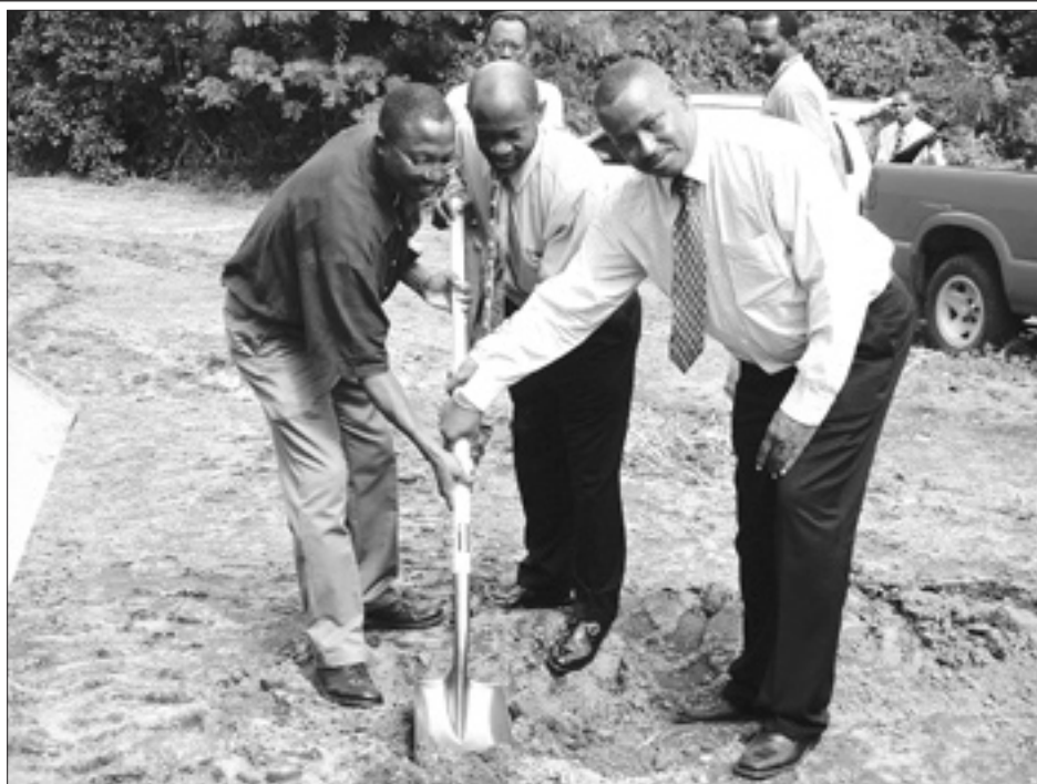
From left: CEO of UTS CariGlobe Clecton Phillip, St. Kitts-Nevis Prime Minister Dr. Denzil Douglas and UTS CEO Julio Constansia turn the sod to mark the official start of construction of the UTS CariGlobe Chippie network in the twin-island federation
