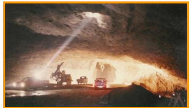
Figure 5. The UDEC-BB model shown above, gave a good (Class A) prediction of 7 to 9 mm downward movement. (Barton et al. , 1994). A view of the huge (stages 1 to 4) top-heading is shown.
