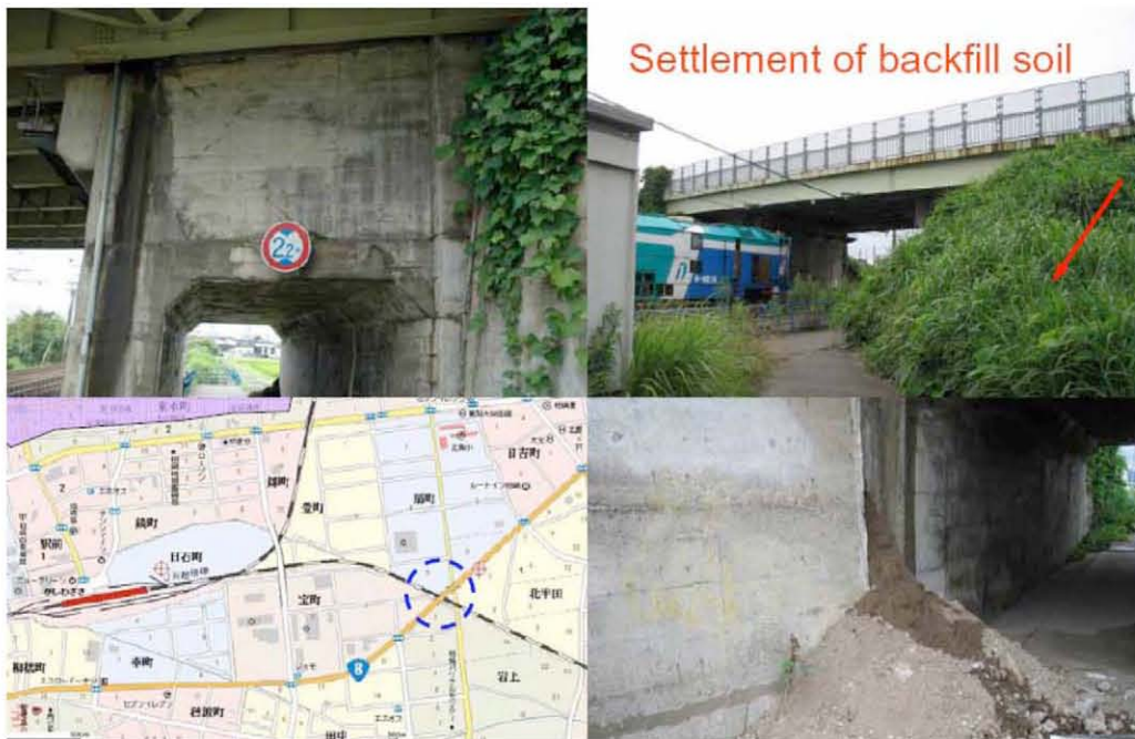
Fig. 6.17. Damage and repairs where railway crosses Highway 8 Bridge (courtesy G. Watanabe, Tokyo Institute of Technology).
