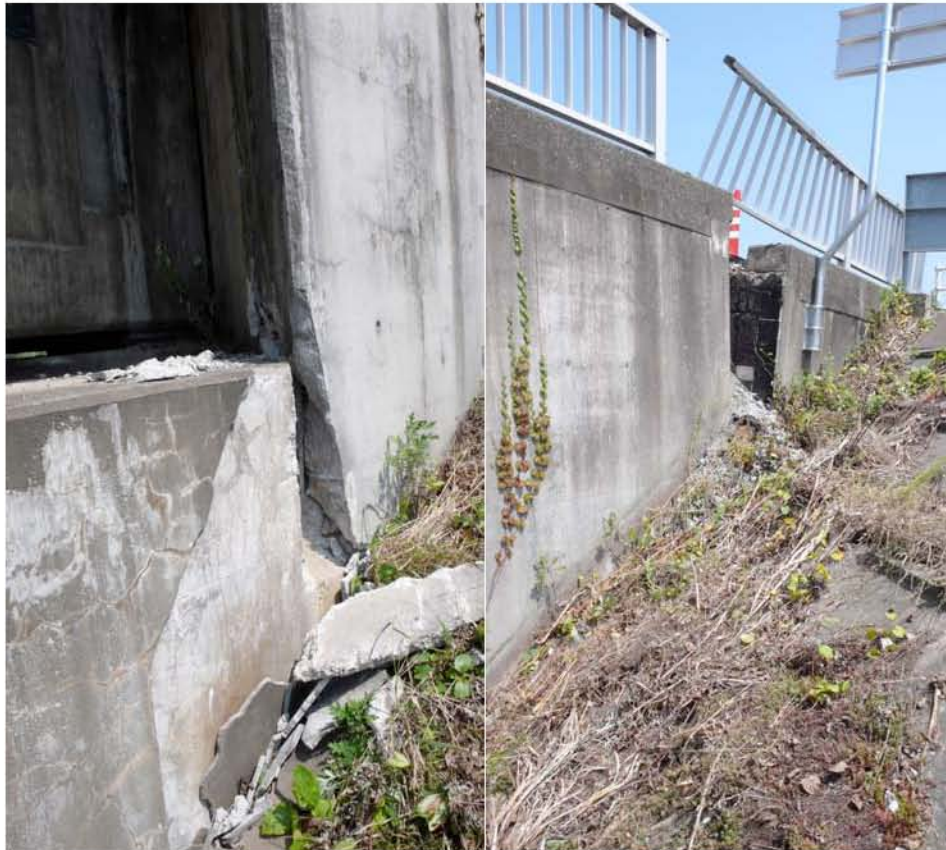
Fig. 6.51. Abutment and wingwall damage from the earthquake.
