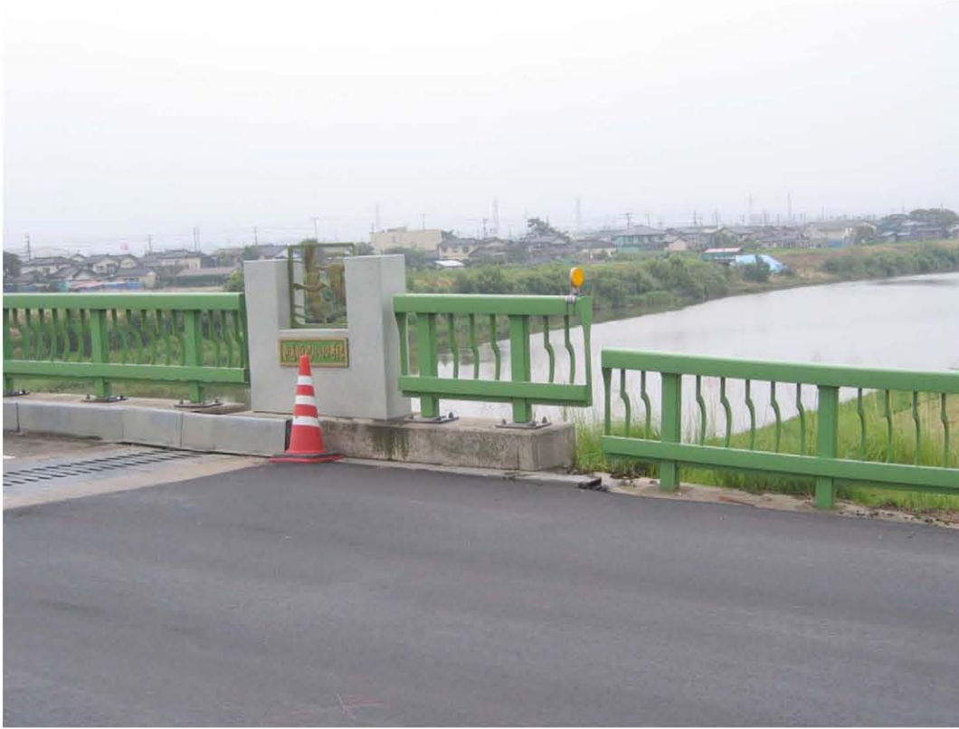
Fig. 6.35. Settlement of north bridge approach.
