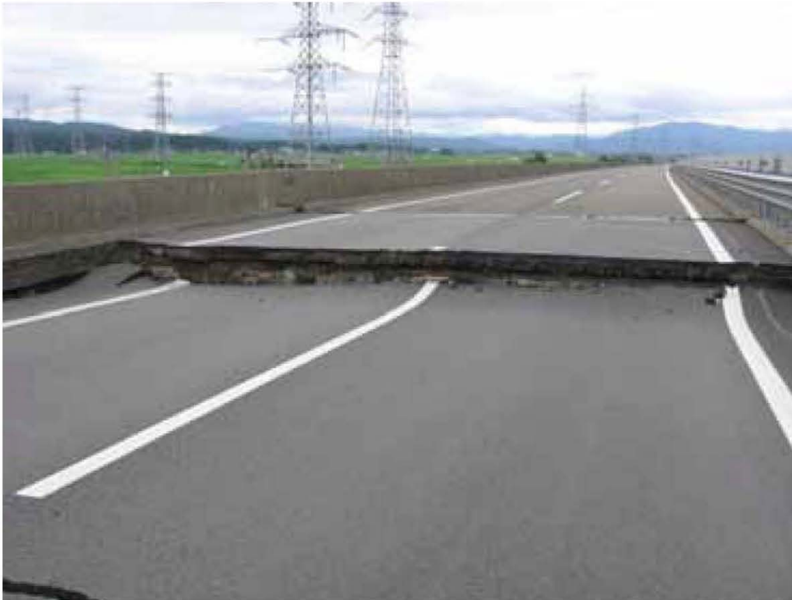
Fig. 6.8. Damage to approach slab and embankment at Yoshiigawa Bridges.
