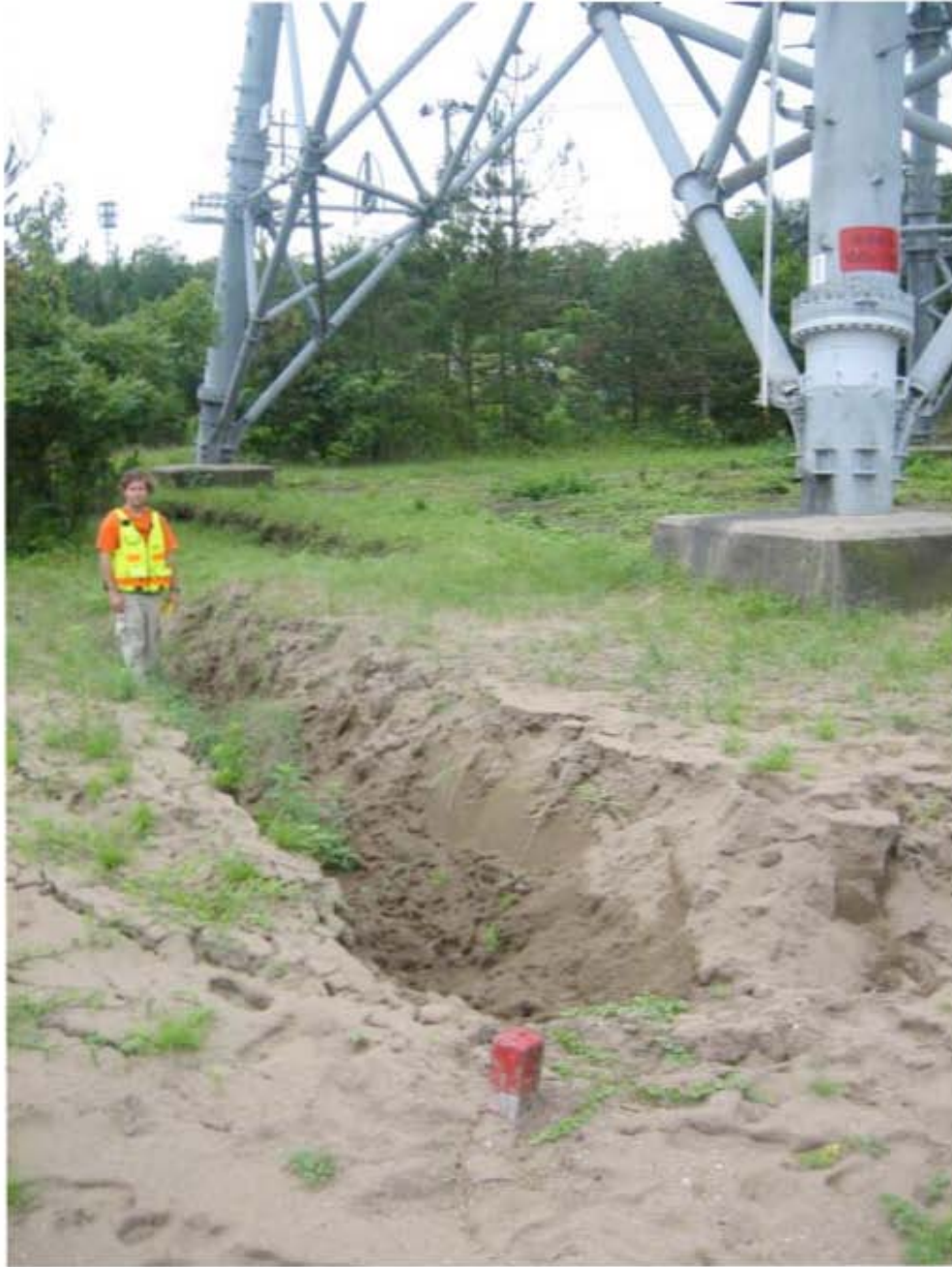
Figure 4.35: Settlement of ground adjacent to grade beam between footings of a high voltage transmission line tower (Site RK40, N37.41633° E138.60792°, 7/22/2007).
