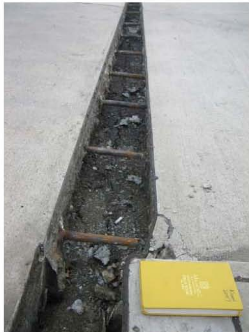
Figure 4.20: Kashiwazaki Harbor - South area experienced ground damage from liquefaction-induced lateral spreading resulting in separated pier slab sections (Site RK25, N37.36713° E138.53210°, 7/20/2007).
