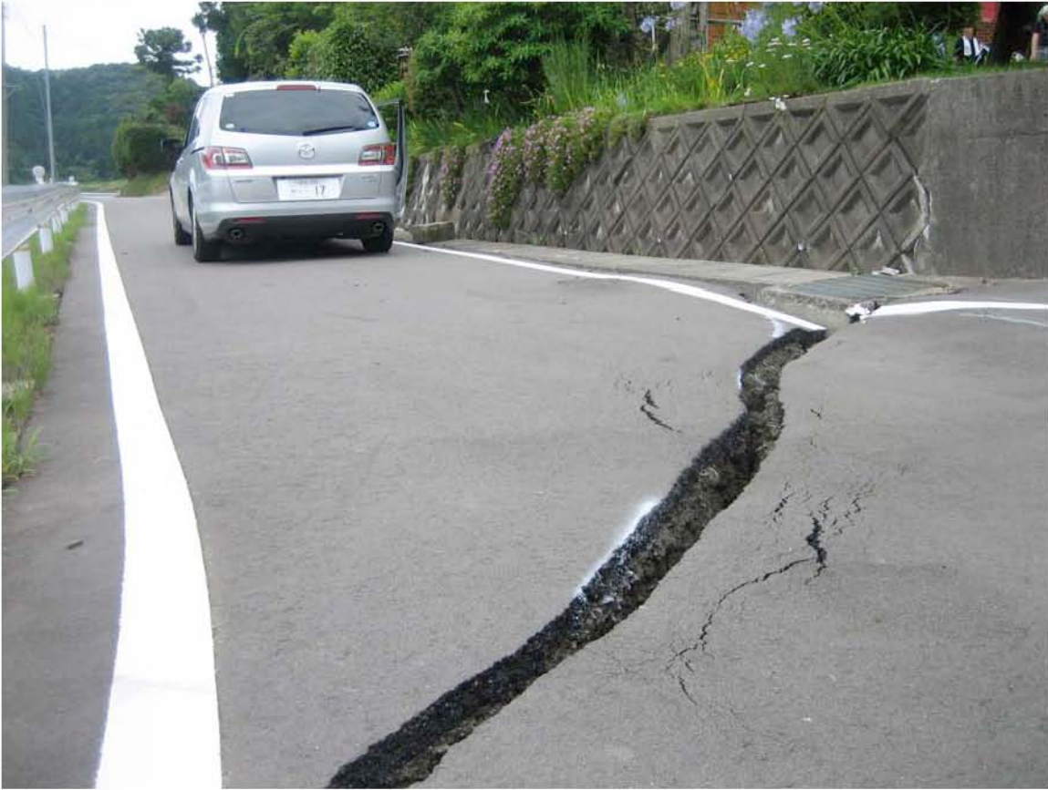
Figure 9.5: Typical road damage near epicentral region (Site RK30, N37.45727° E138.65328°, photo taken 7/22/07 09:46). Cracks of 5 to 10 cm were often quickly paved over in high-traffic areas, within one or two days of the earthquake. On local community roads with alternate traffic routes, this damage was not immediately repaired.
