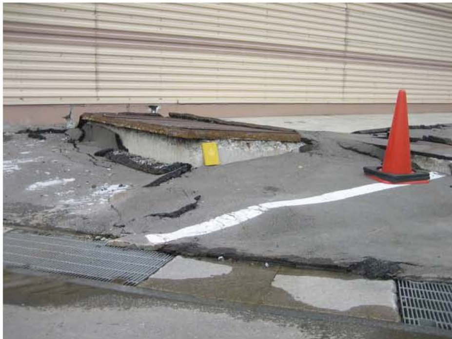
Figure 4.36: Plant 5 Store - Ground settlement in dune sand was observed around the building and an underground storage tank had been uplifted (Site RK41, N37.41468° E138.6084°, 7/22/2007).
