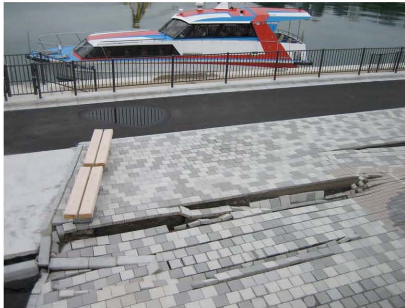
Figure 4.23: Kashiwazaki Harbor - The southern area experienced ground damage from liquefaction-induced lateral spreading and settlement. A harbor-front caisson rotated toward the harbor, uplifting the asphalt and tiled section shown here and initiating lateral displacement of the soil behind it, between the caisson and port building (Site RK25, N37.36713° E138.53210°, 7/20/2007).
