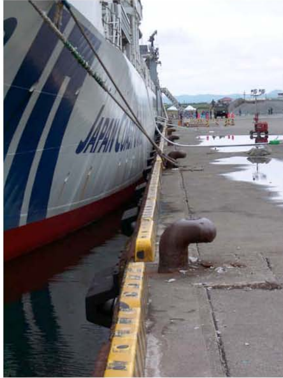
Figure 8.23: Kashiwazaki Port - Evidence of very minor lateral movement of quay walls and minor settlement located along the northern face of the terminal used as the berth for the Japan Coast Guard (Site SD8, N37.36680° E138.53825°, photo taken 7/22/07 15:22).
