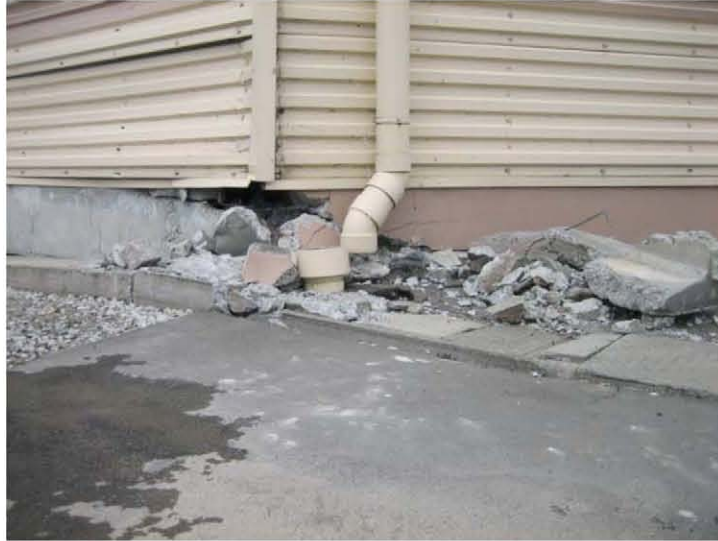
Figure 4.37: Plant 5 Store showing foundation corner area of failed reinforced concrete. (Site RK41, N37.41468° E138.60840°, 7/22/2007).
