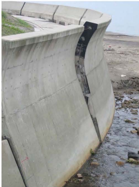
Figure 8.42: Rotation and lateral displacement of the concrete seawall (Site RK37, N37.45478°, E138.60927°, photo taken 7/23/07).
