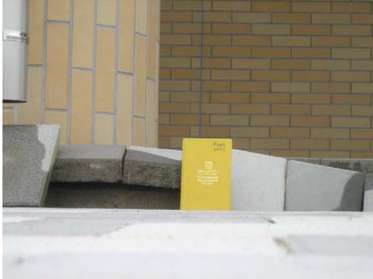
Figure 4.19: Kashiwazaki Harbor - South area experienced ground damage from liquefaction-induced lateral spreading and settlement immediately adjacent to the pile-supported port office building. (Site RK25, N37.36713° E138.53210°, 7/20/2007).
