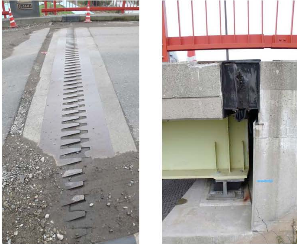
Fig. 6.43. Distortion of expansion joint, bearings, and abutment on Kaiun Bridge.
