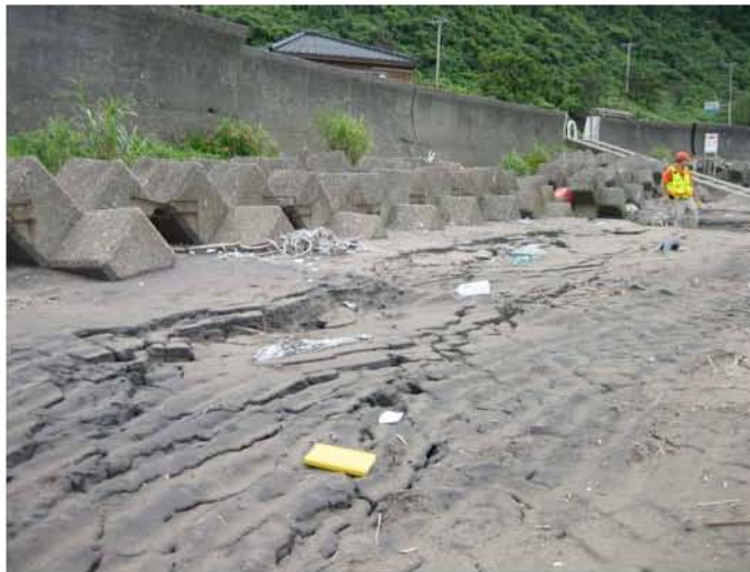
Figure 8.44: Lateral spreading associated with liquefaction of beach sand (Site RK35, N37.48497°, E138.62645°, photo taken 7/23/07).
