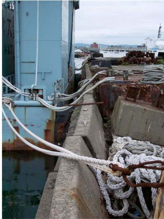
Figure 8.20: Kashiwazaki Port - Steel Scrap Transport Facility showing caisson displacement (Site SD6, N37.36668° E138.53565°, photo taken 7/22/07 14:56).
