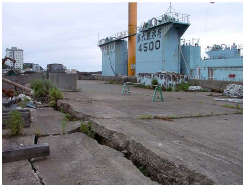
Figure 8.19: Kashiwazaki Port - Steel Scrap Transport Facility showing evidence of ground failure due to liquefaction of sand fill and damage to concrete aprons (Site SD6, N37.36668° E138.53565°, photo taken 7/22/07 14:46).
