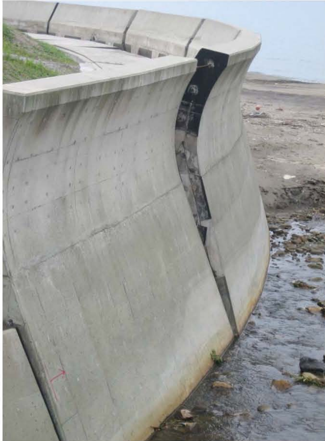
Figure 4.31: Seawall Failure as a result of embankment movement into a seawall founded on top of liquefied beach sands. (Site RK37, N37.45478° E138.60927°, 7/22/2007).
