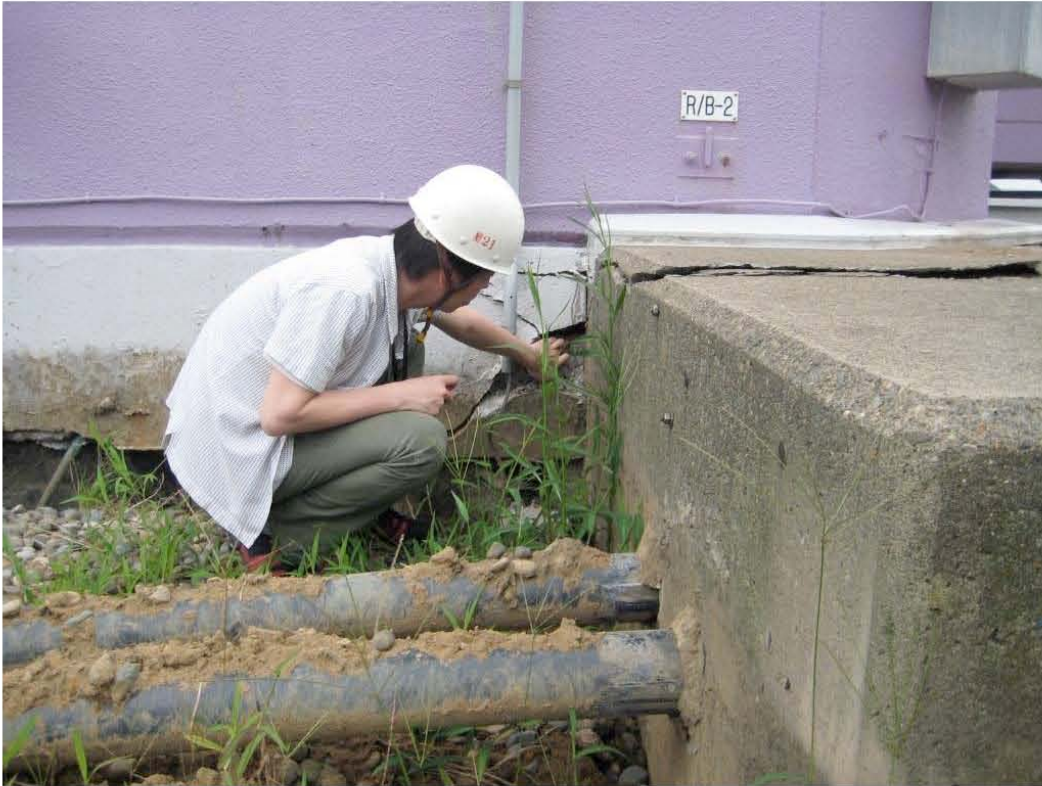
Figure 5.4: Cracks in reinforced concrete element at ground level.
