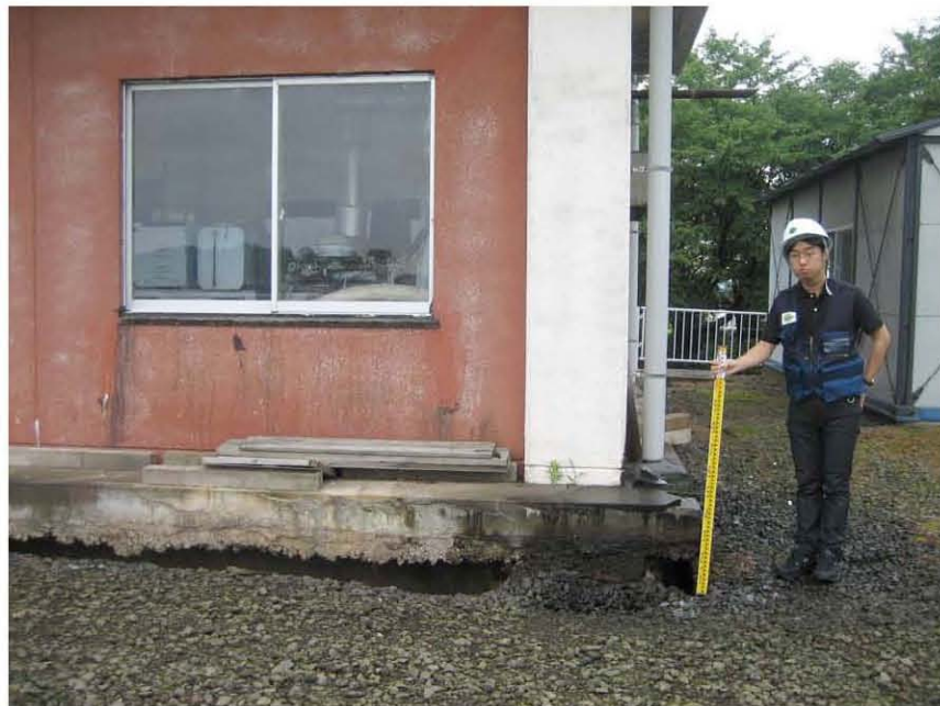
Figure 4.2: Fujii Weir downstream from Tashiou Bridge crossing of river. (Site RK16; N 37.34875^{\circ} E 138.61670^{\circ} , visited 7/21/2007 11:28 am UTZ+8). The control building exhibited damage to the foundation with settlement of fill beneath the structure.
