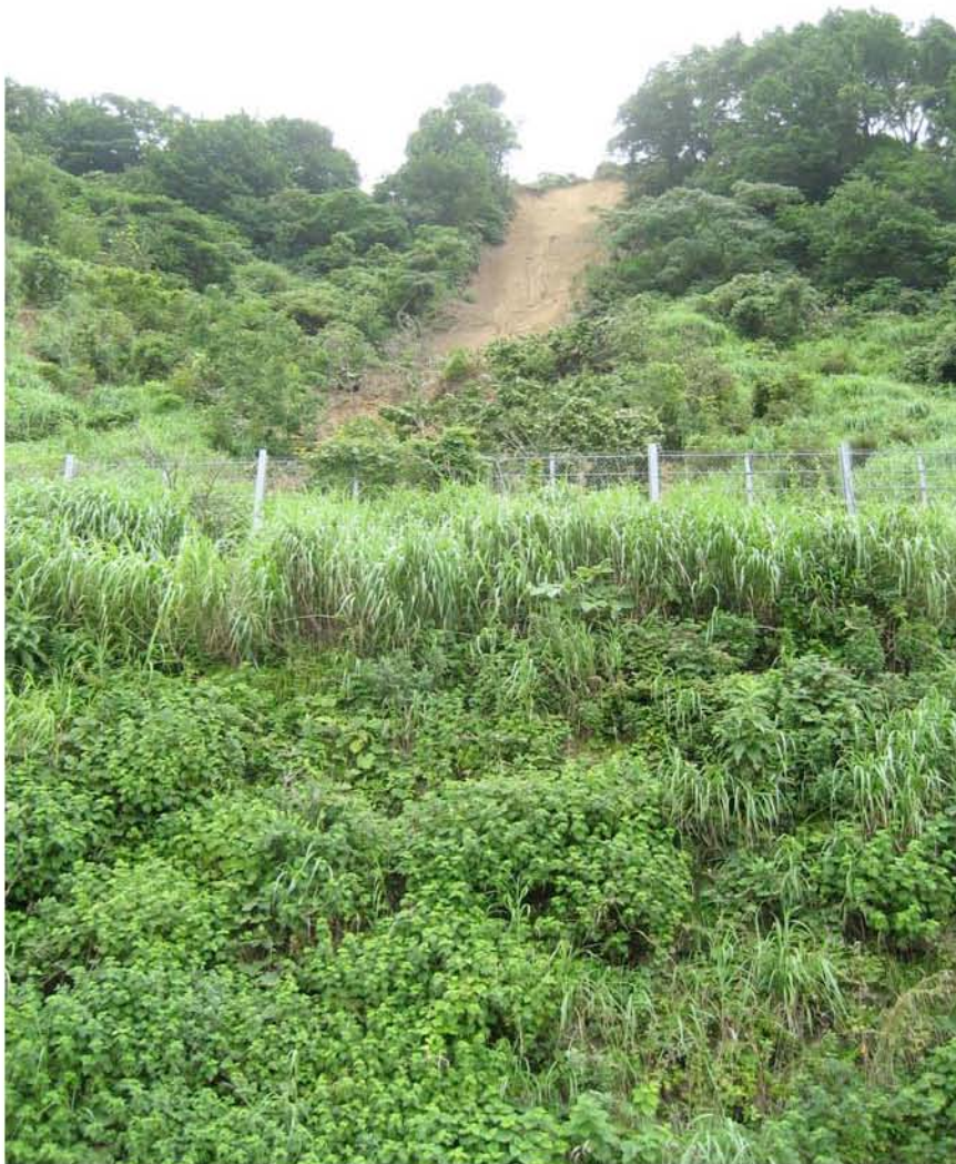
Figure 3.3: Coastal landslides on Highway 352 north of Kashiwazaki-Kariwa Nuclear Power Plant at road closure south of Route 373 (Site RK34-Slide 4; N37.48455° E138.62435°, photos taken 7/22/07 at approx. 10:45). This landslide is typical of many of those observed along the coast, and in this case did not damage transportation lines. Slide is approximately 10 m wide, 25 m long, and 0.5 m thick. Failure plane has approximate 50° inclination.
