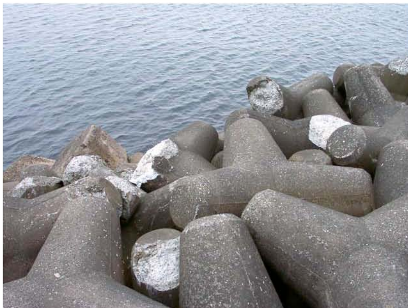
Figure 8.15: Kashiwazaki Port - Likely earthquake-related damage to tetrapod wave armor units (Located near site RK25/SA25/YT4, N37.36713° E138.53210°, photo taken 7/21/07 15:53).
