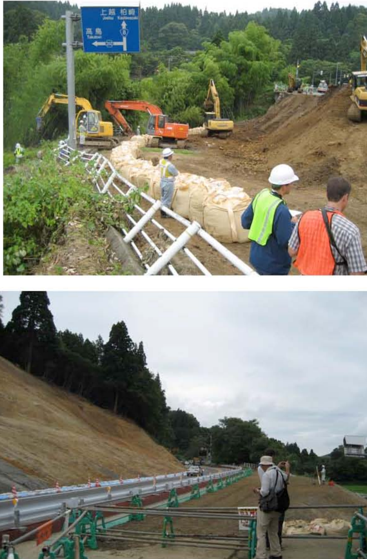
Figure 9.1: The Ozumi Senbon Landslide (Site RK1, N37.41422° E138.71347°), located along Highway 8 just north of the intersection with Route 252, closed both lanes of traffic. The upper photo, taken 7/20/07 at 11:30, four days after the earthquake, shows the displaced roadway which ran from the distance vehicles to the upper right of the photo to just in front of the investigation team members in the lower right. The bottom photo, taken 7/23/07 at 13:00, shows the nearly completed landslide and roadway repair, complete with guard rails, pavement, and center striping, just three days later.
