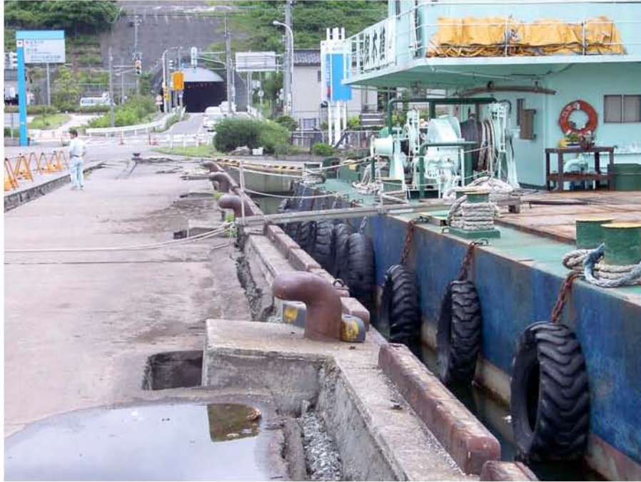
Figure 8.16: Kashiwazaki Port - West facing portion of the “Southwestern Pier” showing displacement of the sheet pile wall and ground settlement due to liquefaction of sandy backfill (Site SD5, N37.36532° E138.53213°, photo taken 7/22/07 13:57).
