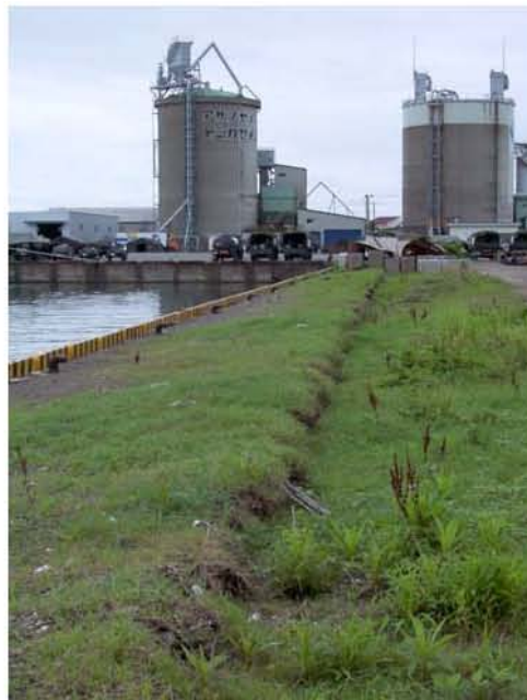
Figure 8.21: Kashiwazaki Port - North facing, landward quay wall exhibiting lateral movement and rotation of caissons (Site SD7, N37.36593° E138.53692°, photo taken 7/22/07 15:12). The Taiheiyo Cement Tanks are in the background.
