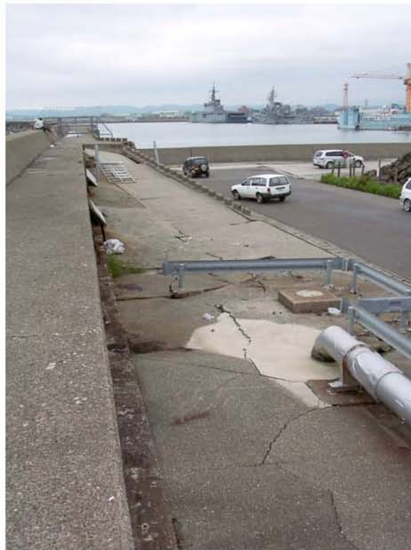
Figure 8.10: Kashiwazaki Port - Seawall and exposed end of the elevated asphalt pipe (Located near Site RK25, N37.36713° E138.53210°, photo taken 7/21/07 15:51).
