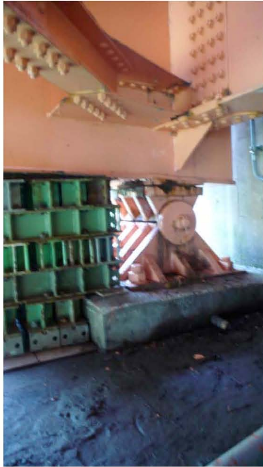
Fig. 6.27. Damage of set bolts and the additional steel box support to prepare the aftershocks)
