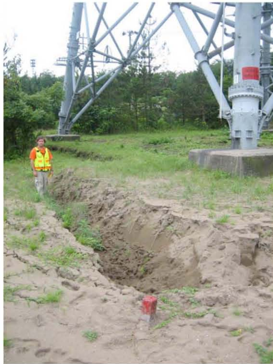
Figure 10.5: Ground failures at the site of a high voltage tower (Site RK40, N37.41633° E138.60792°, photo taken 7/24/07). No evidence of structural damage to the towers was observed.
