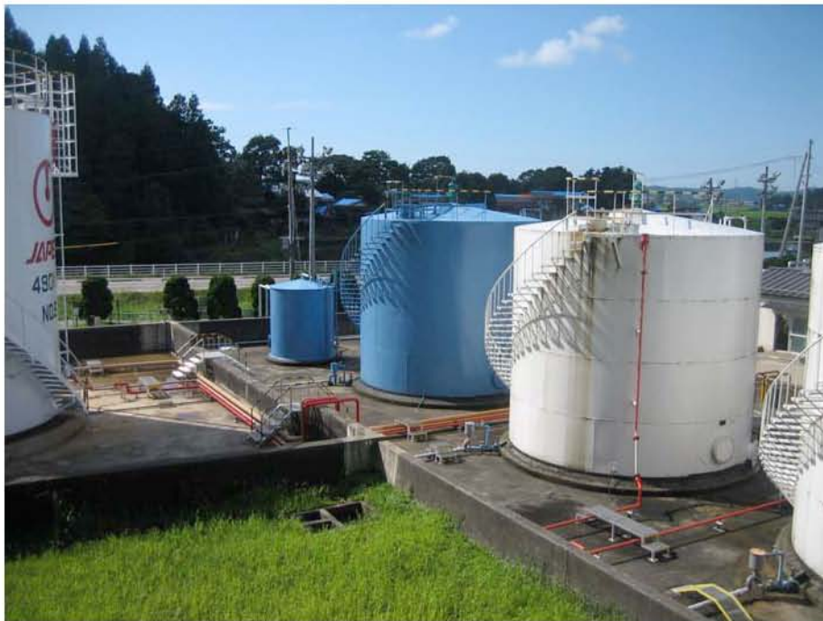
Figure 7.12: Oil storage tanks (Site RK55, N37.38917° E138.63377°, photos taken 7/23/07 12:30). No damage was observed at this site.
