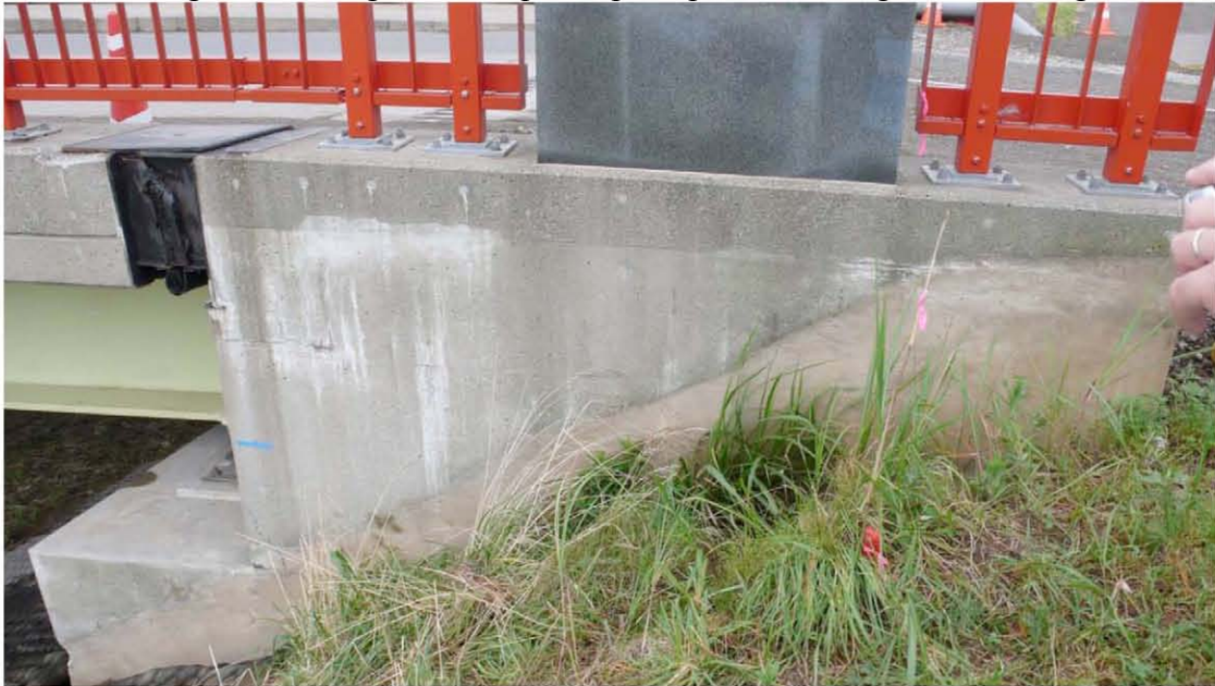
Fig. 6.42 The soil around the south abutment moved towards the river during the earthquake.
