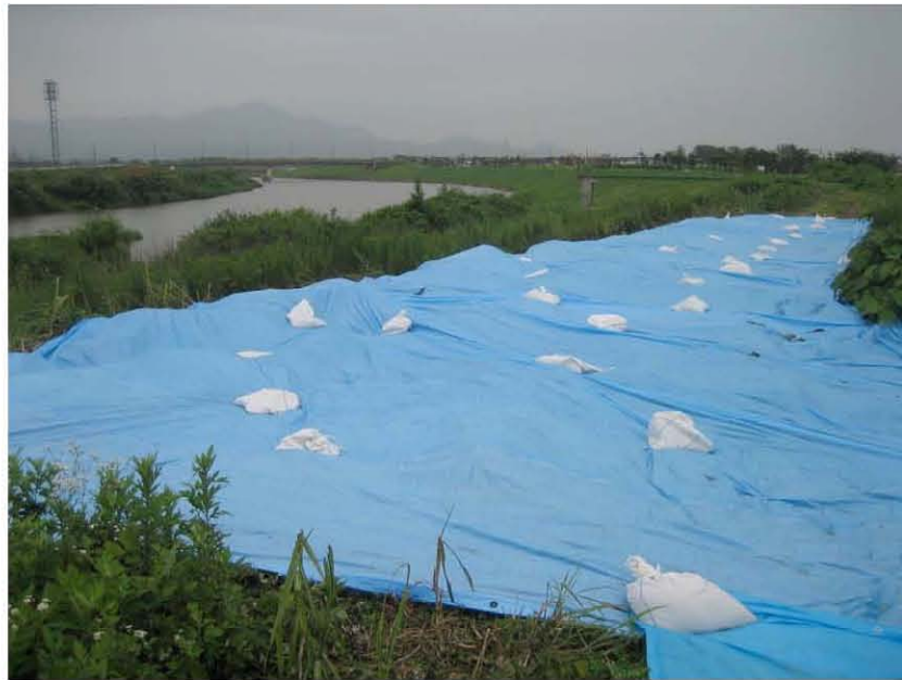
Figure 4.5: Kai-Un Bridge over Sabaishi River (Site RK4 N37.39233° E 138.58063°, 7/19/2007, 1:40 p.m.). Liquefaction induced crest cracking on the levee embankment near the northwest side of the bridge.
