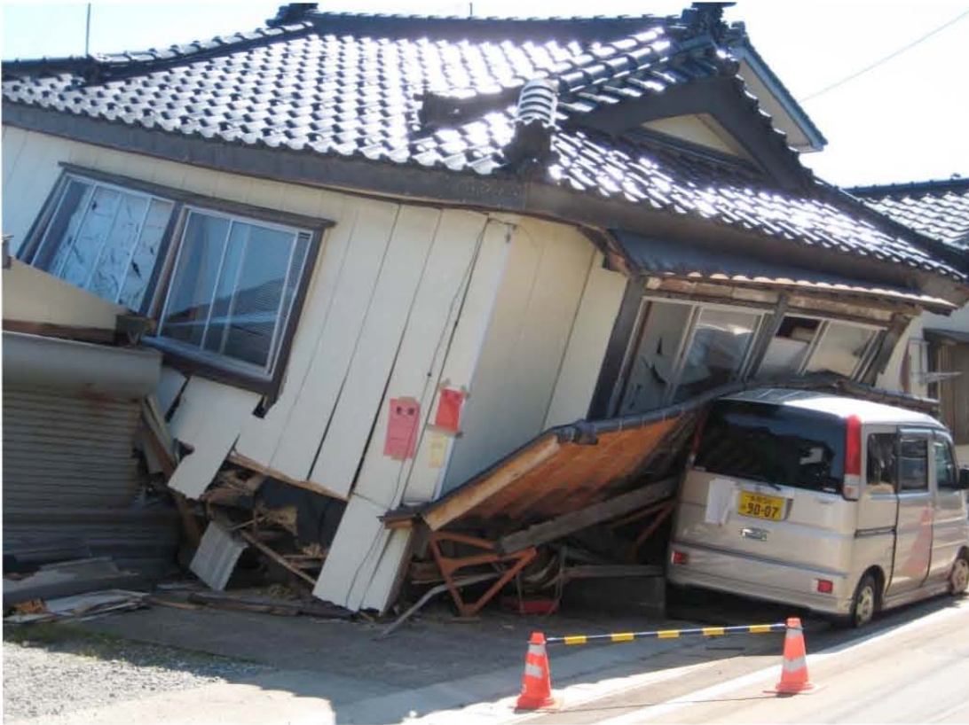
Figure 5.10: Collapse of house (N37.367°, E138.567°).
