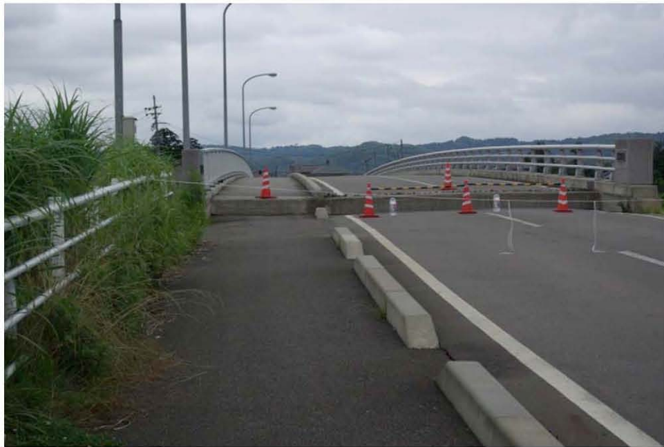
Figure 9.7: Vertical offset at approach of rural bridge that has not yet been repaired (Site SA22 N37.38439° E138.60083°, photo taken 7/21/07 15:00).
