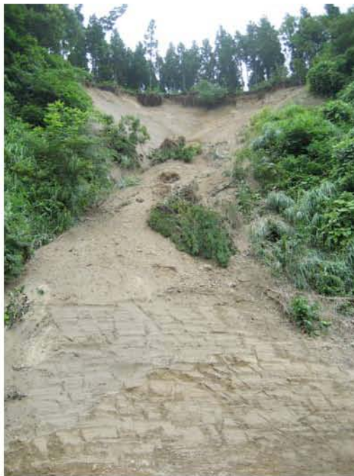
Figure 3.7: Ozumi-Mishimayamachi Landslides (Site RK2/YT2; N37.44057° E138.70467°, photos taken 7/20/07 at approximately 11:30). These slides occurred on a native hill slope and consisted of debris slumps in mudstone/siltstones and colluvium materials. High-resolution, topographic data was collected of these landslides using the terrestrial LiDAR scanning method.
