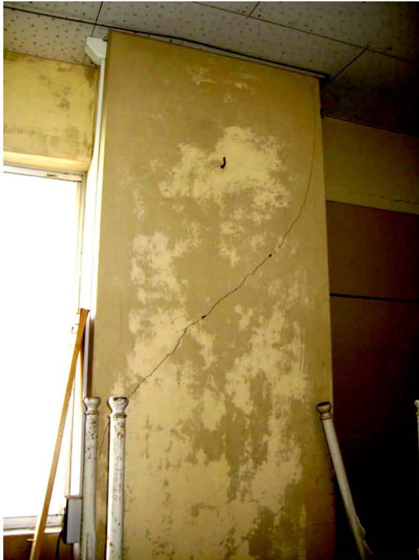
Figure 5.21: Column in first story of The Kashiwazaki High School, cross section and observed crack pattern (Site SP11, N37.3721°, E138.5569°).
