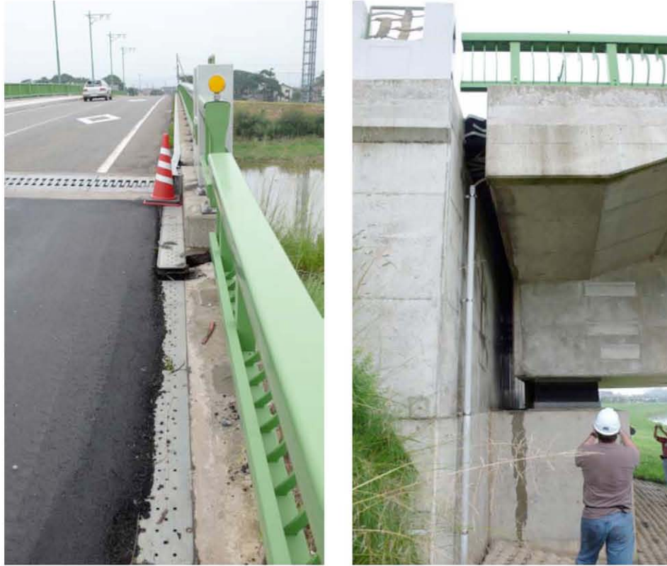
Fig. 6.37. Signs of movement of the abutments included distortion of bearings.
