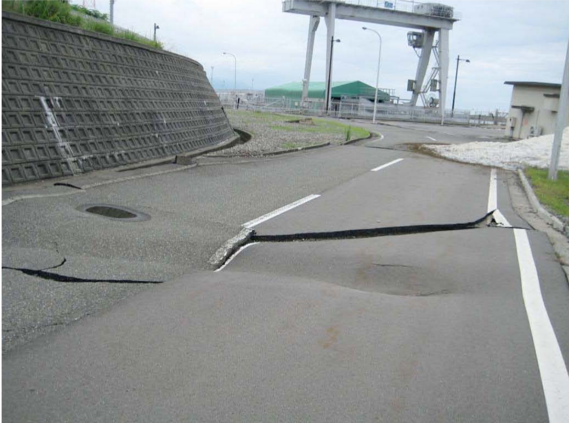
Figure 5.3: Damaged road at power plant.
