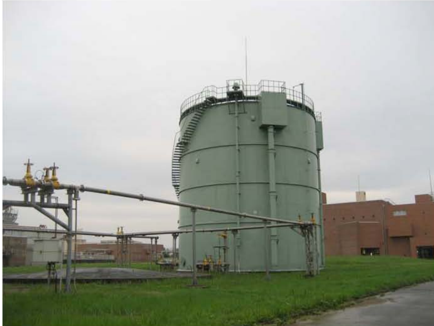
Figure 7.1: Steel tank at the Ansei-Chou waste water treatment plant (Site RK9, N37.38748°, E138.56587°, photo taken 7/20/07 16:40). Sand boils and slight overturning of the support member to the far-most right of the photograph were observed, as was extensive lateral spreading and road damage. Indications of minor distress of the tank was identified but for the most part appeared in good service.
