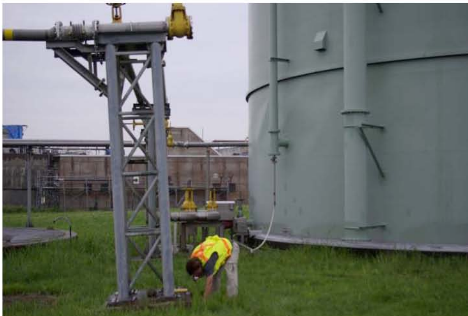
Figure 7.2: Steel tank at the Ansei-Chou waste water treatment plant (Site RK9, N37.38748°, E138.56587°, photo taken 7/20/07 16:40). Minor distress to the wall was observed roughly 3 m above the base of the tank.
