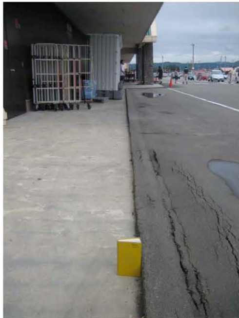
Figure 4.38: Plant 5 Store - Ground settlement in dune sand was observed around the building and an underground storage tank had been uplifted (Site RK41, N37.41468° E138.60840°, 7/22/2007).
