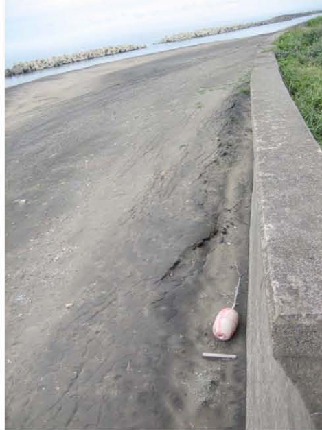
Figure 8.41: Evidence of minor liquefaction and lateral spreading in sandy beach deposits adjacent to the seawall (Site RK37, N37.45478°, E138.60927°, photo taken 7/23/07).
