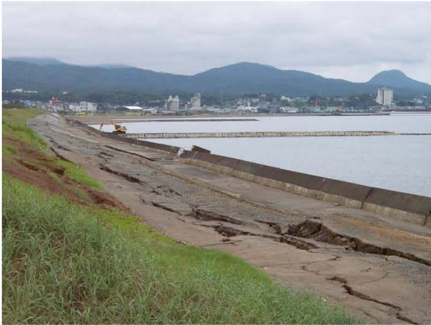
Figure 8.38: Ground deformations adjacent to the embankment and seawall (Location is southwest of Site SD1, photo taken 7/22/07 11:42).
