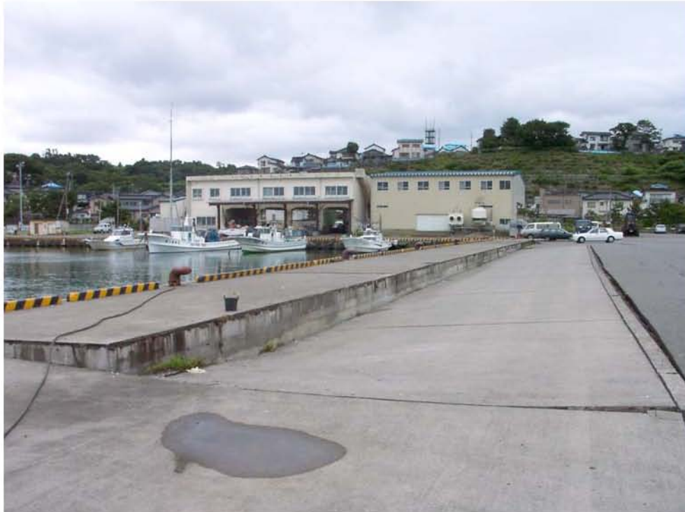
Figure 8.18: Kashiwazaki Port - East facing portion of the “Southwestern Pier” showing pronounced ground settlement (Site SD5, N37.36532° E138.53213°, photo taken 7/22/07 14:05).
