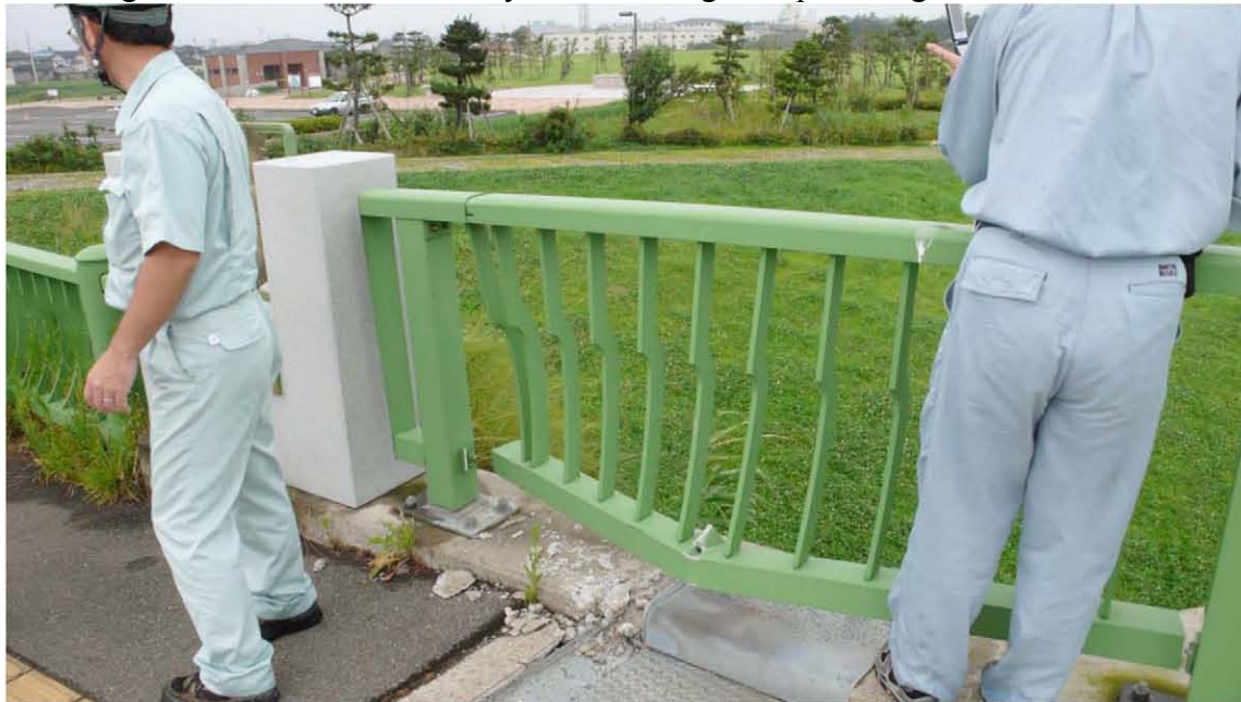
Fig. 6.38. Pounding between abutment and wingwall.
