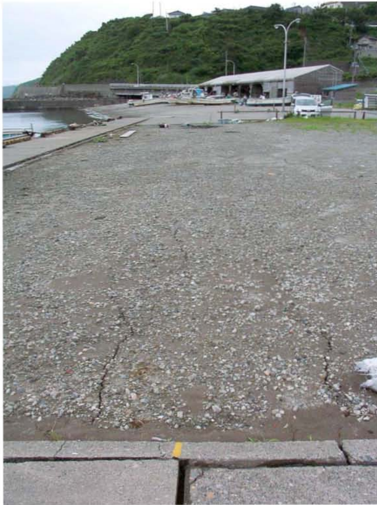
Figure 8.1: Minor ground failure along the waterfront at Kasashima (Site RK21, N37.33702° E138.46680°, photo taken 7/21/07 14:49). The limited extent of the ground cracking indicated incipient lateral movement.
