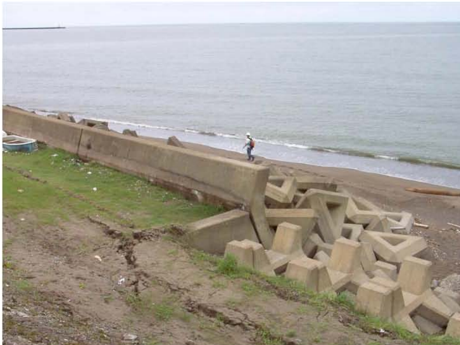
Figure 8.32: Eastern end of the seawall located adjacent to the damaged cement plant and mouth of the Sabaishi River (Site SD1, approximately N37.38868° E138.56413°, photo taken 7/22/07 10:56). Lateral spreading behind the wave armor units, as well as ground settlement and minor sea wall damage was widespread.
