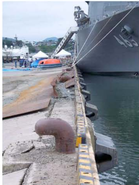
Figure 8.26: Kashiwazaki Port - Evidence of more extensive lateral caisson displacement and ground settlement adjacent to the quay wall located along the eastern end of the north face of the terminal (Site SD8, approximately N37.36680° E138.53825°, photo taken 7/22/07 15:36).
