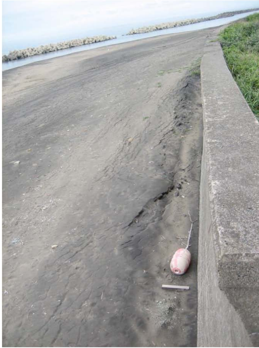
Figure 4.32: Lateral spreading related ground cracking in front of seawall. (Site RK37, N37.45478° E138.60927°, 7/22/2007).
