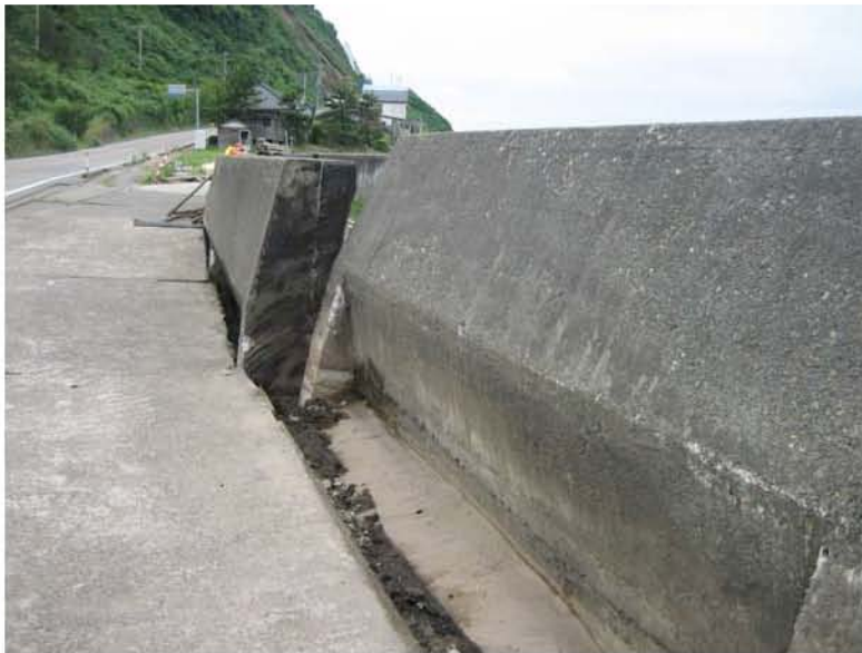
Figure 4.29: Liquefaction of beach sand led to lateral spreading of a road embankment and both rotation and translation of a 30-meter-long segment of concrete seawall. (Site RK35, N37.48497° E138.62645°, 7/22/2007). Deformations were on the order of 25 cm vertical, and up to 64 cm horizontal, with a component of rotation as measured by 32 cm lateral deformation at the base of wall and 64 cm lateral deformation at 2 m height of wall.
