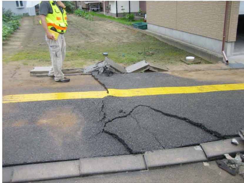
Figure 4.7: Kai-Un Bridge area Sabaishi River (Site RK4 N37.39233° E138.58063°, 7/19/2007, 1:40 p.m.). A sub-linear zone of lateral spreading, sand boils and settlement that may be associated with a buried shoestring sand deposit from the former channel of the Sabaishi River resulted in damage in the neighborhood immediately south of the Kai-Un Bridge.
