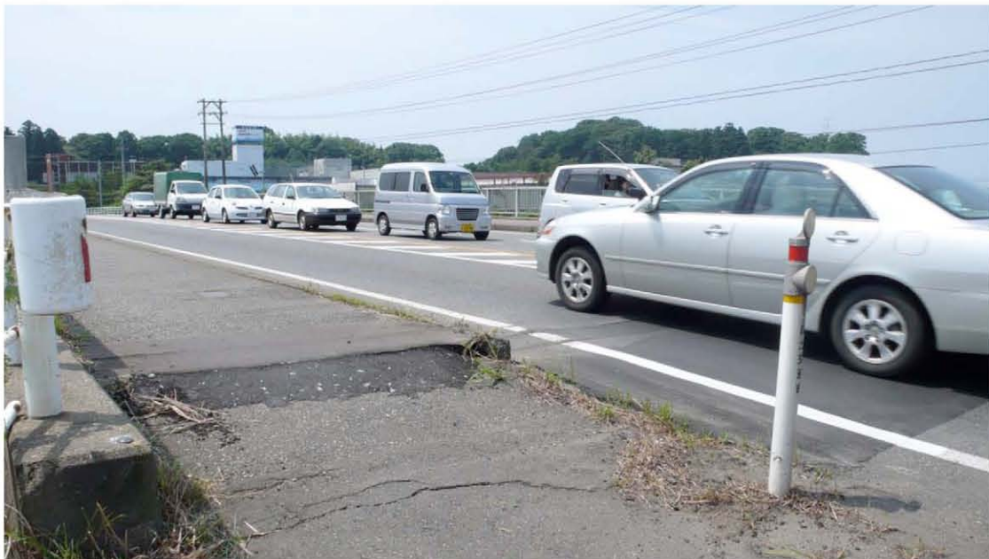
Fig. 6.19. Slight (10cm) settlement at bridge approaches.
