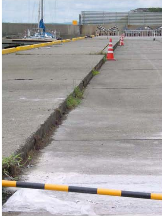
Figure 8.5: Kashiwazaki Marina - Evidence of minor settlement behind quay walls (Site SD3, N37.36093° E138.52027°, photo taken 7/22/07 13:12).
