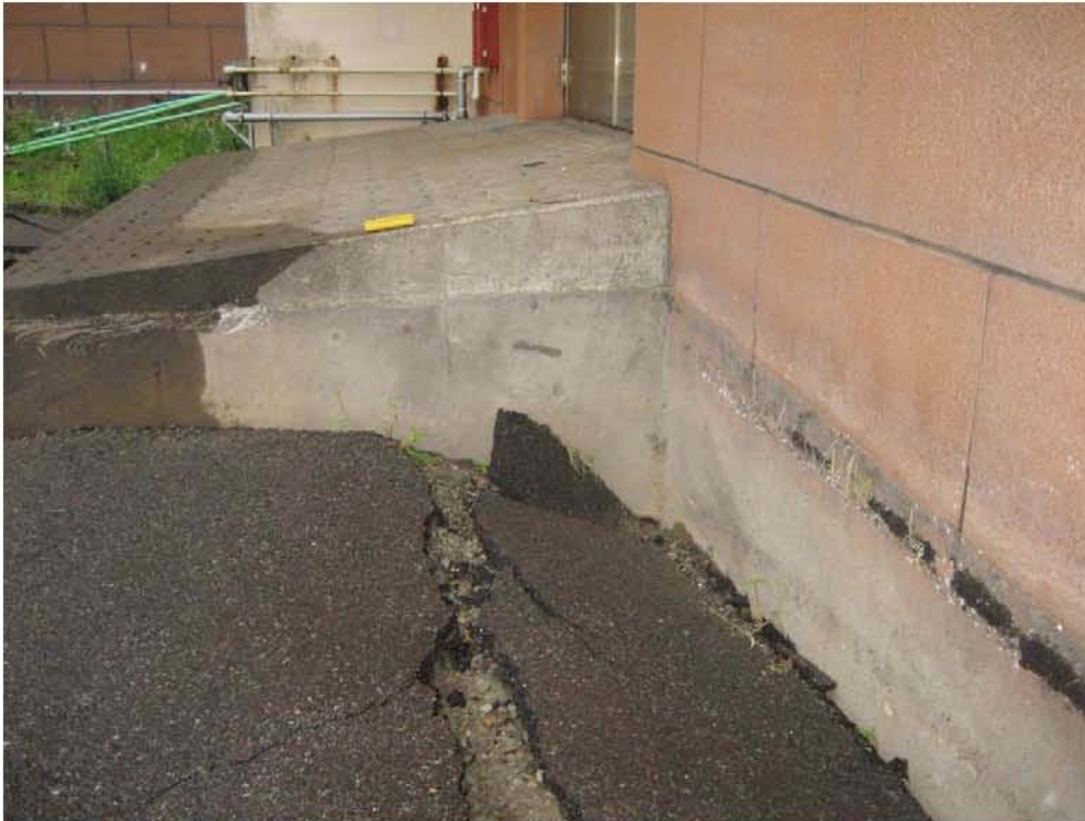
Figure 4.15: Kashiwazaki Wastewater Treatment Plant on the south side of Sabaishi River near the Sea of Japan (Site RK9 N37.38748° E138.56587°, 7/19/2007). Damage to the main building from liquefaction of ground resulted in meter-scale ground settlements.
