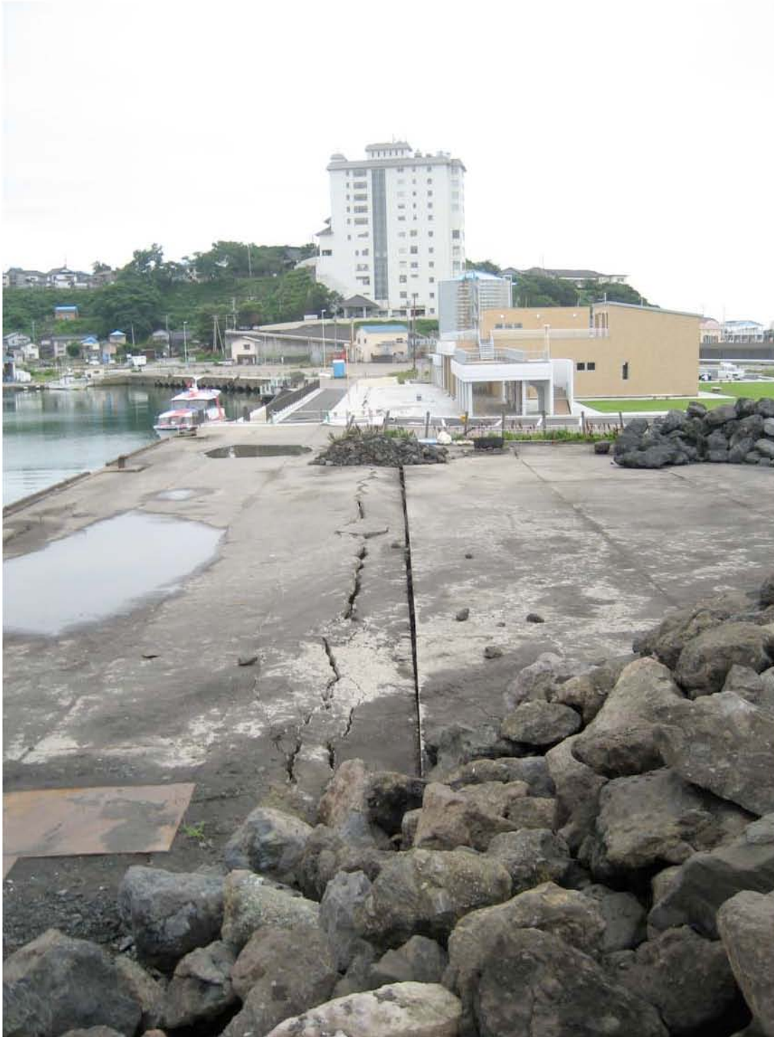
Figure 4.24: Kashiwazaki Harbor - South area experienced ground damage from liquefaction-induced lateral spreading and settlement, here seen from a mound of riprap (Site RK25, N37.36713° E138.53210°, 7/20/2007).
