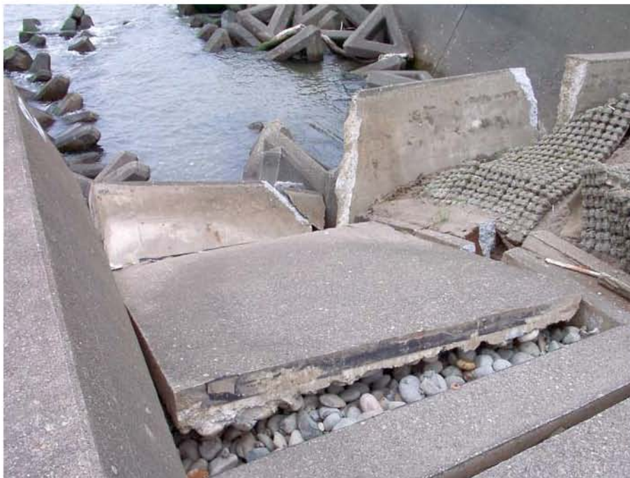
Figure 8.34: Close-up of the collapsed portion of the seawall showing the clean cobble backfill (Site SD1, N37.38868° E138.56413°, photo taken 7/22/07 11:23).
