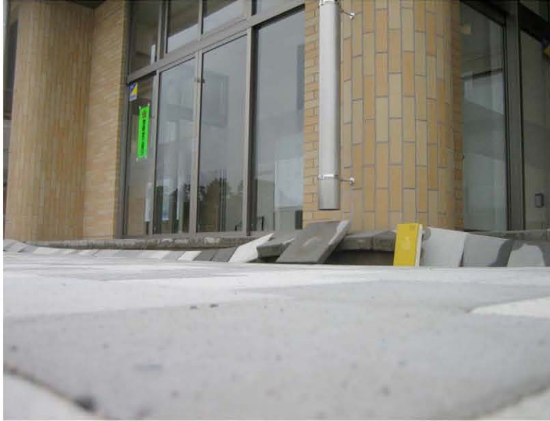
Figure 4.22: Kashiwazaki Harbor - The southern area experienced ground damage from liquefaction-induced lateral spreading and settlement. We observed settlement immediately adjacent to the pile supported port office building. (Site RK25, N37.36713° E138.53210°, 7/20/2007).
