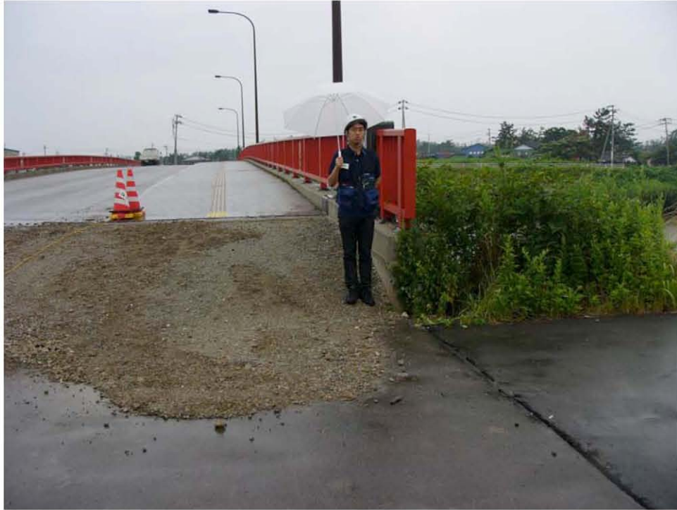
Figure 9.6: Vertical offset at the approach of Kai-Un Bridge that has been temporarily repaired with gravel fill to permit access (Site YT3, N37.39232° E138.58063°, photo taken 7/20/07 12:42). A vertical offset of 33 cm was measured at the adjacent abutment (left of this photo).
