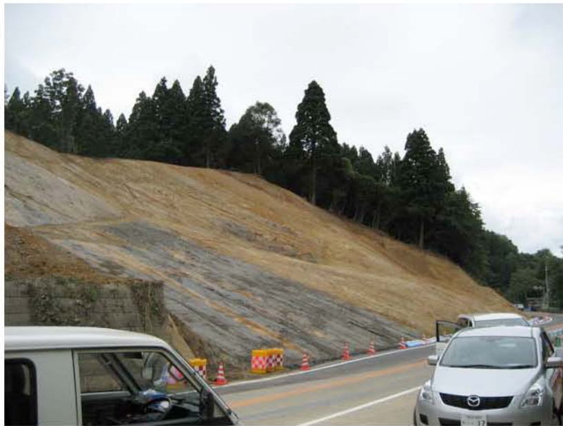
Figure 3.6: Ozumi Senbon Landslide at Highway 8 north of intersection with Route 252 (Site RK1/YT1; N37.41422° E138.71347°, photos taken 7/20/07 10:24 (top) and 7/23/07 13:04 (bottom)). This slide is approximately 150 meter wide, 100 meters long and 10 meters deep. According to construction personnel at the site during the reconnaissance, the slide plane occurred near the colluvial/bedrock interface, at a depth of between 6 and 11 meters. Signs of rotational movement were noted from back-rotated guardrails at the toe of the slide. This landslide forced closure of both lanes of traffic along Highway 8, just north of the intersection with Route 252, however both lanes had been reopened as early as 8 days following of the earthquake when reconnaissance team members revisited the site. Bottom photo shows excavated slide and subsurface bedrock lithology and structure.
