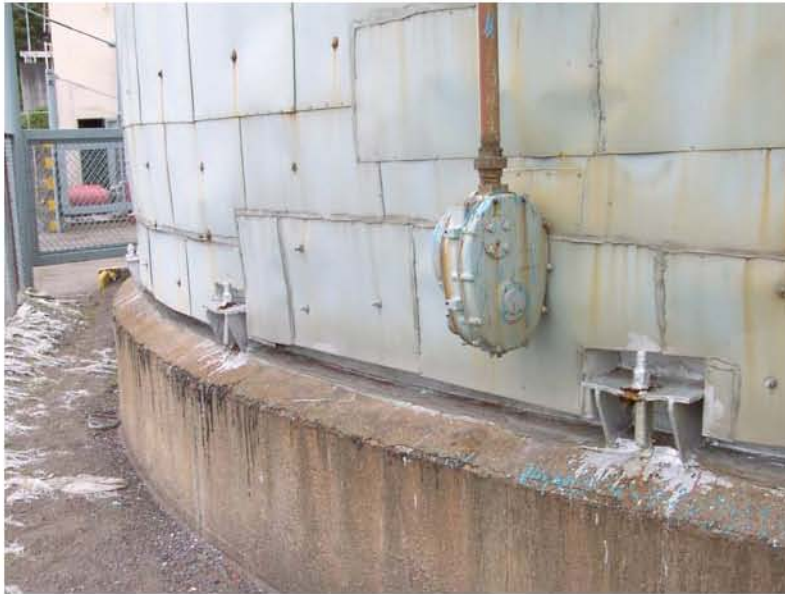
Figure 7.7: Kashiwazaki Port - Anchorage of asphalt storage tank (Located near Site RK25, N37.36713° E138.53210°, photo taken 7/22/07 12:37).
