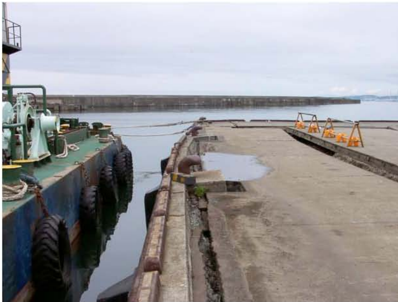
Figure 8.17: Kashiwazaki Port - West facing portion of the “Southwestern Pier” showing displacement of the sheetpile wall and ground settlement due to liquefaction of sandy backfill (Site SD5, N37.36532° E138.53213°, photo taken 7/22/07 13:58).
