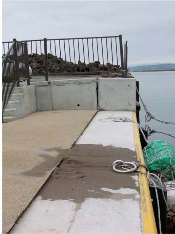
Figure 8.12: Kashiwazaki Port - Liquefaction-induced damage to the sightseeing wharf with minor displacement of the caisson quay wall (Site RK25/SA25/YT4, N37.36713° E138.53210°, photo taken 7/21/07 16:09).
