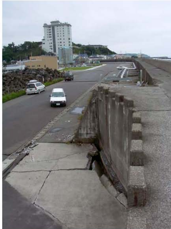
Figure 8.14: Kashiwazaki Port - Evidence of ground failure adjacent to the seawall at the outer quay wall area (Located near site RK25/SA25/YT4, N37.36713° E138.53210°, photo taken 7/21/07 15:50).
