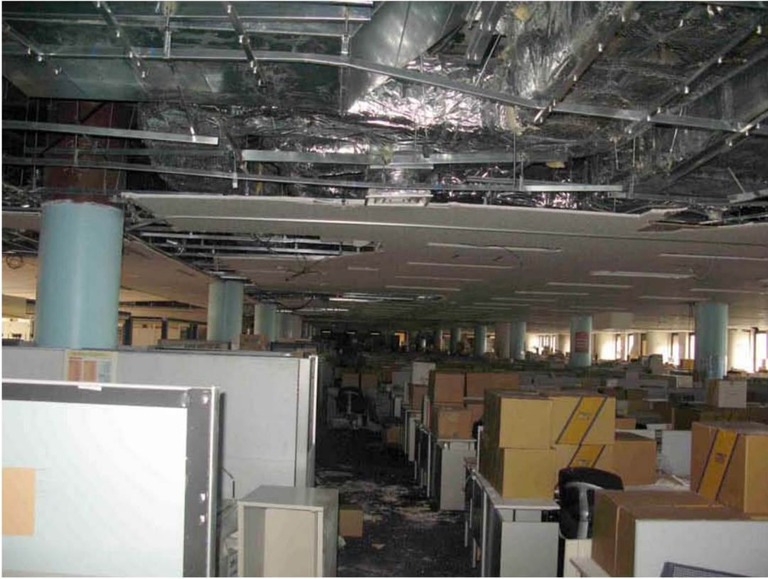
Figure 5.7: Ceiling damage in administration building of nuclear power plant.
