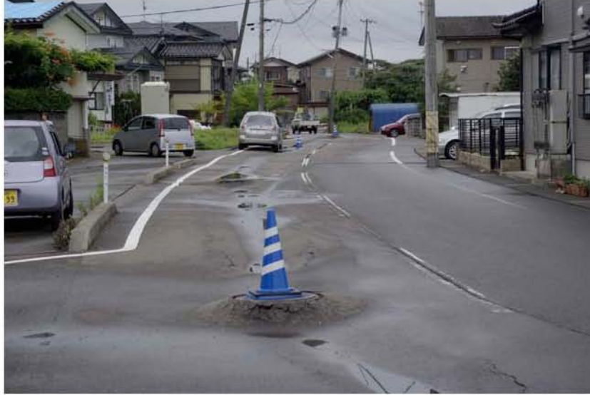
Figure 10.1: Example of an elevated manhole caused by settlement of road fill. The depression caused by densification of lightly compacted trench backfill during cyclic loading was evident along extensive sections of the roadway. This area was conspicuous for pipe breaks associated with ground deformation (Site SD11, N37.36650° E138.58868°, photo taken 7/23/07).
