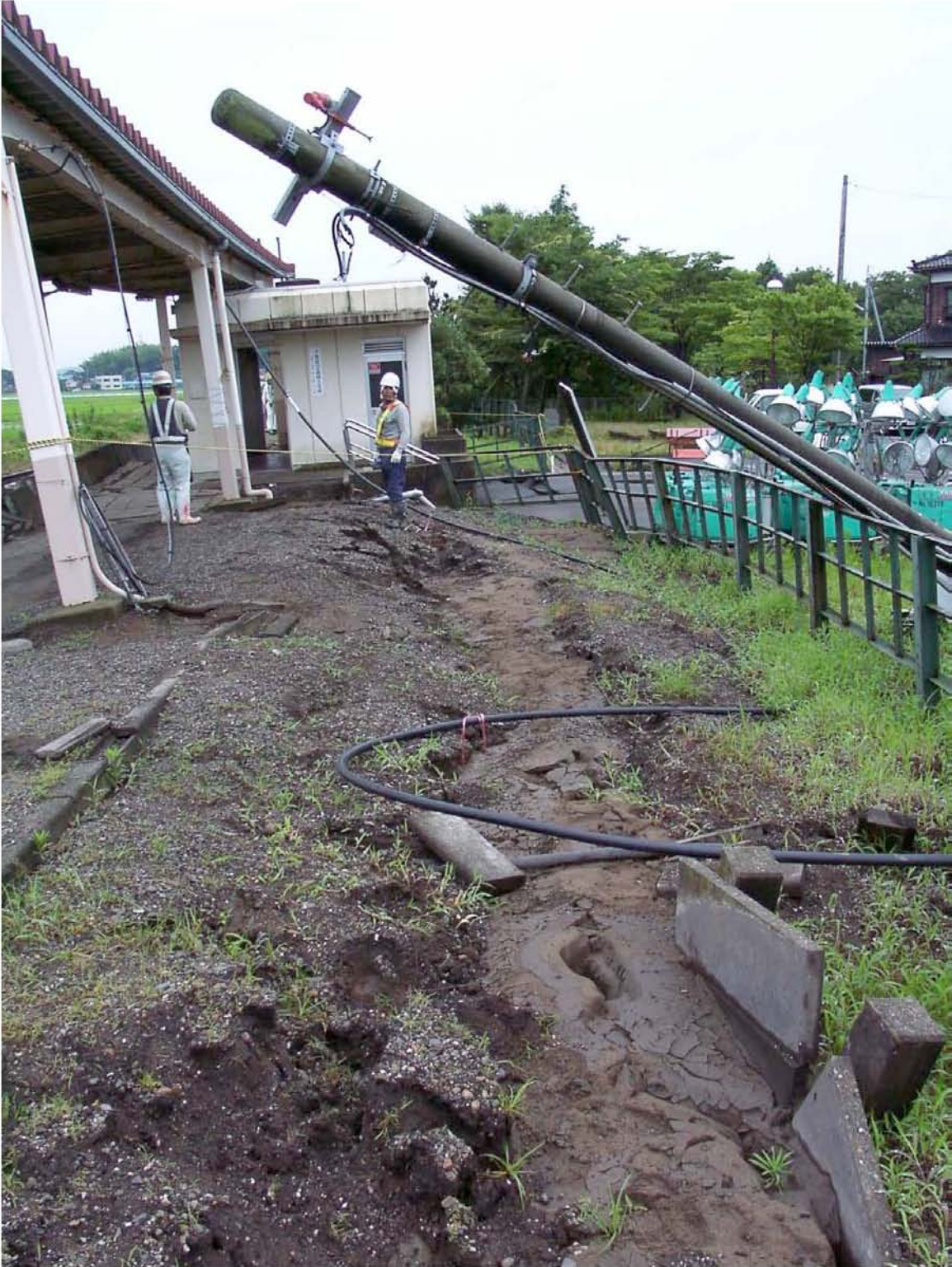
Figure 9.11: Liquefaction-induced damage at Arahama Station (Site RK13, N37.40555° E138.60197°, 7/21/07 09:42).
