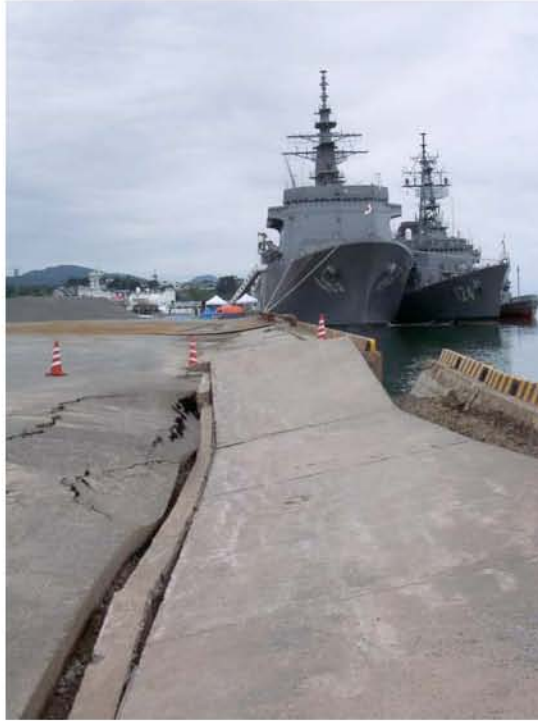
Figure 8.27: Kashiwazaki Port - Significant liquefaction-related damage to the quay walls located at the eastern edge of the terminal adjacent to the mouth of the U River (Site SD8, approximately N37.36680° E138.53825°, photo taken 7/22/07 15:32).
