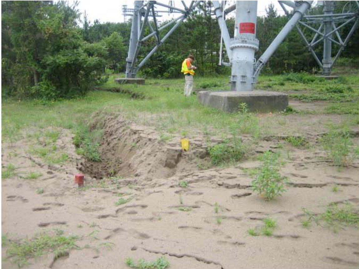
Figure 4.33: Liquefaction and lateral spread of ground adjacent to High Voltage Transmission Line Tower (Site RK40, N37.41633° E138.60792°, 7/22/2007).
