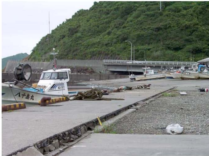
Figure 8.3: Kasashima Harbor - Settlement of fill behind quay walls (Site RK21, N37.33702° E138.46680°, photo taken 7/21/07 14:48).
