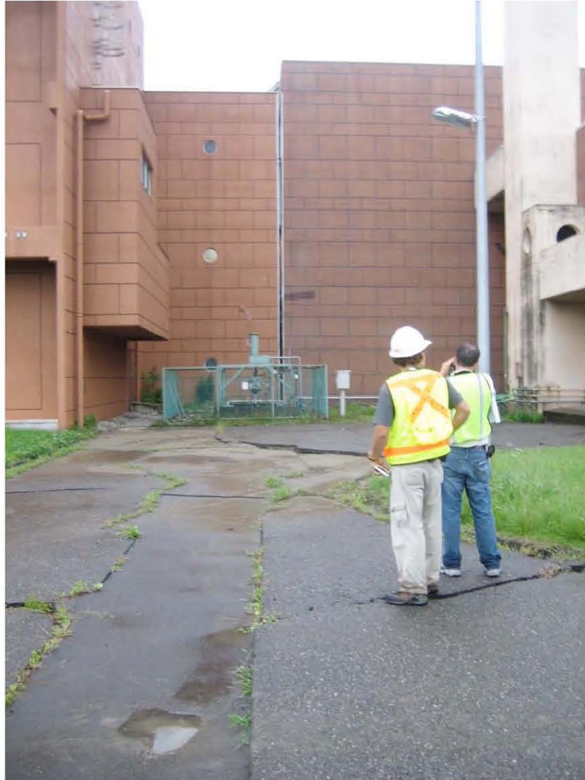
Figure 4.16a: Kashiwazaki Wastewater Treatment Plan on the south side of Sabaishi River near its outlet to the Sea of Japan (Site RK9 N37.38748° E138.56587°, 7/19/2007). Damage to the main building from liquefaction of ground resulted in the complete separation of two sections of the adjacent, yet integrated, three-story buildings with associated building and ground settlements.
