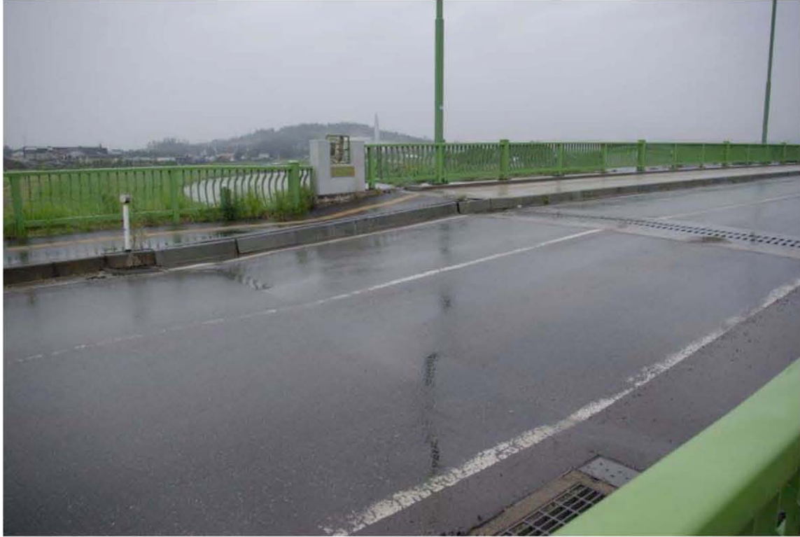
Fig. 6.39. Settlement of north bridge abutment.
