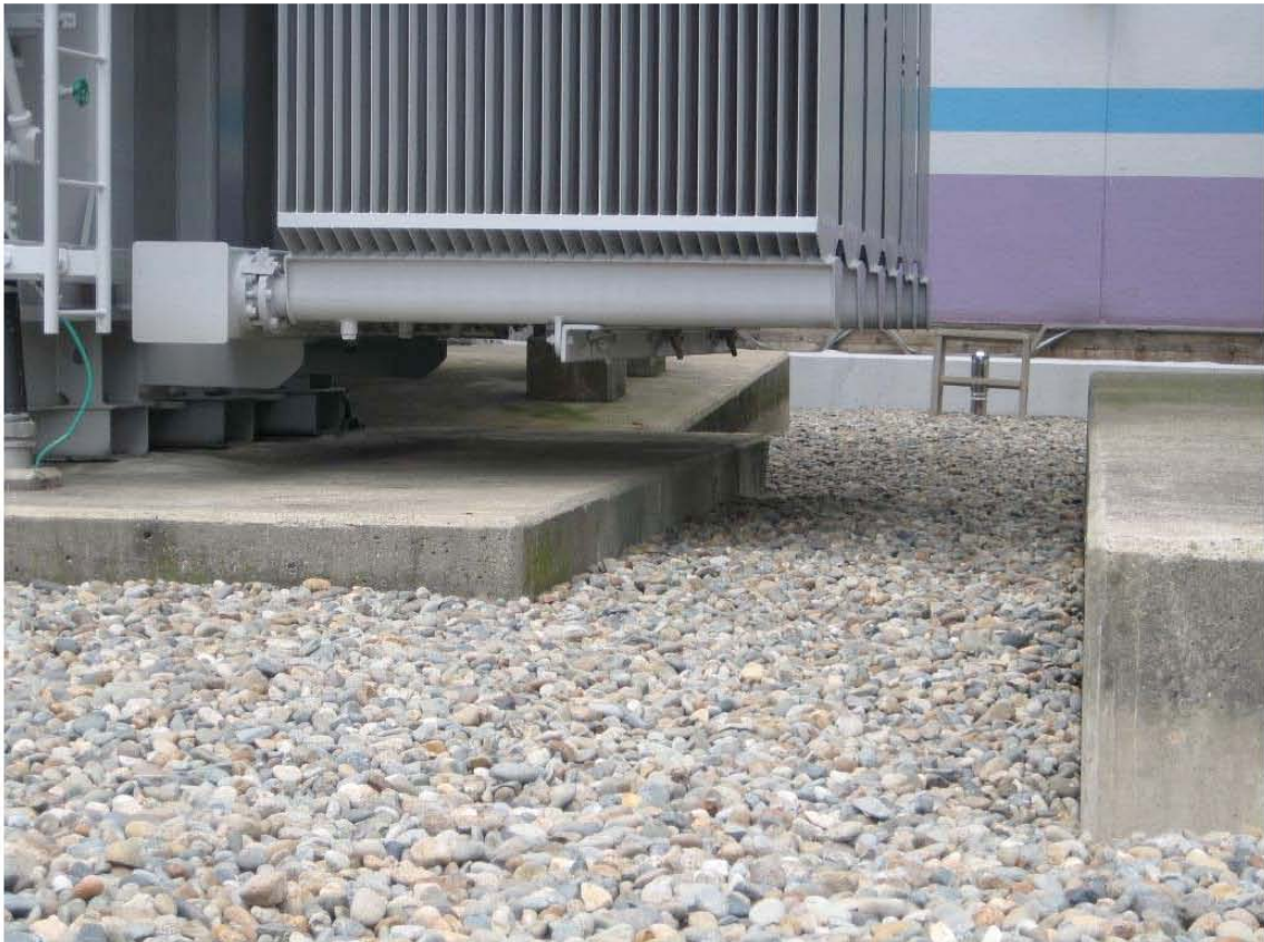
Figure 5.6: Rotation of isolated footings for equipment at nuclear power plant.
