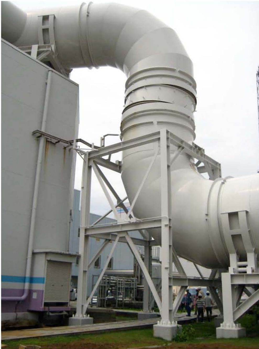
Figure 5.5: Failure of joint in exhaust pipe.
