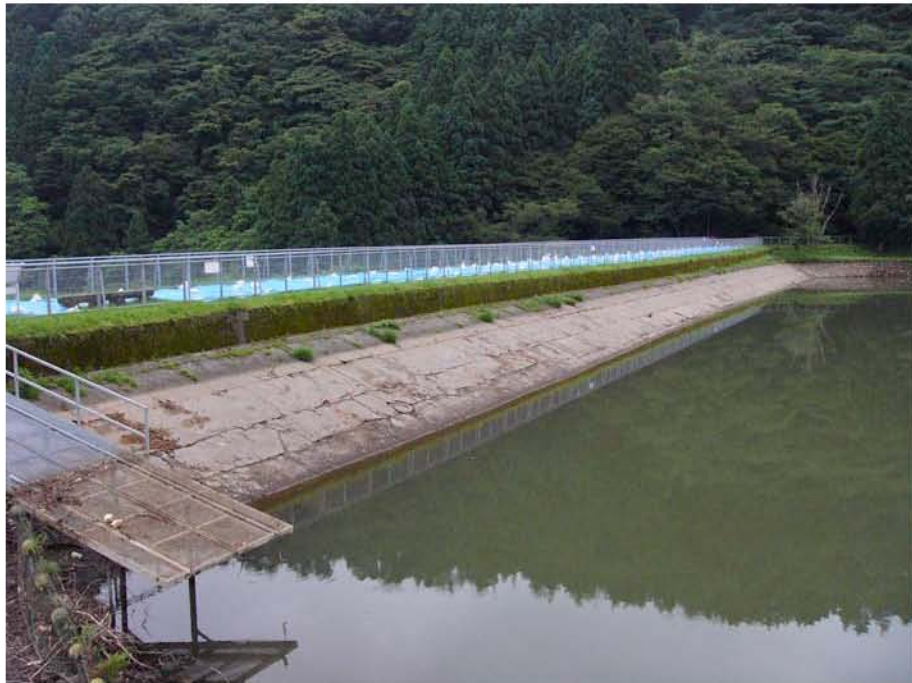
Figure 3.10: Embankment cracking at the crest of Kawauchi Dam, constructed in 1938. (Site YT19; N37.33635° E138.52410°, photos taken 7/21/07 at approximately 16:20).
