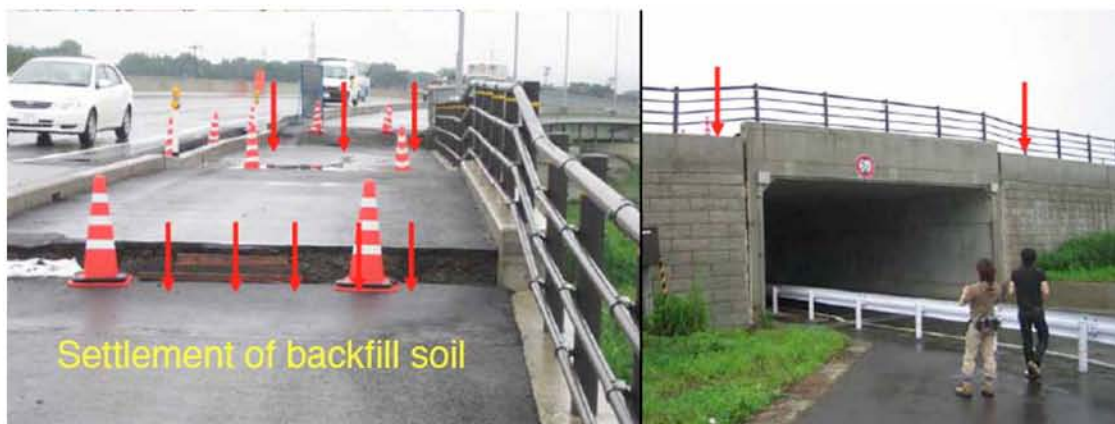
Fig. 6.13. Settlement of west embankment (courtesy G. Watanabe, Tokyo Institute of Technology).
