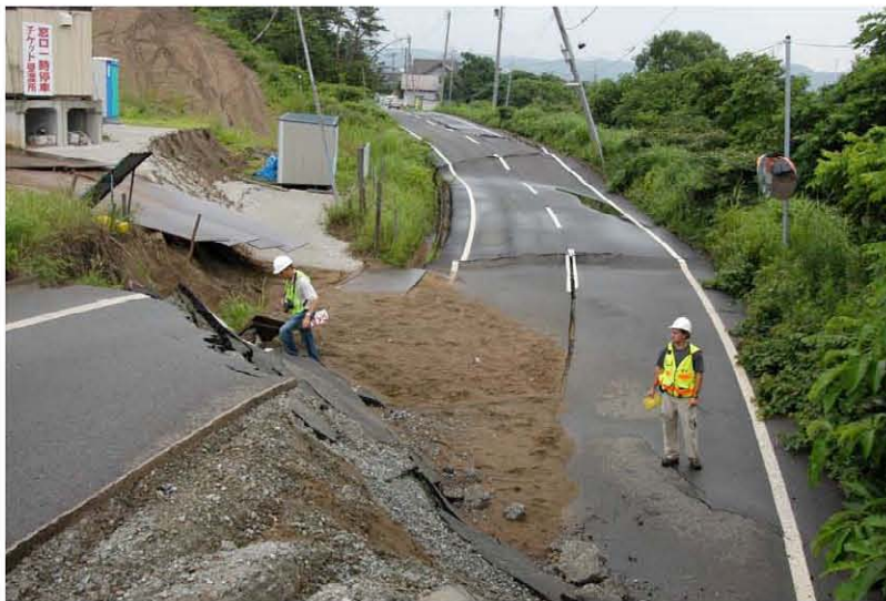
Figure 4.11: North side of Kai-Un Bridge area of the Sabaishi River - Lateral Spread on road to Kashiwazaki Municipal Incinerator (Site RK6, N37.39343° E138.58555°, 7/19/2007). A zone of lateral spreading, sand boils and settlement crossing the present-day Sabaishi River, and that may be associated with a buried shoestring sand deposit of a former channel, resulted in failure of a road on the north side of the river adjacent to the Kashiwazaki Municipal Incinerator.
