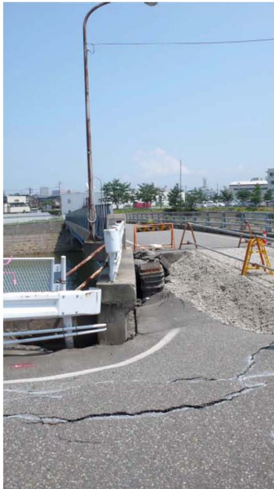
Fig. 6.62. Closer view of settlement at south abutment.
