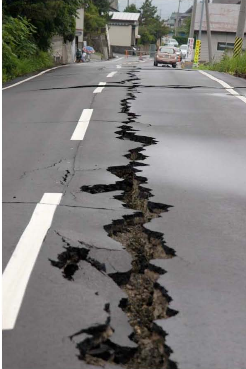
Figure 4.13: North side of Kai-Un Bridge area Sabaishi River - Lateral Spread on Road to Kashiwazaki Incinerator (Site RK6, N37.39343° E138.58555°, 7/19/2007). Lateral spreading on the north side of the river adjacent to the Kashiwazaki Municipal Incinerator damaged the access road of the facility.
