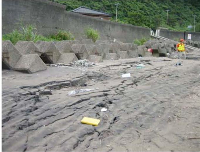
Figure 4.28: Liquefaction of beach sand resulted in lateral spreading, above, in front of a 30-meter-long segment of concrete seawall. (Site RK35, N37.48497° E138.626°, 7/22/2007)
