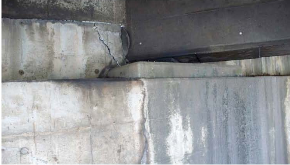
Fig. 6.52. Backwall-Diaphragm damaged by earthquake.
