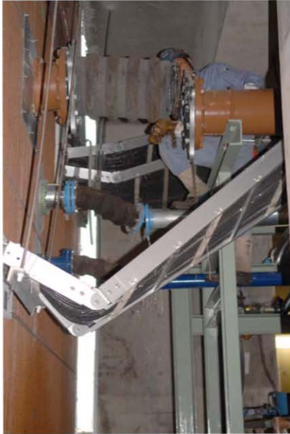
Figure 4.16b: Kashiwazaki Wastewater Treatment Plan on the south side of Sabaishi River near its outlet to the Sea of Japan (Site RK9 N37.38748° E138.56587°) Pipe breaks are due to separation of two adjacent building sections (Photo taken at 7/21/07 9:15)
