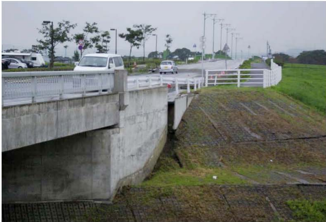
Fig 6.31. Looking southeast at Heisei bridge abutment, settled embankment, and the island.
