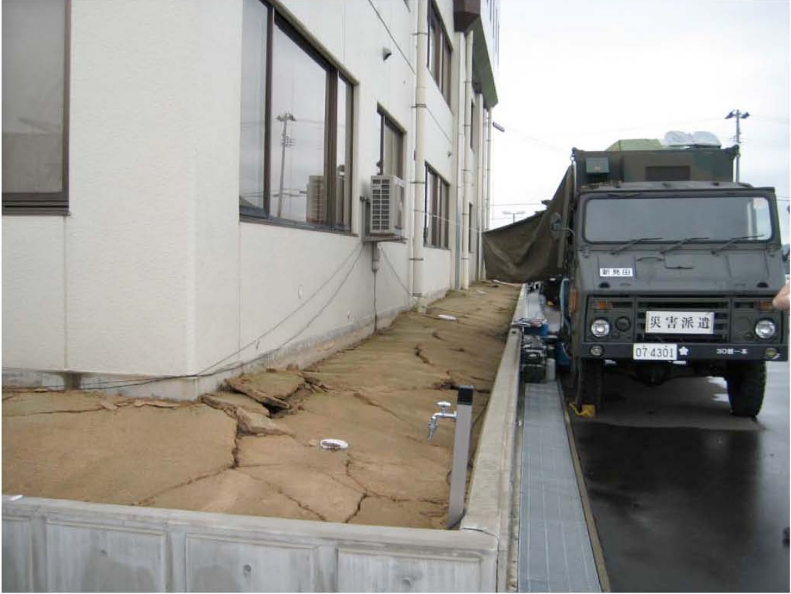
Figure 5.22: Disruption of soil surrounding a government building in Kariwa (Site SP33, N37.4223° E138.6222°).
