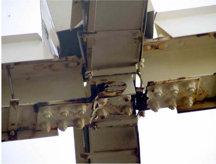
Fig. 6.26. Torn cross bracing connection on Yonahime Bridge.
