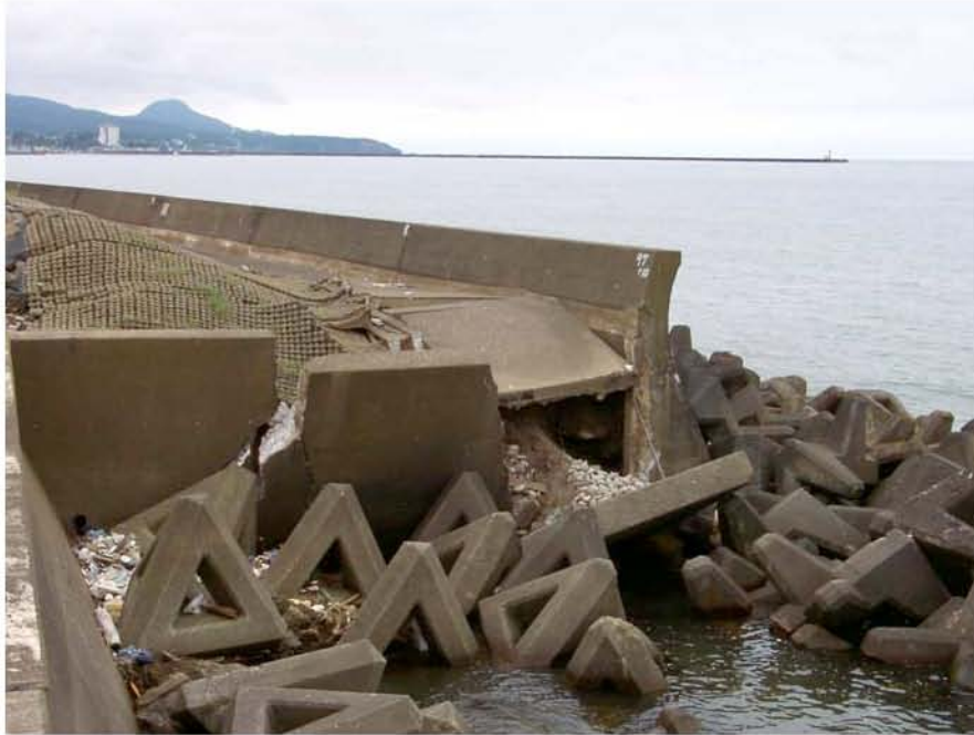
Figure 8.33: Partial collapse of a portion of the seawall located at the lateral, seaward step in alignment just west of the damaged cement plant (Site SD1, N37.38868° E138.56413°, photo taken 7/22/07 11:18).
