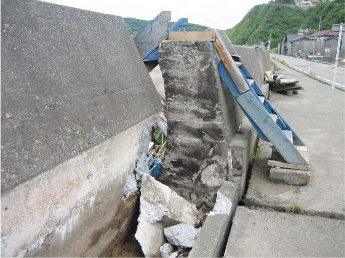
Figure 4.30: Concrete seawall deformations were on the order of 25 cm vertical (failed section up), and up to 64 cm horizontal, with a component of rotation as measured by 32 cm lateral deformation at the base of wall and 64 cm lateral deformation at 2 m height of wall. (Site RK35, N37.48497° E138.62645°, 7/22/2007).
