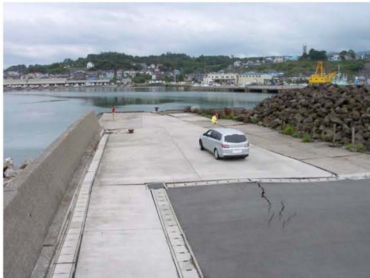
Figure 8.13: Kashiwazaki Port - Evidence of lateral ground deformation adjacent to the outer quay wall (Located near site RK25/SA25/YT4, N37.36713° E138.53210°, photo taken 7/21/07 15:49).
