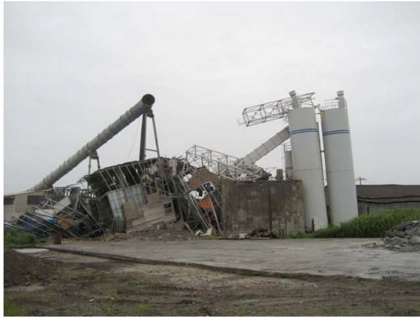
Figure 7.3: Damage to steel tanks at the cement plant located adjacent to the mouth of the Sabaishi River (Site RK10, N37.38795°, E138.56508°, photo taken 7/20/07 17:10). Tank damage likely caused by the cumulative effects of inertial loading, ground failures, and lateral loads due to the failure of appurtenant structures.
