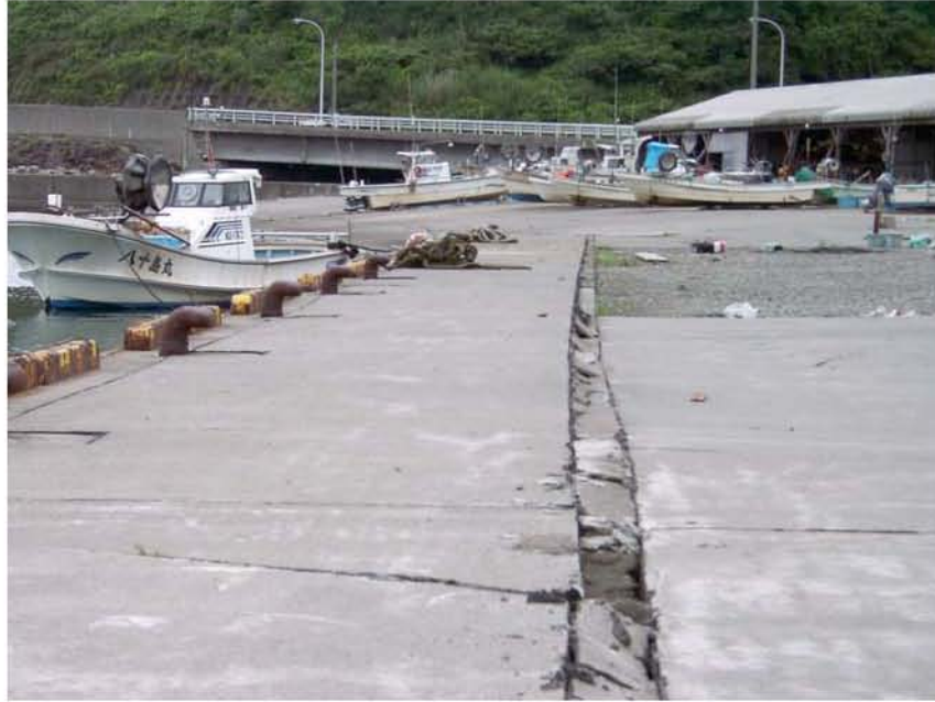
Figure 8.2: Kasashima Harbor - Ground settlement and minor lateral deformation adjacent to quay walls (Site RK21, N37.33702° E138.46680°, photo taken 7/21/07 14:40).
