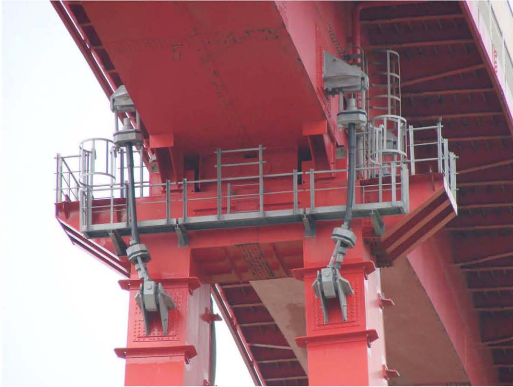
Fig. 6.22. Retrofitted bent cap at Yoneyama Bridge (courtesy of S. Unjoh, PWRI).
