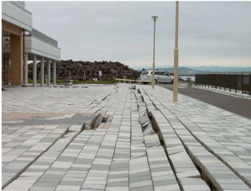
Figure 8.11: Kashiwazaki Port - Liquefaction-induced damage to the sightseeing wharf (Site RK25/SA25/YT4, N37.36713° E138.53210°, photo taken 7/21/07 16:03).
