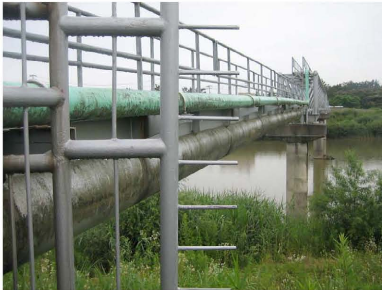
Figure 4.3: Kai-Un Bridge over Sabaishi River (Site RK4 N37.39233°, E 138.58063°, 7/19/2007, 1:40 p.m.). A water pipeline rupture was found with pipe offsets of 13 cm in the horizontal direction, 10 cm in the vertical direction, and with 40 cm of associated nearby settlement between the pipeline and the ground.
