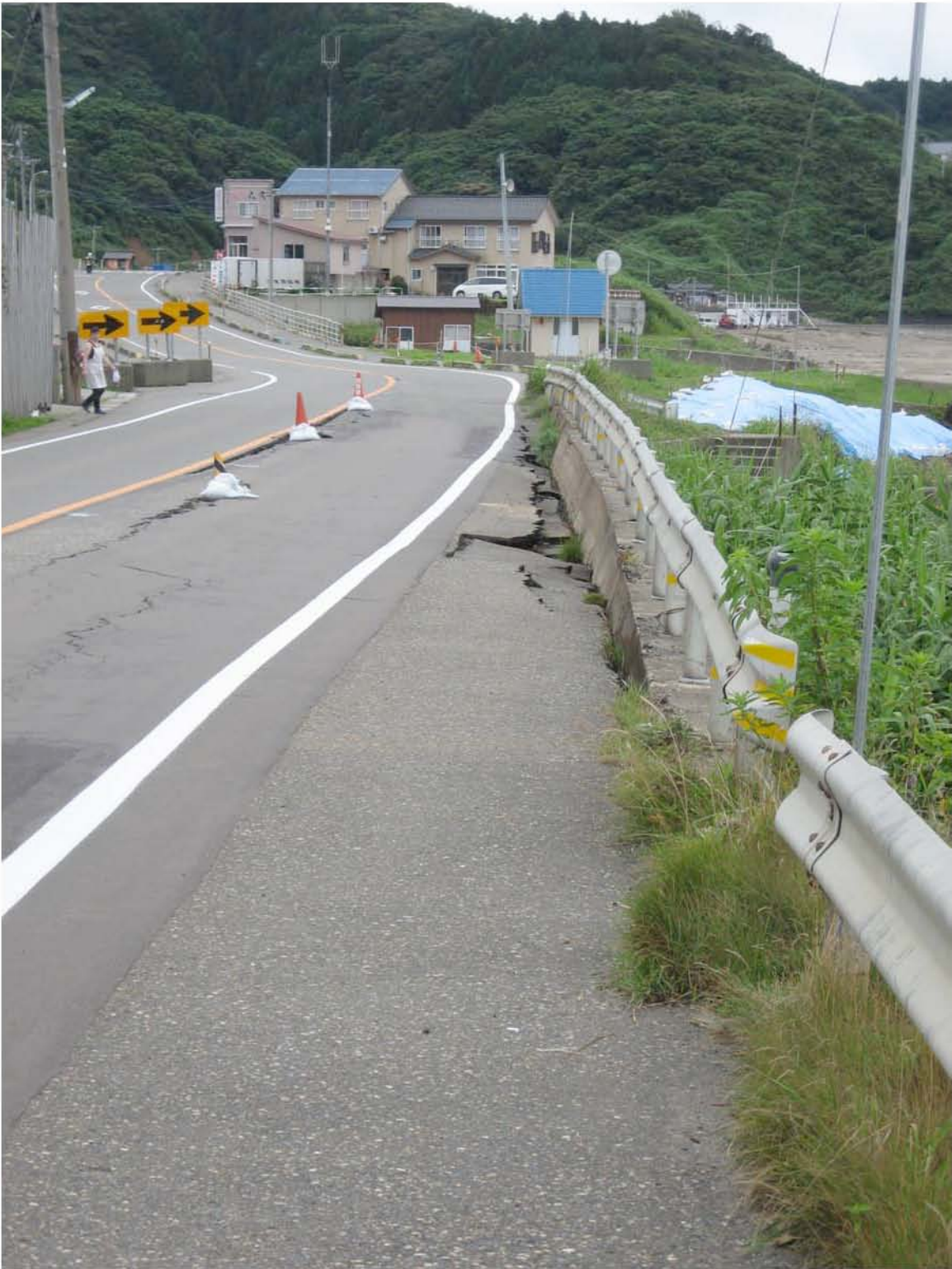
Figure 9.4: Site RK34 - Road damage from fill embankment failure on coastal road north of Kashiwazaki-Kariwa Nuclear Power Plant (Site RK34, N37.48455° E138.62435°, photo taken 7/22/07 09:56).
