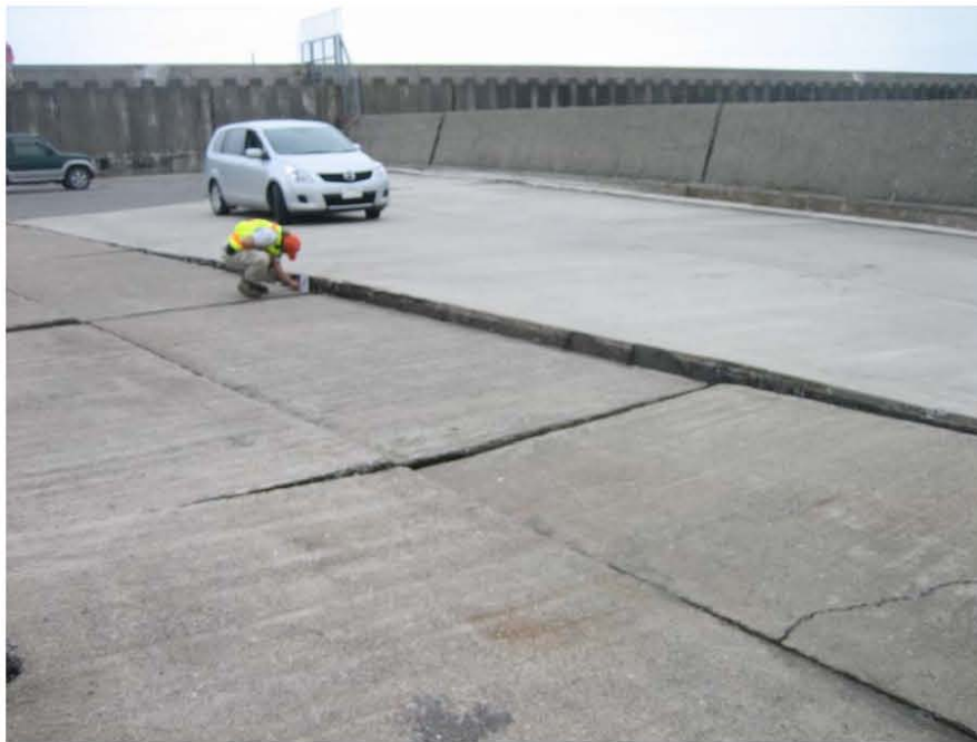
Figure 4.18: Kashiwazaki Harbor - South area experienced ground damage from liquefaction induced lateral spreading and settlement of separated pier slab sections (Site RK25, N37.36713° E138.53210°, 7/20/2007).
