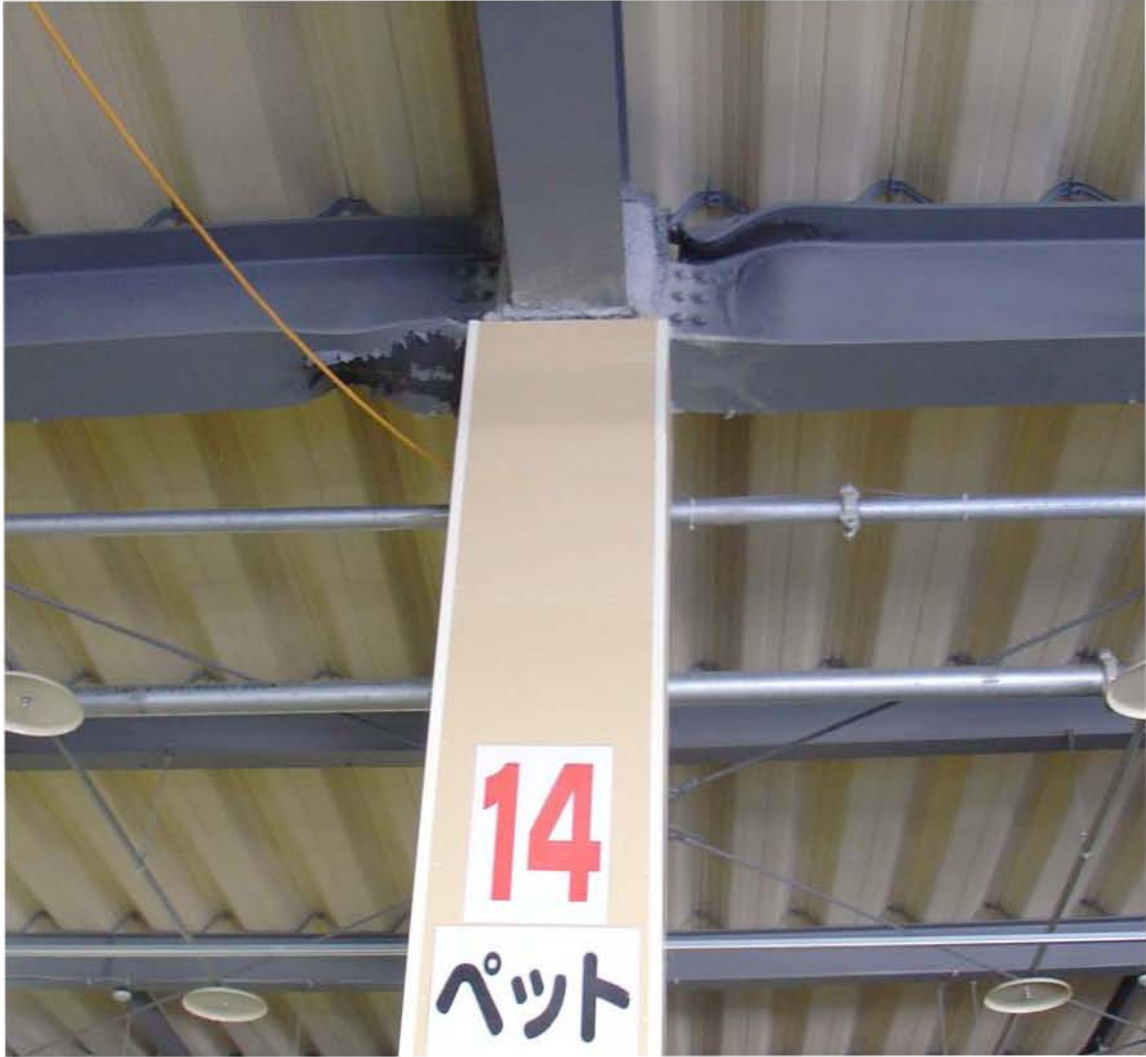
Figure 5.15: Buckling of beam flanges (Site RK41, N37.41472° E138.60833°, photo by Peter Yanev).
