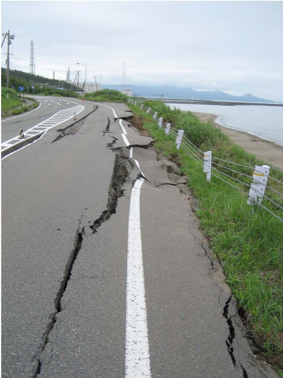
Figure 9.3: Road damage from fill embankment failure on coastal road north of Kashiwazaki Nuclear Power Station (Site RK38, N37.44927° E138.60572°, photo taken 7/22/07 13:04). Such damage tended to increase with distance toward the epicenter, often requiring traffic controls to guide cars across the one open lane.
