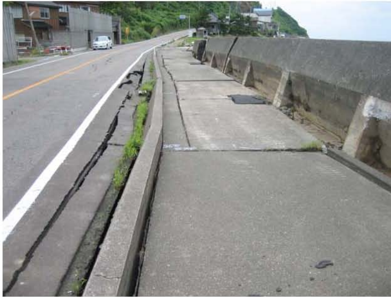
Figure 8.43: Liquefaction-induced damage to the seawall and adjacent roadway (Site RK35, N37.48497°, E138.62645°, photo taken 7/23/07).
