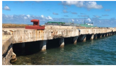
Deterioration of a wharf
