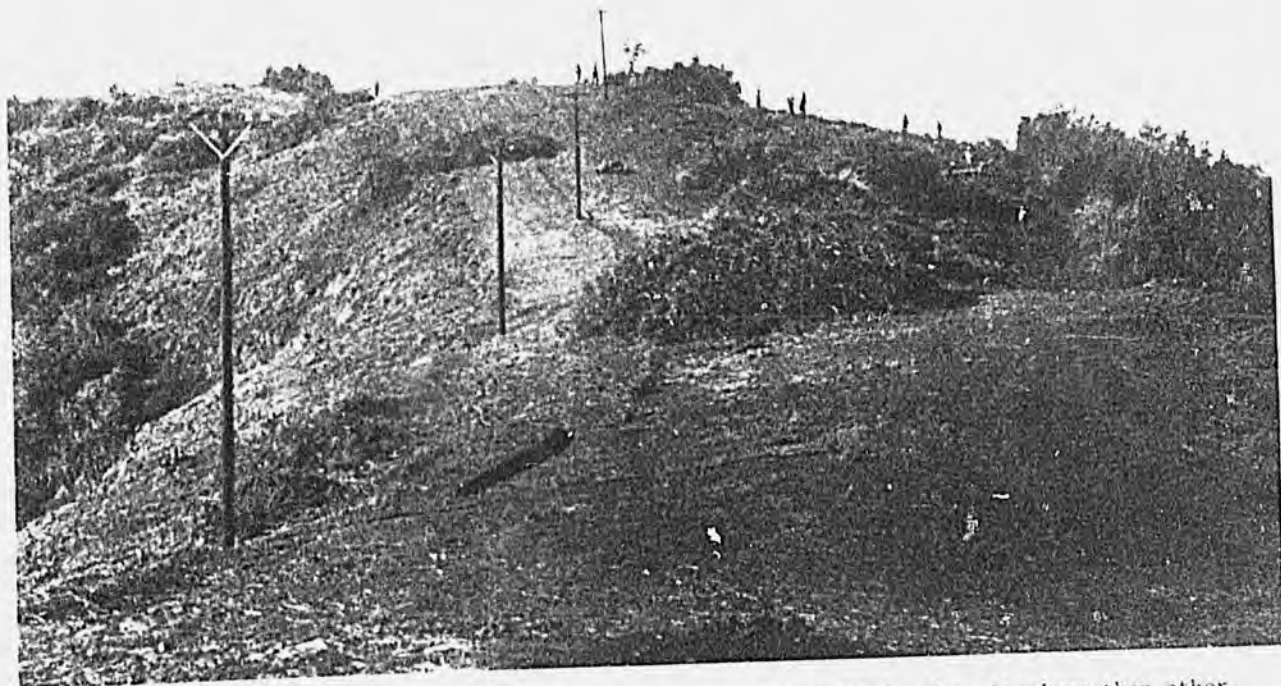
Figure 2--Hand cutting and piling of brush is expensive, but disturbs the site less than other clearing methods.
