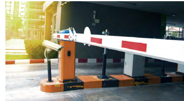
Vehicle Access Control
