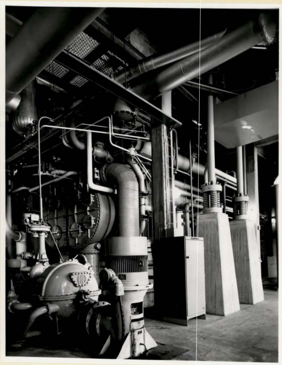
Photograph 3. Turbine condenser with cooling-water pump and filter.
