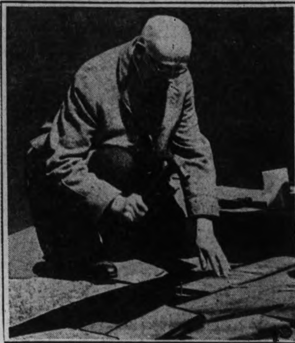
OLD TIRES MAKE STREETS. —Rubber paving blocks, made from auto tires, are being tried out in Boston streets. They are said to take the noise out of traffic and to wear better than many paving materials. John A. Rourke, a Boston city official, is shown laying the first blocks.
