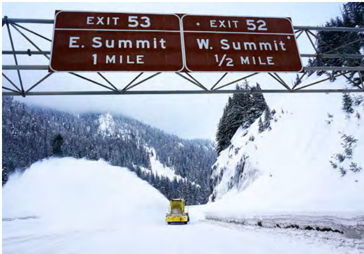
Photo: Snow removal on Snoqualmie Pass Source: Washington State Department of Transportation
