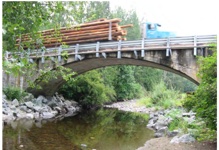
Photo: Log truck over concrete arch bridge Source: Washington State Department of Transportation
