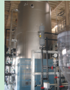
Ion exchange resin tower
