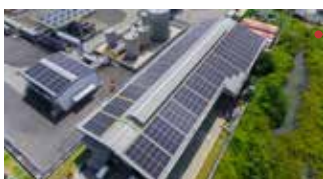
Solar rooftop panels installed at the JIIPE utility center open opportunities for tenant utilization.
