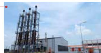
Gas-powered electricity generators will be used as the primary power source.
