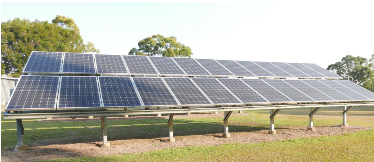
Image 6: Solar system at CVRA
