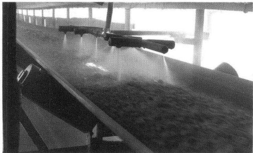
Figure 2 Atomised water sprinkling on belt conveyors
