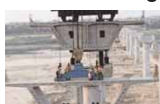
Awasthi said that the total length of Bundelkhand Expressway project was 296 km. He said keeping in view the quality, the construction of ROBs and structures on the expressway was also being done at a rapid pace. In-charge of Bundelkhand Expressway and UPEIDA Chief Engineer Manoj Kumar Gupta said that out of the total length of
