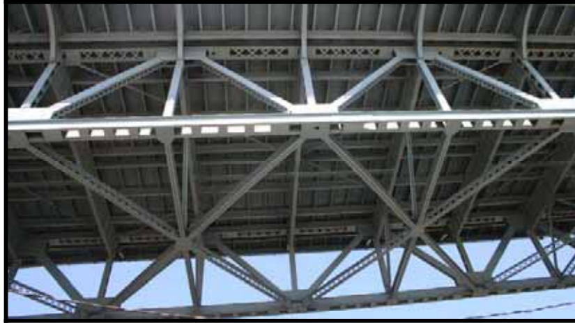
Image 4: Detail of Warren deck truss and I-beam grating, Image courtesy of EHT Traceries, May 2006
