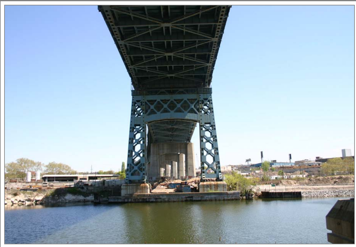
Photo V-19. View of Kosciuszko Bridge supports over Newtown Creek, looking northeast from Greenpoint, Brooklyn, New York
