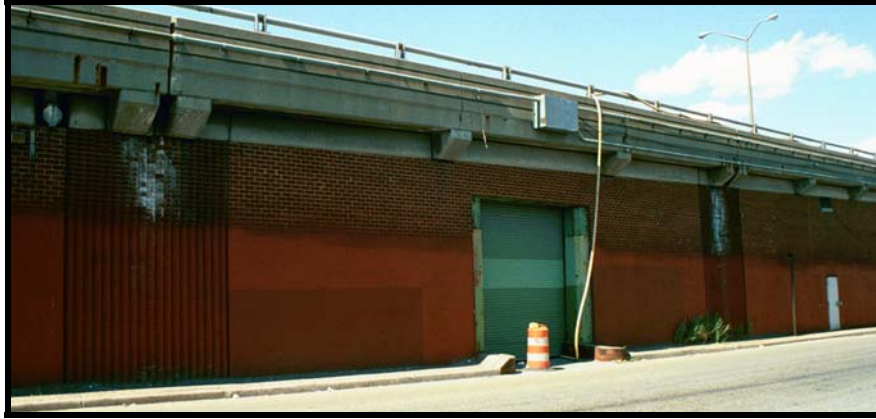
Image 3: Detail of bridge abutments and storage spaces, Image courtesy of EHT Tracerics, May 2006
