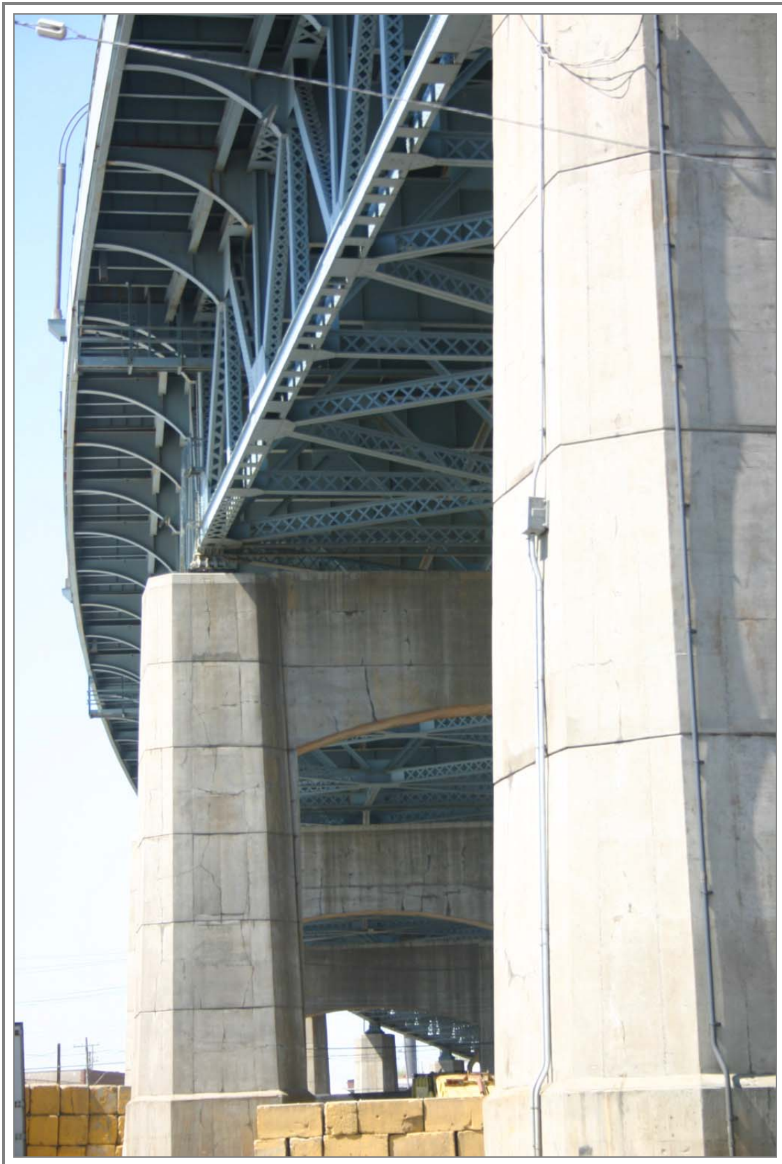
Detail of concrete piers and substructure, looking northeast from Greenpoint, Brooklyn, New York
