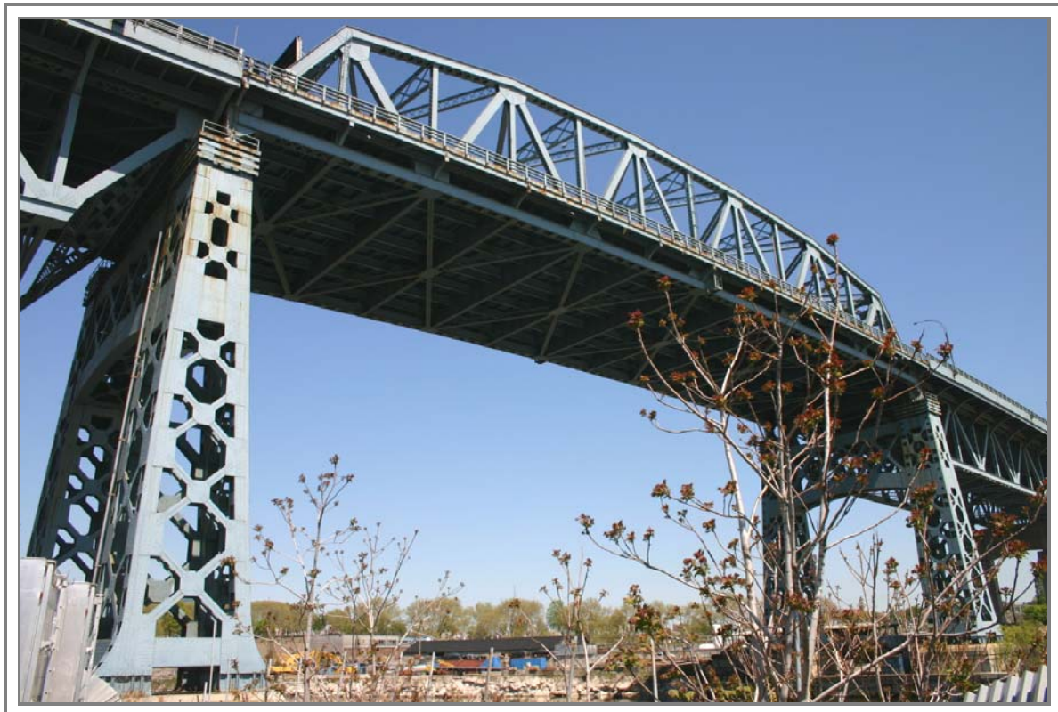
Photo V-18. Detail of the Warren truss main span and overhead bracing, looking northwest from Greenpoint, Brooklyn, New York
