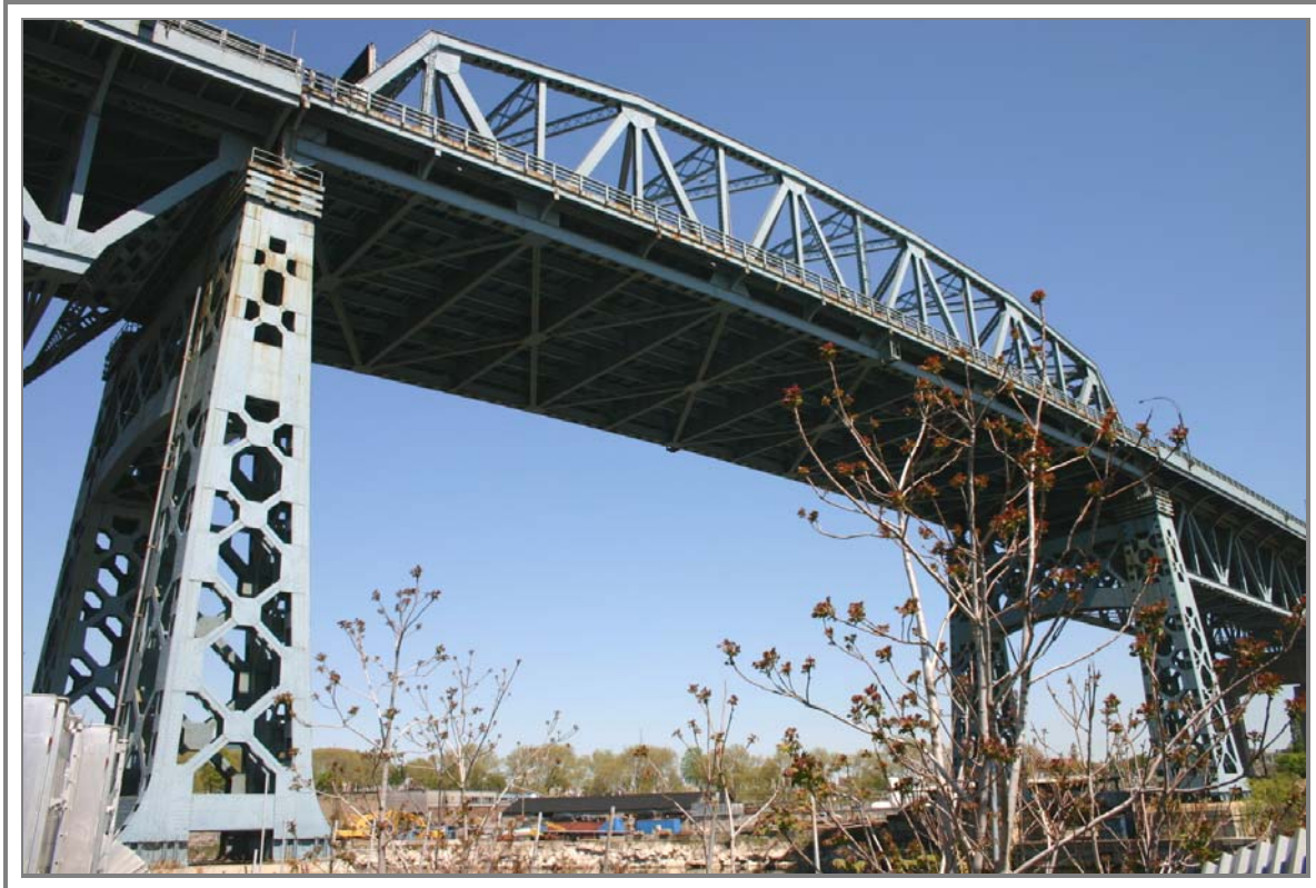
Detail of the Warren truss main span and overhead bracing, looking north from Greenpoint, Brooklyn, New York
