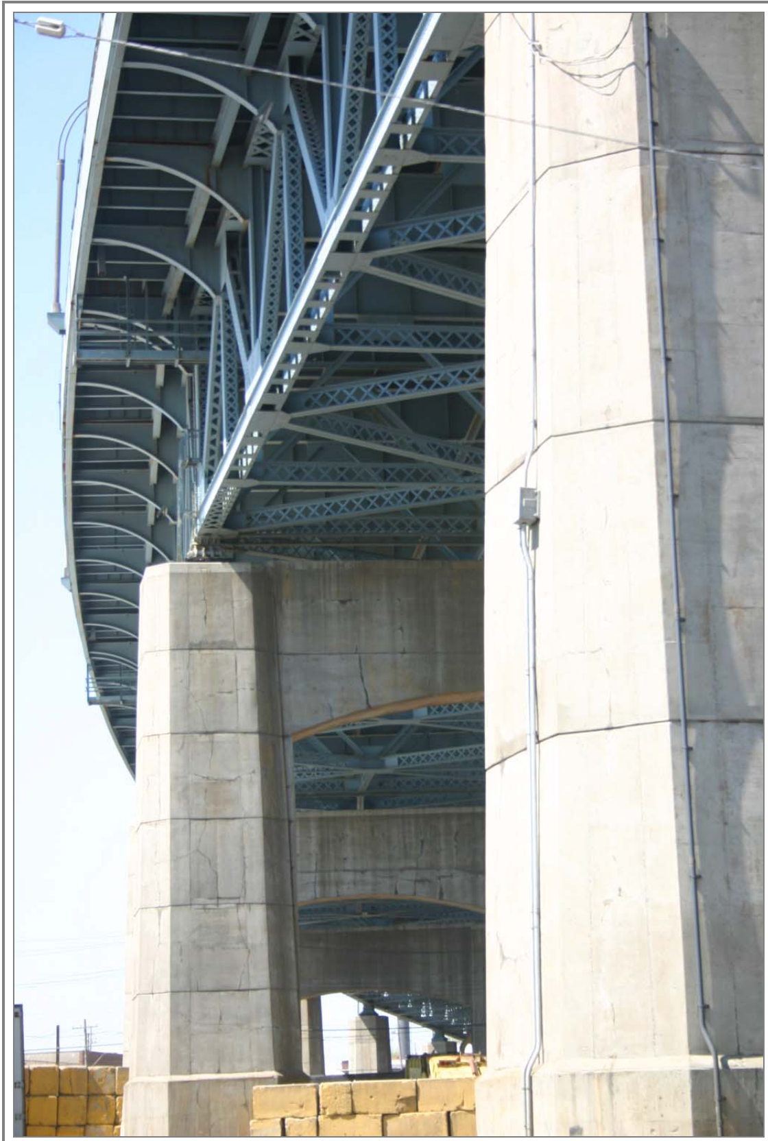
Photo V-17. Detail of concrete piers and substructure, looking southwest from Greenpoint, Brooklyn, New York
