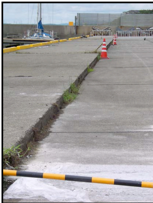
Figure 8.5: Kashiwazaki Marina - Evidence of minor settlement behind quay walls (Site SD3, N37.36093° E138.52027°, photo taken 7/22/07 13:12).
