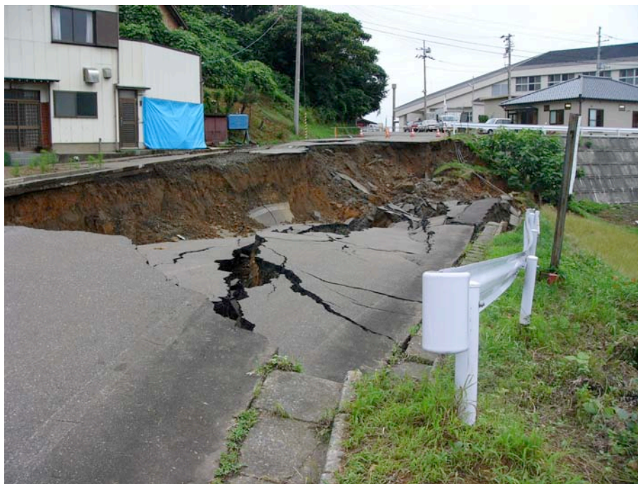
Figure 3.8: Road embankment failure off Route 8 on the way to Kasashima (Site YT18; N 37.33325 ° E 138.46500°, photos taken 7/21/07 at approximately 15:40). The slope appears to have undergone previous stabilization using slope grading and gabion baskets to support the toe.
