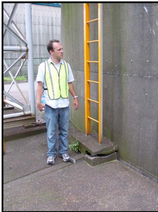
Figure 8.30: Kashiwazaki Port (Taiheiyo Cement Facility) - Evidence of minor to moderate settlement of sandy fill adjacent to one of the large diameter tanks (Site SD9, approximately N37.36665° E138.53983°, photo taken 7/22/07 15:48).
