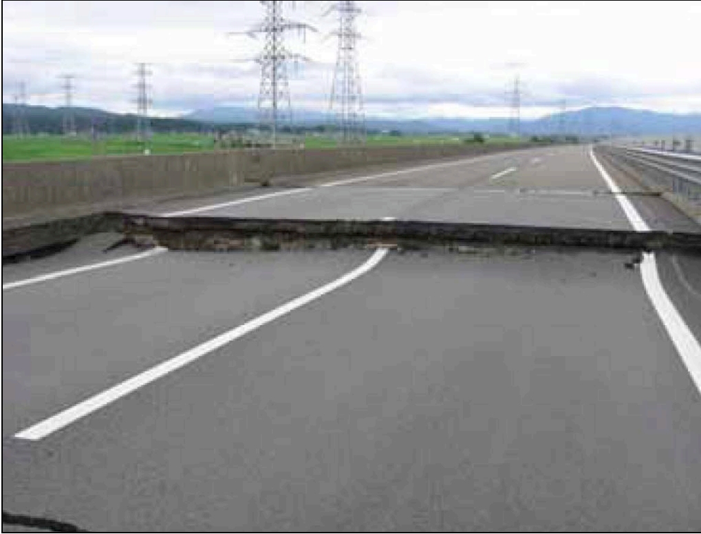
Fig. 6.8. Damage to approach slab and embankment at Yoshiigawa Bridges.
