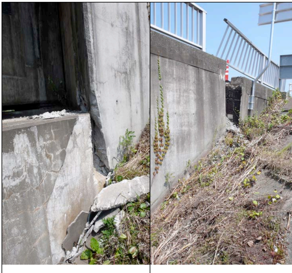
Fig. 6.51. Abutment and wingwall damage from the earthquake.
