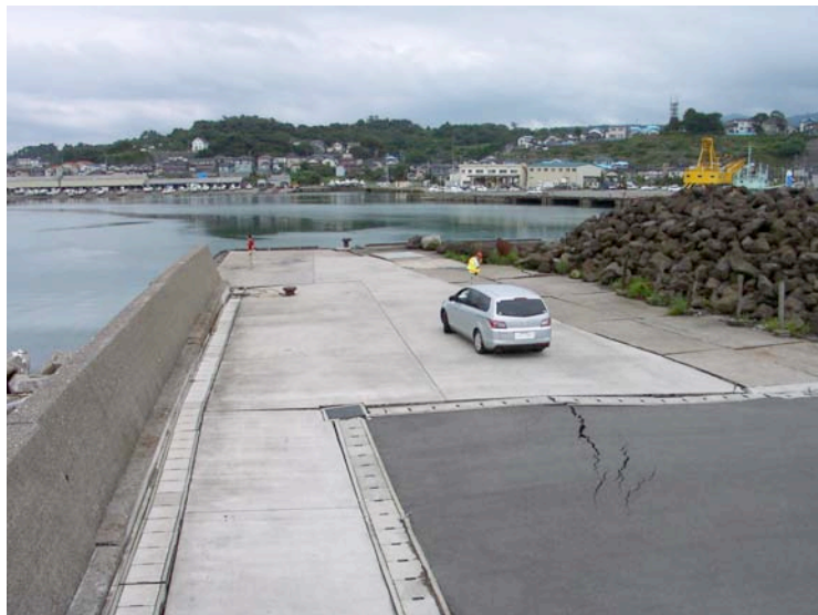
Figure 8.13: Kashiwazaki Port - Evidence of lateral ground deformation adjacent to the outer quay wall (Located near site RK25/SA25/YT4, N37.36713° E138.53210°, photo taken 7/21/07 15:49).
