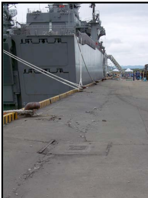
Figure 8.25: Kashiwazaki Port - Evidence of very minor lateral movement of quay walls and minor settlement located along the northern face of the terminal used as the berth for the Japan Self Defense Force (Site SD8, approximately N37.36680° E138.53825°, photo taken 7/22/07 15:24).
