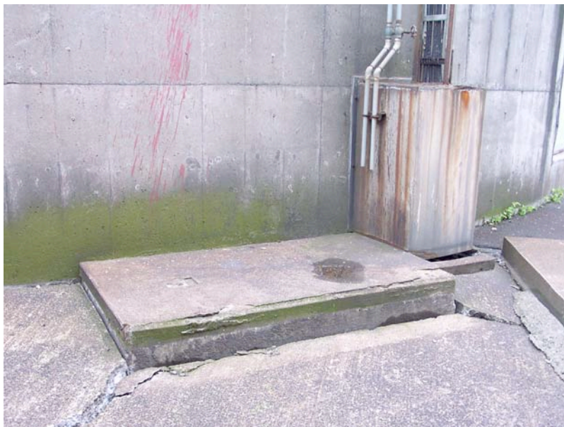
Figure 7.8: Kashiwazaki Port (Taiheiyo Cement Facility) - Evidence of minor to moderate settlement of sandy fill adjacent to one of the large diameter tanks (Site SD 9, approximately N37.36665° E138.53983°, photo taken 7/22/07 15:48).
