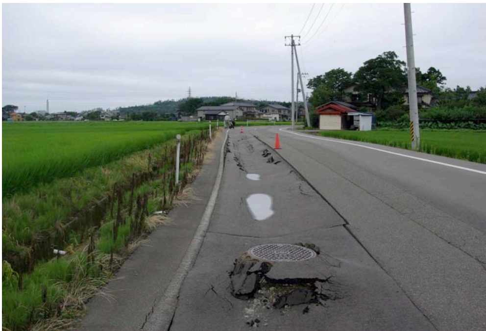
Figure 9.9: Pavement damage caused by utility trench liquefaction (Site SA21, N37.38950° E138.59662°, photo taken 7/21/07 14:57).
