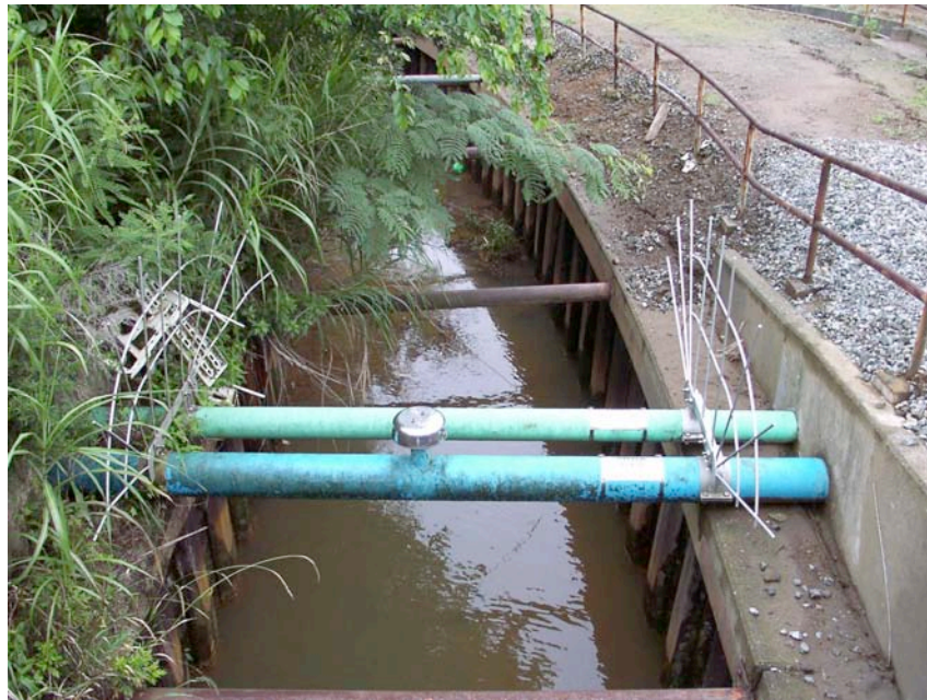
Figure 10.2: Example of short span pipes (water and gas) across a channelized stream exhibiting very minor ground deformation. No damage to the pipes was observed (Site SD12, N37.36663° E138.59223°, photo taken 7/23/07).
