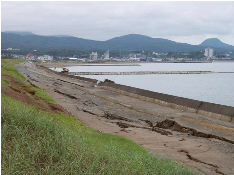
Figure 8.38: Ground deformations adjacent to the embankment and seawall (Location is southwest of Site SD1, photo taken 7/22/07 11:42).
