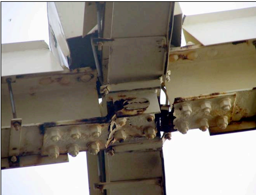
Fig. 6.26. Torn cross bracing connection on Yonahime Bridge.
