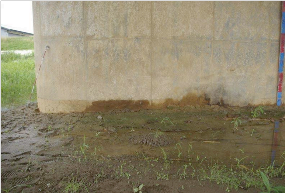
Fig. 6.45. Soil settled around pier in riverbank (photo courtesy of Scott Brandenburg).
