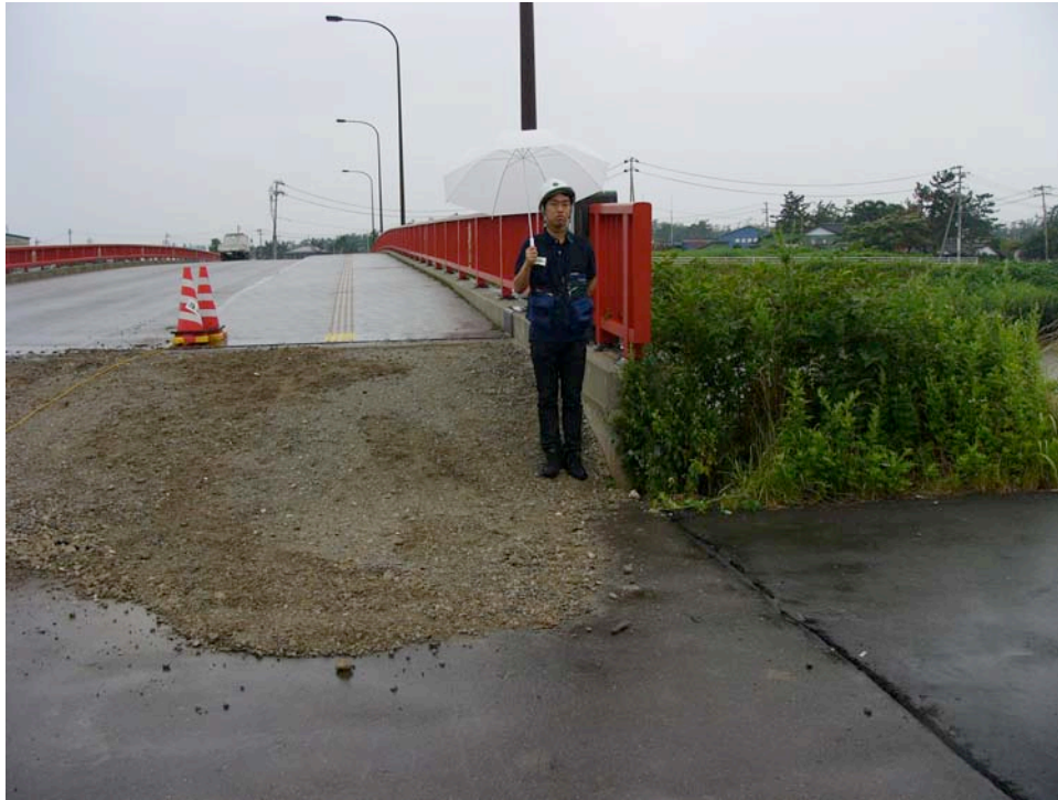
Figure 9.6: Vertical offset at the approach of Kai-Un Bridge that has been temporarily repaired with gravel fill to permit access (Site YT3, N37.39232° E138.58063°, photo taken 7/20/07 12:42). A vertical offset of 33 cm was measured at the adjacent abutment (left of this photo).
