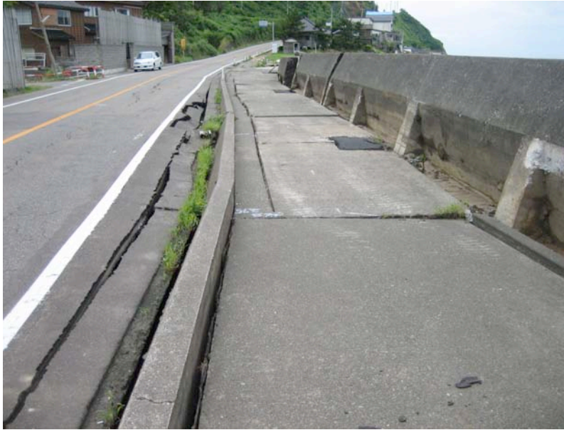
Figure 8.43: Liquefaction-induced damage to the seawall and adjacent roadway (Site RK35, N37.48497°, E138.62645°, photo taken 7/23/07).
