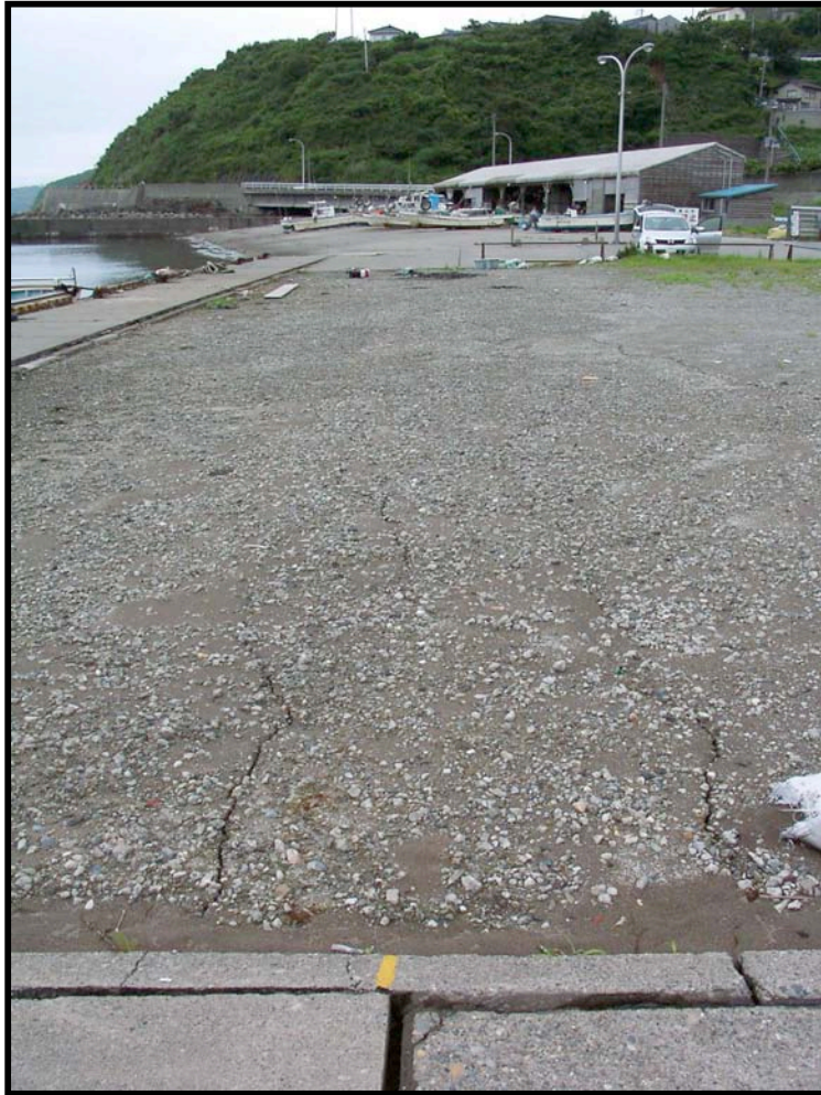
Figure 8.1: Minor ground failure along the waterfront at Kasashima (Site RK21, N37.33702° E138.46680°, photo taken 7/21/07 14:49). The limited extent of the ground cracking indicated incipient lateral movement.
