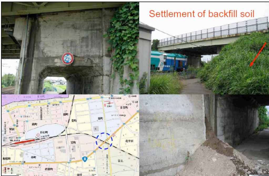
Fig. 6.17. Damage and repairs where railway crosses Highway 8 Bridge (courtesy G. Watanabe, Tokyo Institute of Technology).
