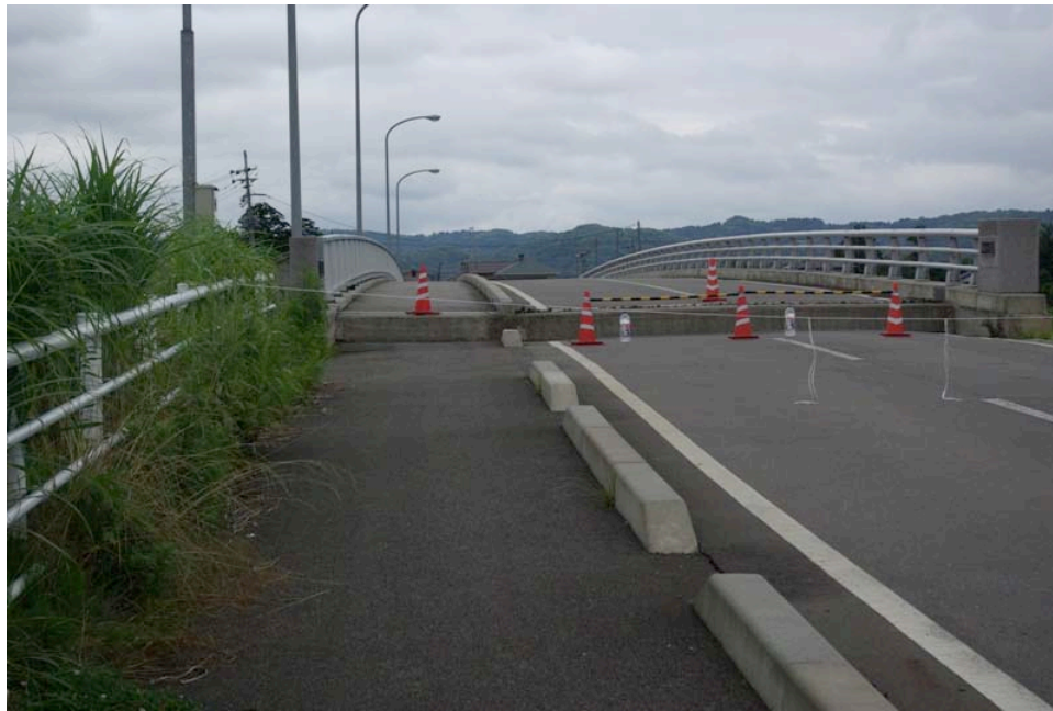
Figure 9.7: Vertical offset at approach of rural bridge that has not yet been repaired (Site SA22 N37.38439° E138.60083°, photo taken 7/21/07 15:00).
