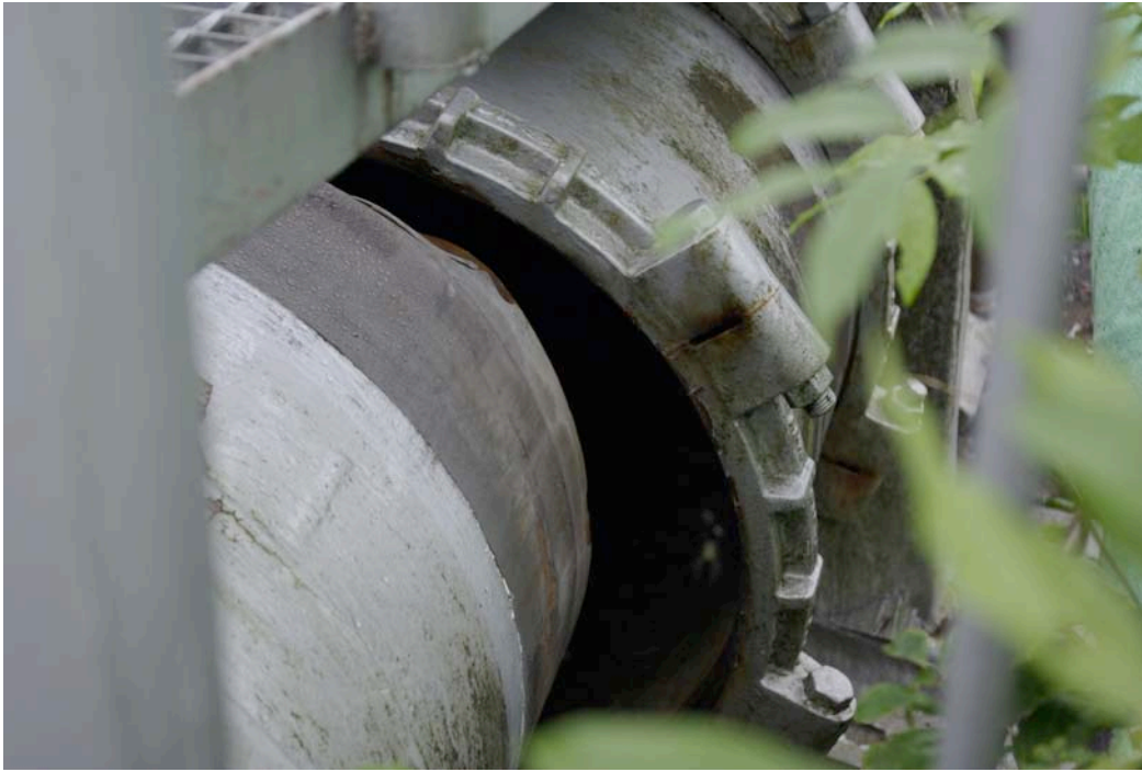
Figure 10.3: Damage to a water pipe at a stream crossing (Site RK4/YT3, N37.39233° E138.58063°, photo taken 7/20/07).
