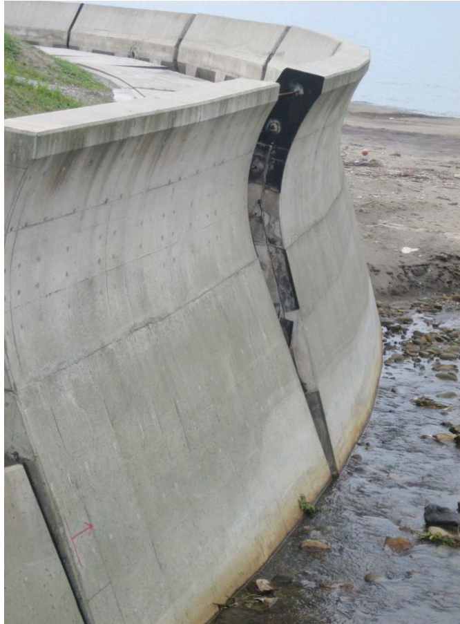
Figure 4.31: Seawall Failure as a result of embankment movement into a seawall founded on top of liquefied beach sands. (Site RK37, N37.45478° E138.60927°, 7/22/2007).
