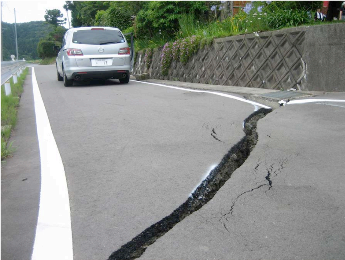
Figure 9.5: Typical road damage near epicentral region (Site RK30, N37.45727° E138.65328°, photo taken 7/22/07 09:46). Cracks of 5 to 10 cm were often quickly paved over in high-traffic areas, within one or two days of the earthquake. On local community roads with alternate traffic routes, this damage was not immediately repaired.
