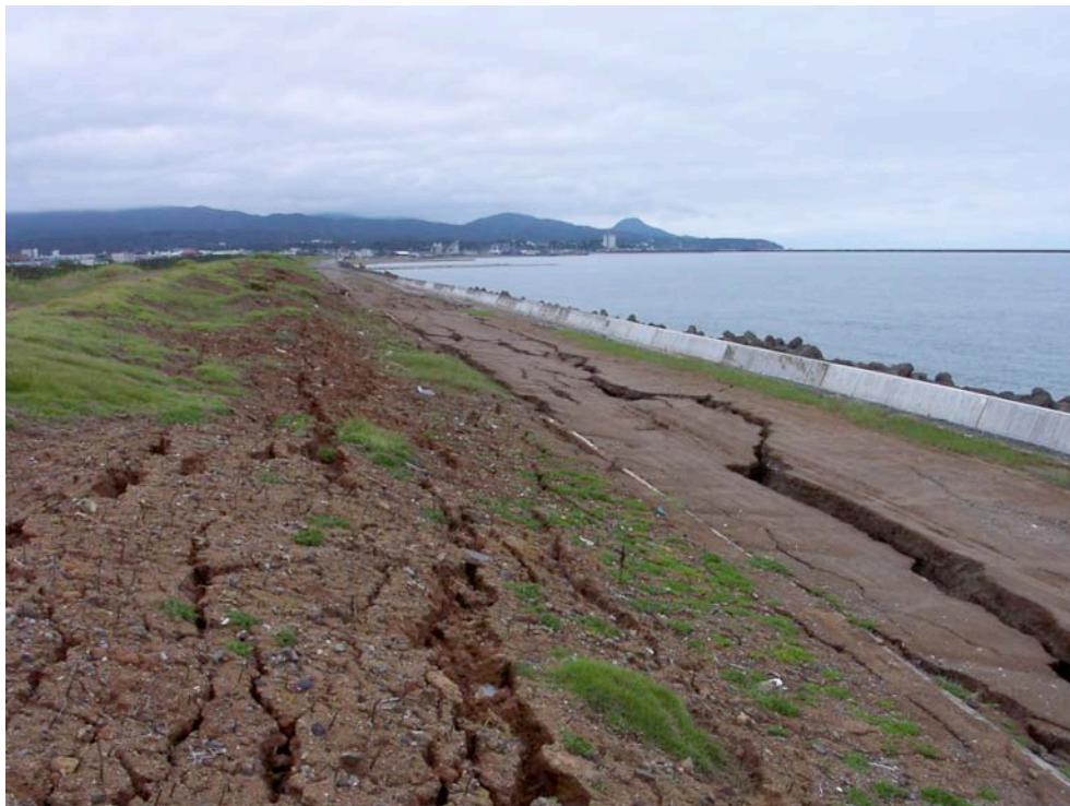
Figure 8.36: Representative cracking and lateral displacement of the clayey earth embankment adjacent to the seawall (Location is southwest of Site SD1, photo taken 7/22/07 11:35).
