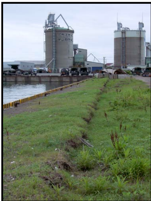
Figure 8.21: Kashiwazaki Port - North facing, landward quay wall exhibiting lateral movement and rotation of caissons (Site SD7, N37.36593° E138.53692°, photo taken 7/22/07 15:12). The Taiheiyo Cement Tanks are in the background.
