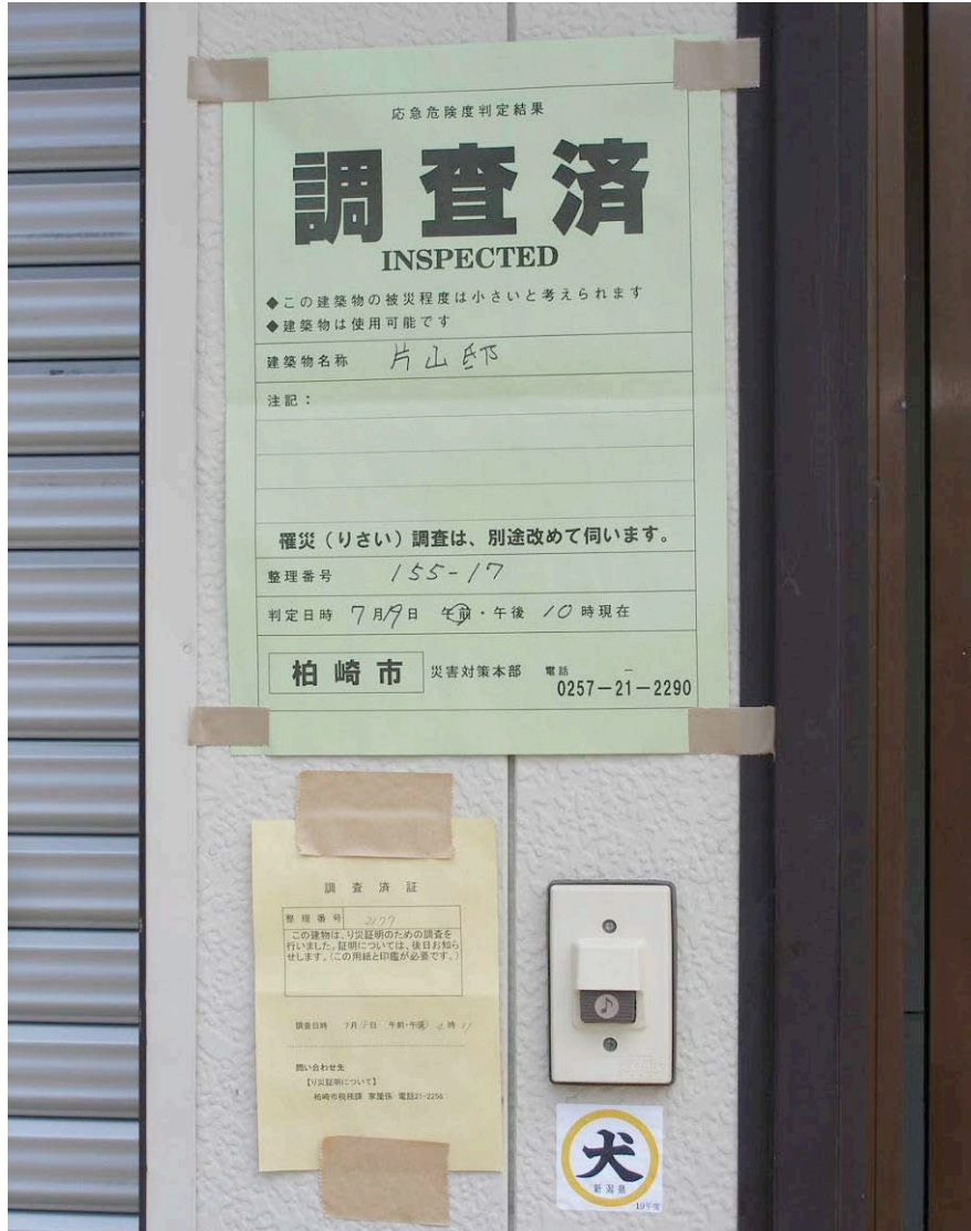
Figure 11.7: A building in Kashiwazaki city that has been through two surveys, with both a green tag as well as a standard yellow notice that the damage certification survey has also been completed.
