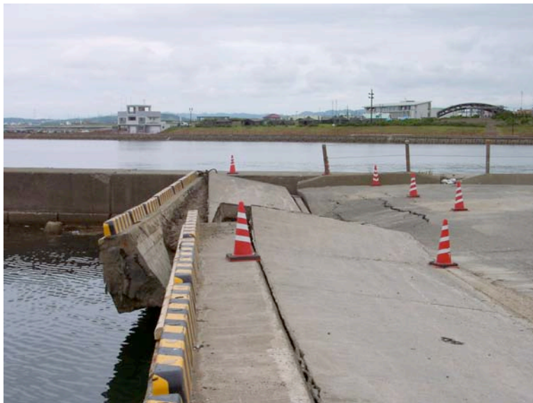
Figure 8.28: Kashiwazaki Port - Significant liquefaction-related damage to the quay walls located adjacent to the U River (Site SD8, approximately N37.36680° E138.53825°, photo taken 7/22/07 15:36).
