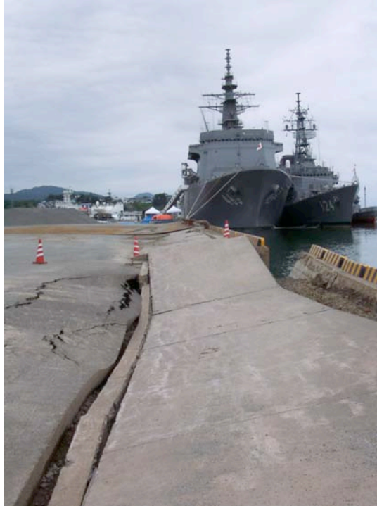
Figure 8.27: Kashiwazaki Port - Significant liquefaction-related damage to the quay walls located at the eastern edge of the terminal adjacent to the mouth of the U River (Site SD8, approximately N37.36680° E138.53825°, photo taken 7/22/07 15:32).
