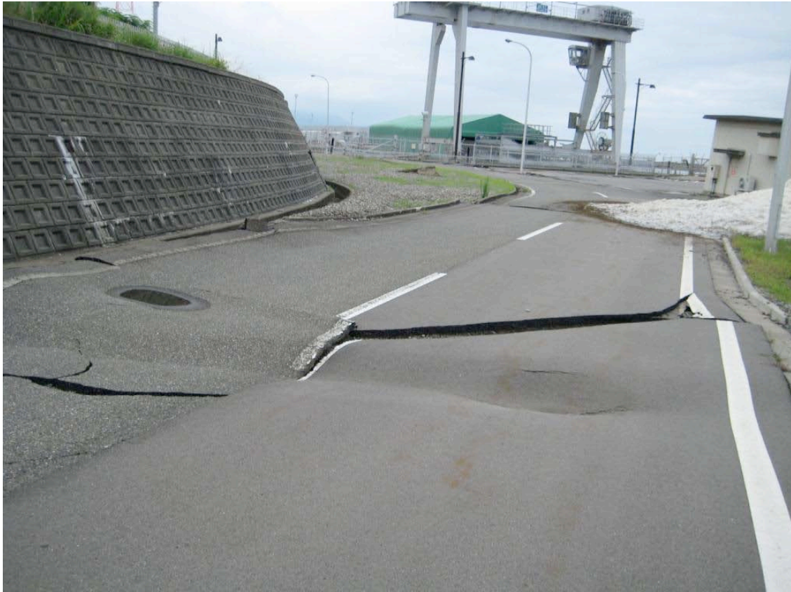
Figure 5.3: Damaged road at power plant.
