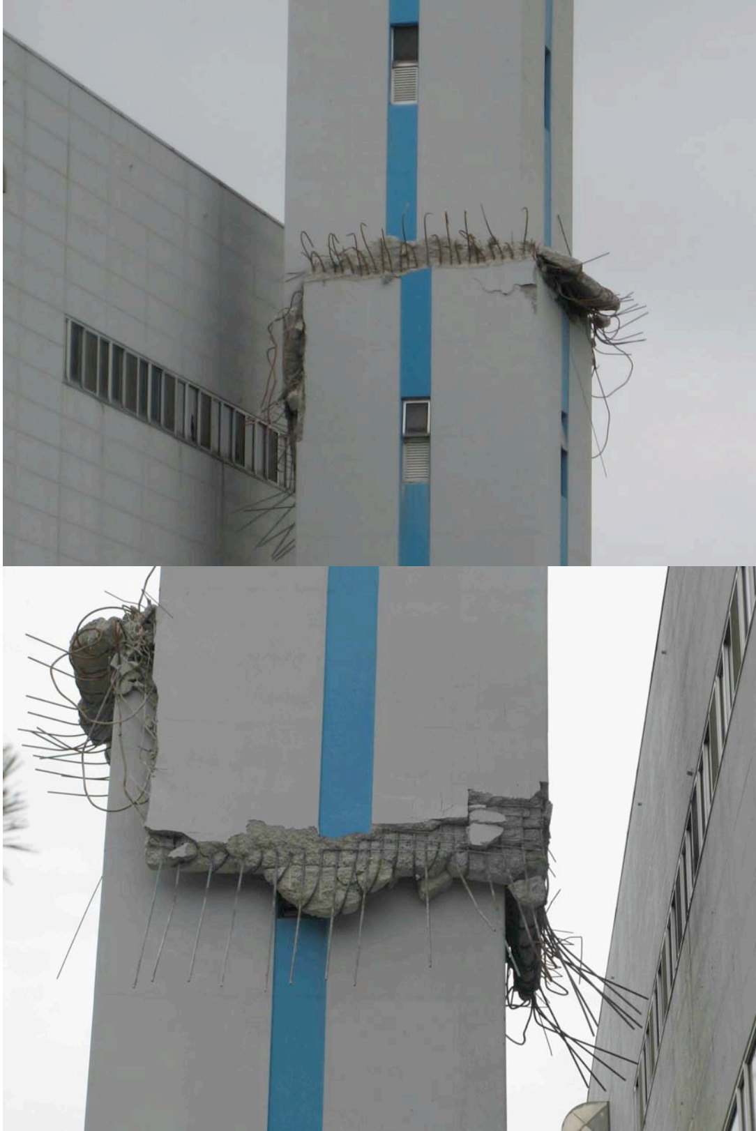
Figure 5.9: Details of failure of reinforced concrete stack (Site SP31, N37.3939° E138.5840°).
