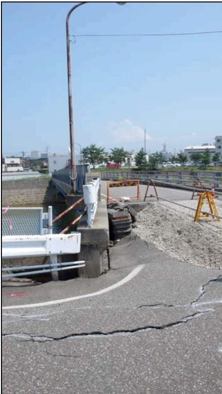
Fig. 6.62. Closer view of settlement at south abutment.
