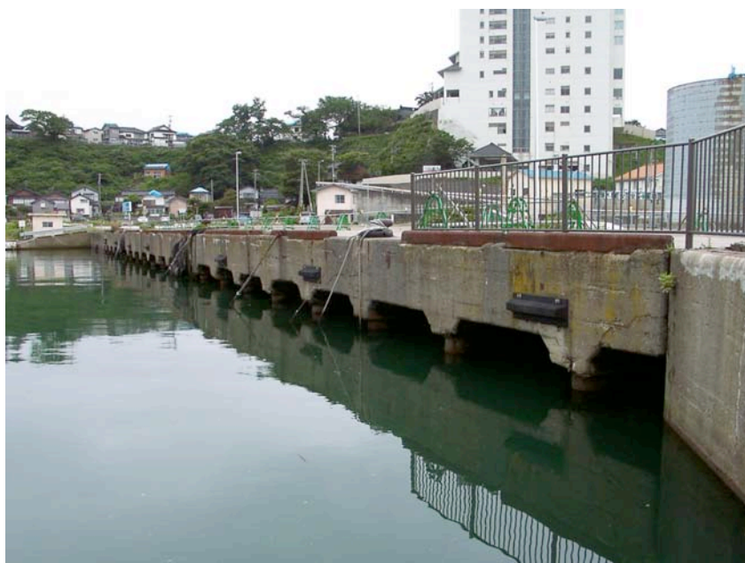
Figure 8.6: Kashiwazaki Port - Older, undamaged pile-supported wharf located in the western portion of the port facility (Site RK25/SA25/YT4, N37.36713° E138.53210°, photo taken 7/21/07 16:12).
