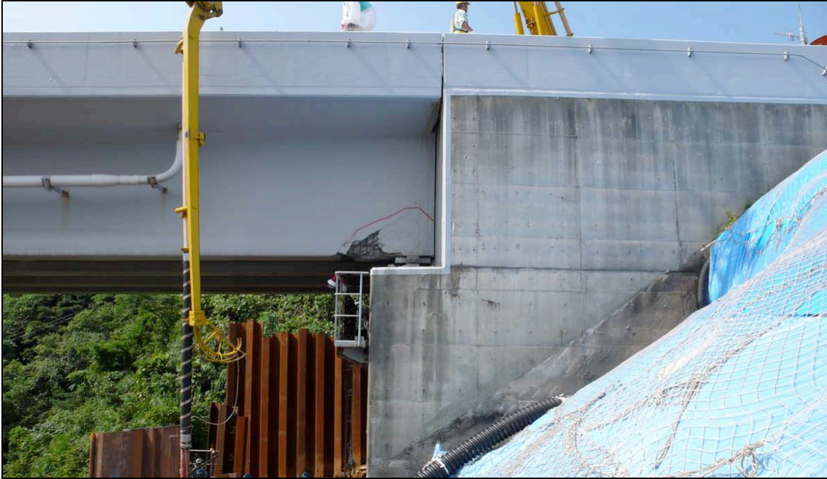
Fig. 6.3. Damage at north end of the west Hachisaki Bridge.
