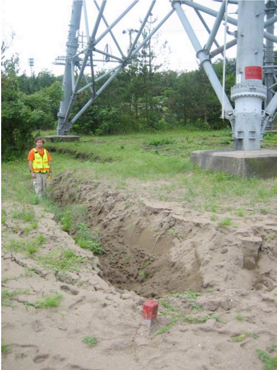
Figure 4.35: Settlement of ground adjacent to grade beam between footings of a high voltage transmission line tower (Site RK40, N37.41633° E138.60792°, 7/22/2007).
