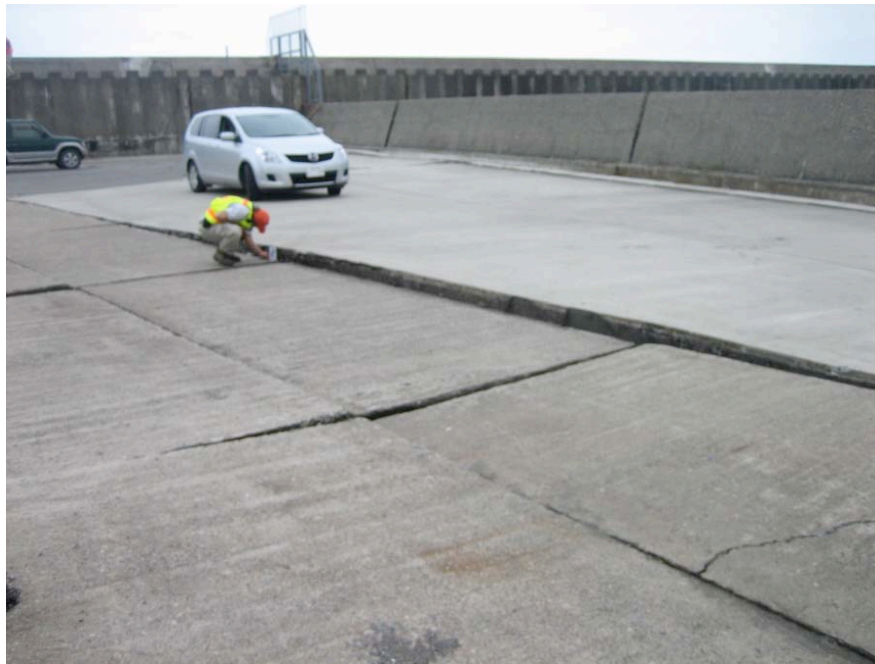
Figure 4.18: Kashiwazaki Harbor - South area experienced ground damage from liquefaction induced lateral spreading and settlement of separated pier slab sections (Site RK25, N37.36713° E138.53210°, 7/20/2007).
