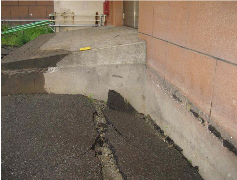
Figure 4.15: Kashiwazaki Wastewater Treatment Plant on the south side of Sabaishi River near the Sea of Japan (Site RK9 N37.38748° E138.56587°, 7/19/2007). Damage to the main building from liquefaction of ground resulted in meter-scale ground settlements.
