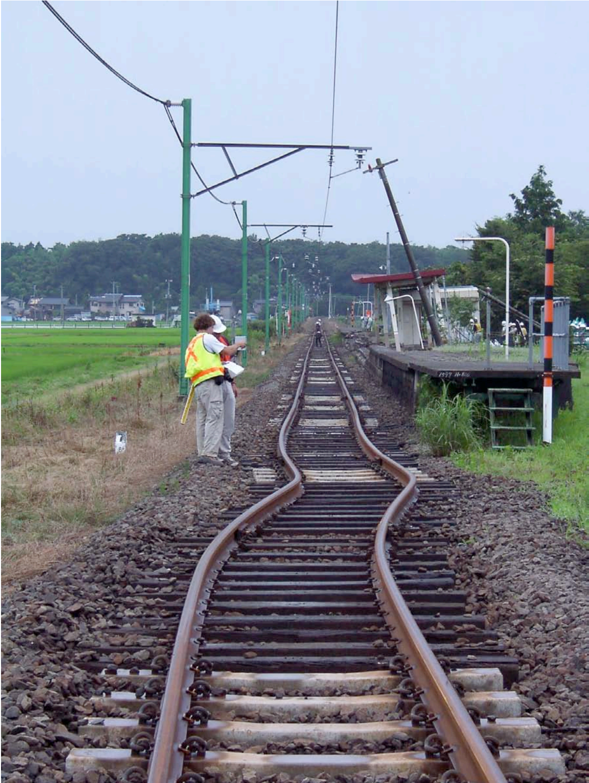
Figure 9.12: Lateral deformation of train tracks at Arahama Station (Site RK13, N37.40555° E138.60197°, 7/21/07 09:52).
