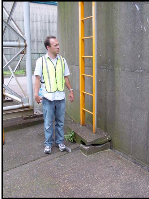
Figure 7.9: Kashiwazaki Port (Taiheiyo Cement Facility) - Evidence of minor to moderate settlement of sandy fill adjacent to one of the large diameter tanks (Site SD 9, approximately N37.36665° E138.53983°, photo taken 7/22/07 15:48).
