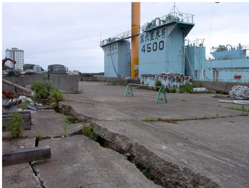
Figure 8.19: Kashiwazaki Port - Steel Scrap Transport Facility showing evidence of ground failure due to liquefaction of sand fill and damage to concrete aprons (Site SD6, N37.36668° E138.53565°, photo taken 7/22/07 14:46).
