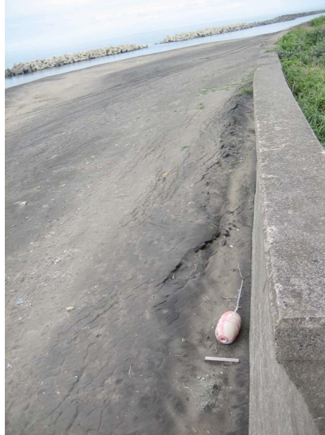
Figure 8.41: Evidence of minor liquefaction and lateral spreading in sandy beach deposits adjacent to the seawall (Site RK37, N37.45478°, E138.60927°, photo taken 7/23/07).
