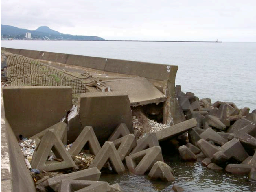
Figure 8.33: Partial collapse of a portion of the seawall located at the lateral, seaward step in alignment just west of the damaged cement plant (Site SD1, N37.38868° E138.56413°, photo taken 7/22/07 11:18).
