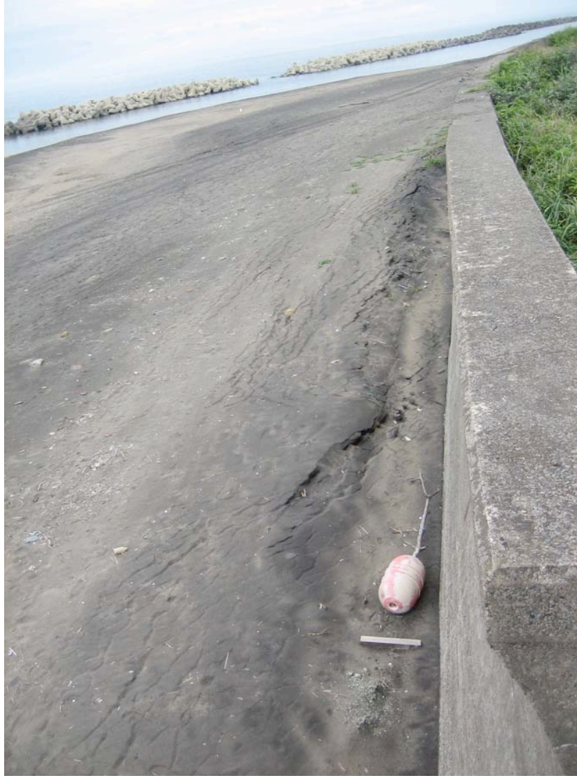
Figure 4.32: Lateral spreading related ground cracking in front of seawall. (Site RK37, N37.45478° E138.60927°, 7/22/2007).
