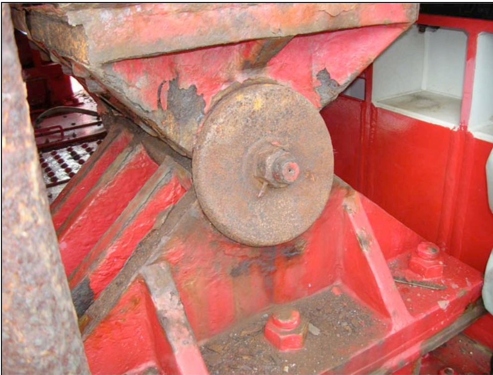
Fig. 6.23. Deformation of Bearing Pin-Cap caused by uplift force (courtesy of S. Unjoh, PWRI).
