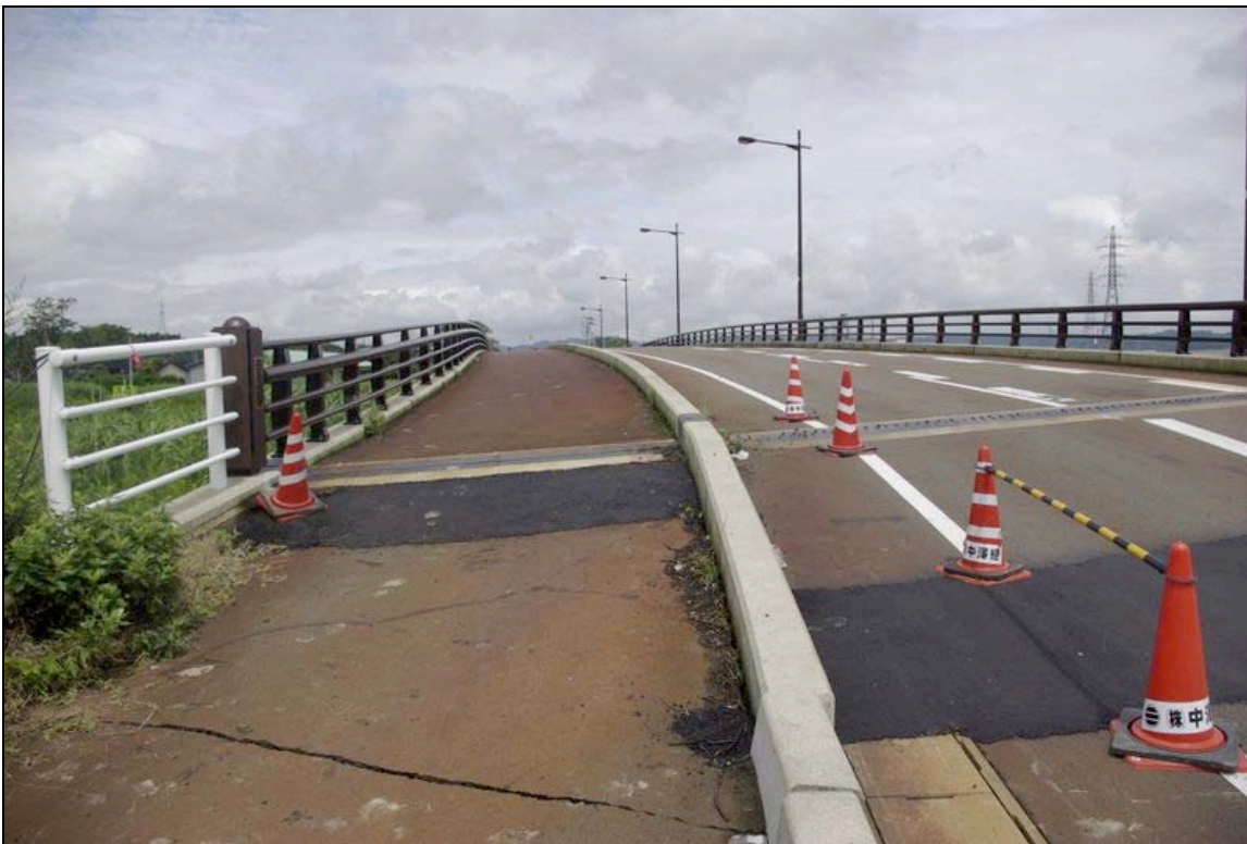
Fig 47. Repairs to bridge approach on Nagomi Bridge (photo courtesy of Scott Brandenburg).
