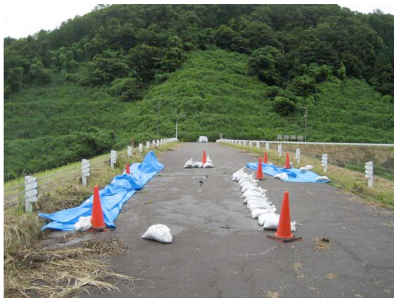
Figure 3.9: Embankment cracking and settlement of South Dam near Miyamo Parking Area along Highway 8, Nagaoka-Shi region (Site RK50; N37.43267° E138.73674°, photos taken 7/23/07 at approximately 11:15). The dam is a 15-meter tall, 97.5-meter wide earth fill structure with 3(H):1(V) downstream and 3.5(H):1(V) upstream benched slopes. Crest elevation is 63 meters and normal pool elevation is 55 meters. Observations were made of an embankment slope failure along the crest of this dam, through half the crest width (~4 m). Settlement and deformation occurred along a 10 m long section with up to 4 cm each of lateral and vertical deformation in the down slope direction. Contour-parallel ground cracking (2-4 cm wide, 1-2 m long) along the ground-spillway interface were also observed, two-thirds of the way down the dam face. The reservoir was empty and appeared to not have been filled in some time judging by the height of vegetation growing in the reservoir area.
