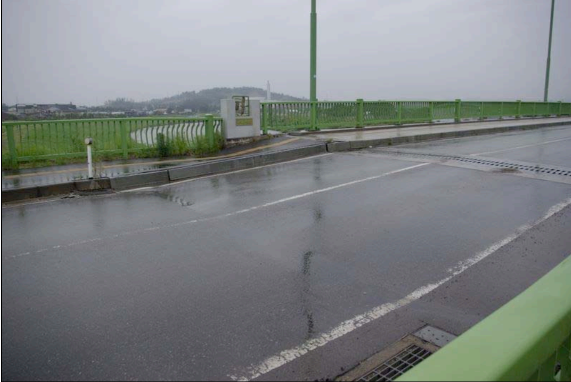
Fig. 6.39. Settlement of north bridge abutment.
