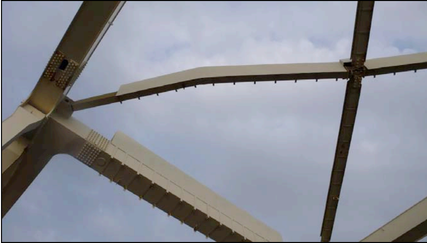
Fig. 6.25. Buckled cross bracing on Yonahime Bridge.
