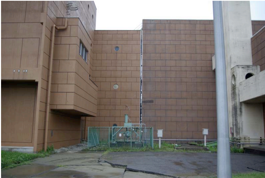
Figure 10.4: Ansui-Chou waste water treatment plant showing evidence of lateral spreading and extension of the structure (Site RK9, N37.38748° E138.56587°, photo taken 7/20/07).
