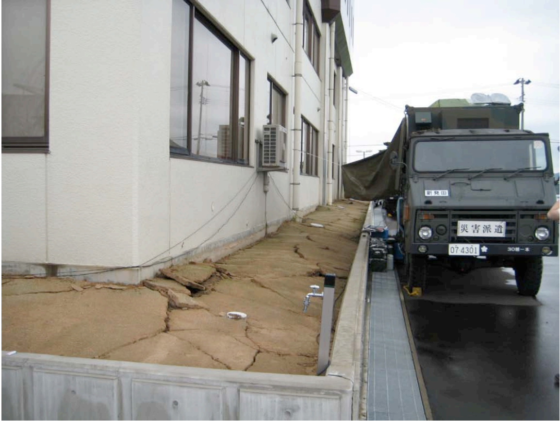
Figure 5.22: Disruption of soil surrounding a government building in Kariwa (Site SP33, N37.4223° E138.6222°).
