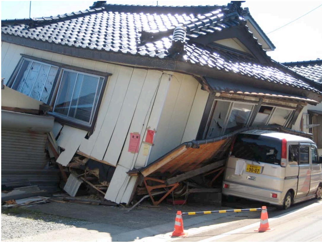
Figure 5.10: Collapse of house (N37.367°, E138.567°).
