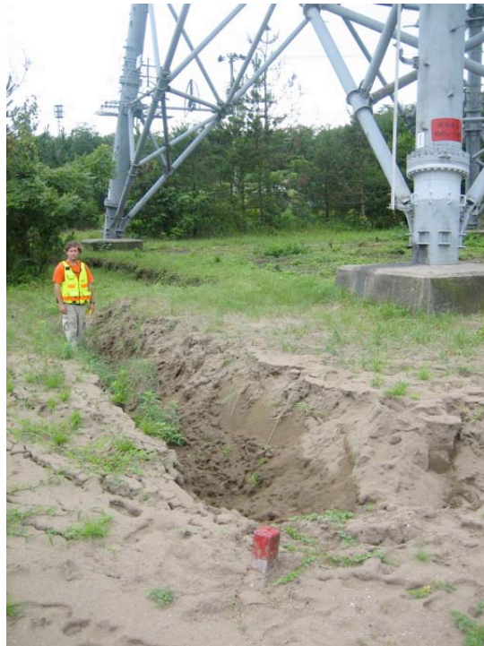
Figure 10.5: Ground failures at the site of a high voltage tower (Site RK40, N37.41633° E138.60792°, photo taken 7/24/07). No evidence of structural damage to the towers was observed.
