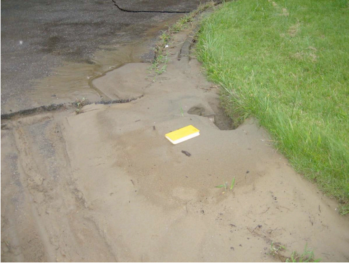
Figure 4.17: Kashiwazaki Wastewater Treatment Plant on the south side of Sabaishi River near its outlet to the Sea of Japan (Site RK9 N37.38748° E138.56587°, 7/19/2007). Liquefaction features were abundant near the wastewater treatment facility.
