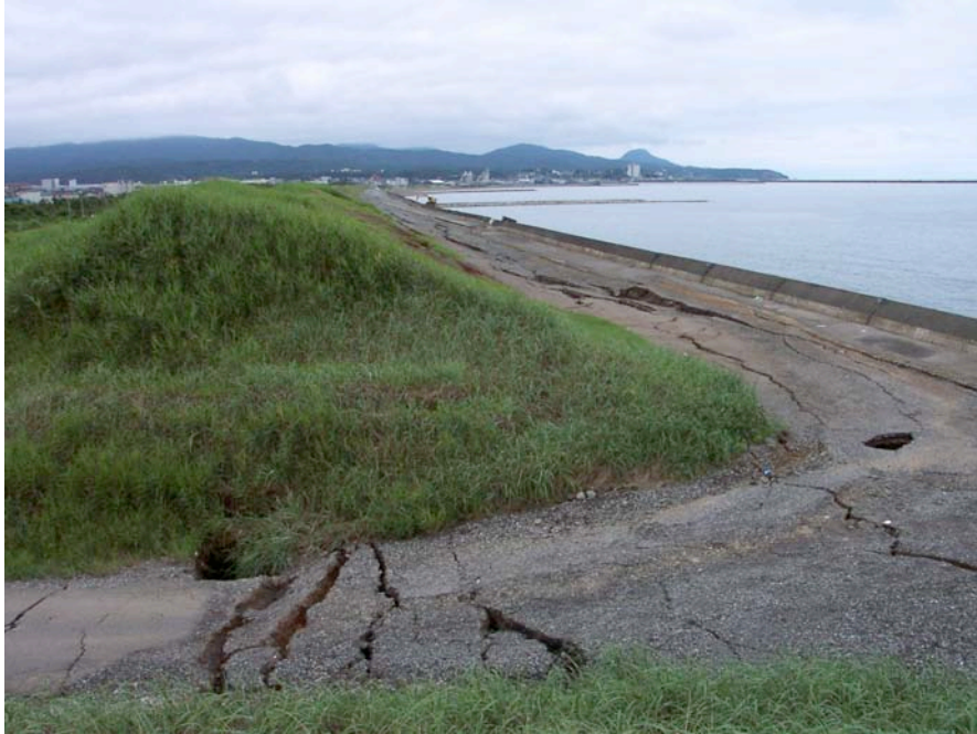
Figure 8.37: Ground deformations adjacent to the embankment and seawall (Location is southwest of Site SD1, photo taken 7/22/07 11:41).
