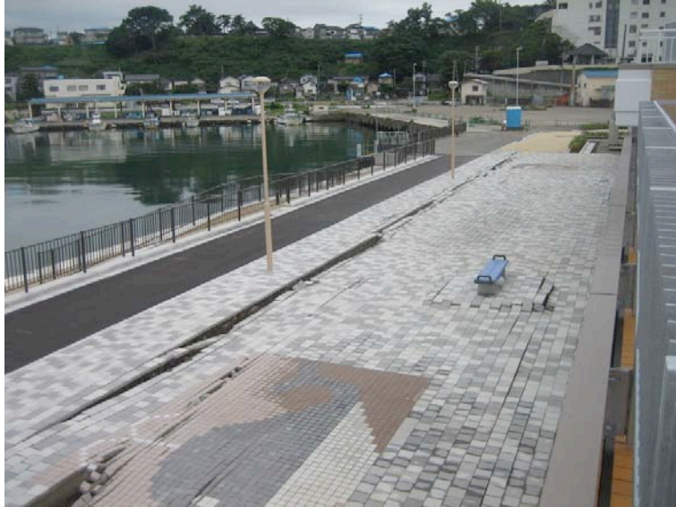
Figure 4.25: Kashiwazaki Harbor - South area experienced ground damage from liquefaction-induced lateral spreading and settlement. A harbor front caisson rotated toward the harbor, to the left of the photo, initiating lateral displacement of the soil behind it, between the caisson and port building. Settlements can also be seen in this photo. (Site RK25, N37.36713° E138.53210°, 7/20/2007)
