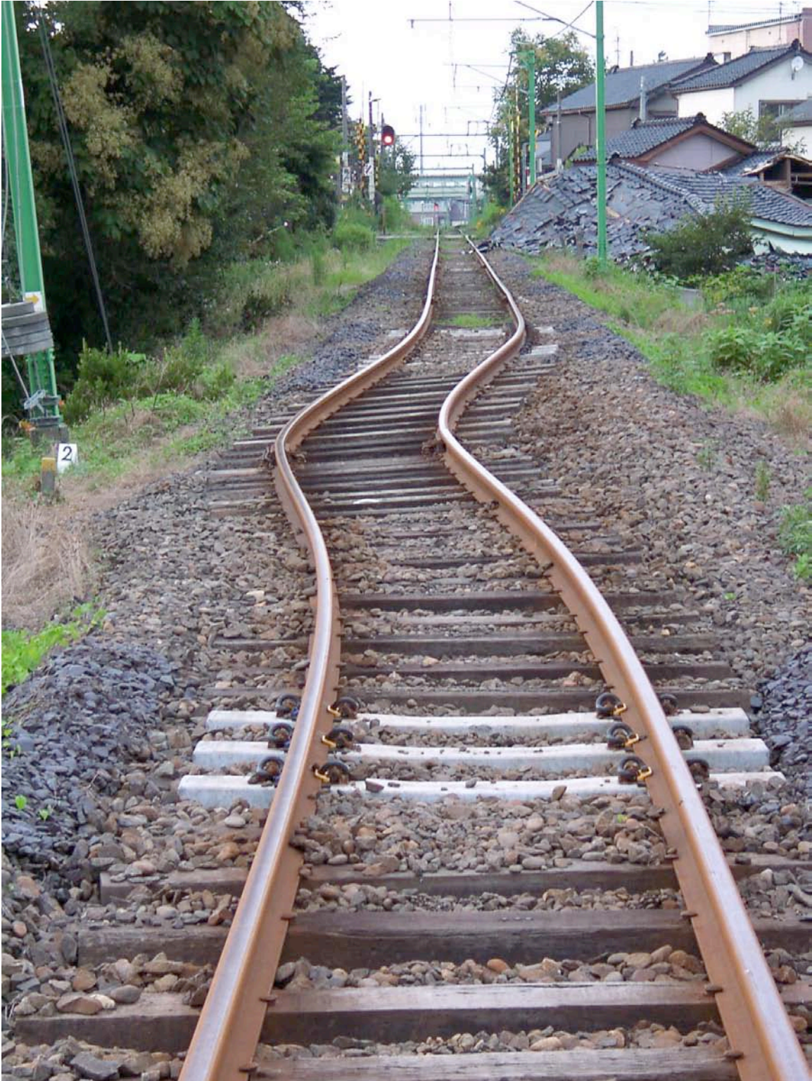
Figure 9.13: Lateral railway buckling (Site RK28, N37.37037° E138.56475°, 7/21/07 18:01).
