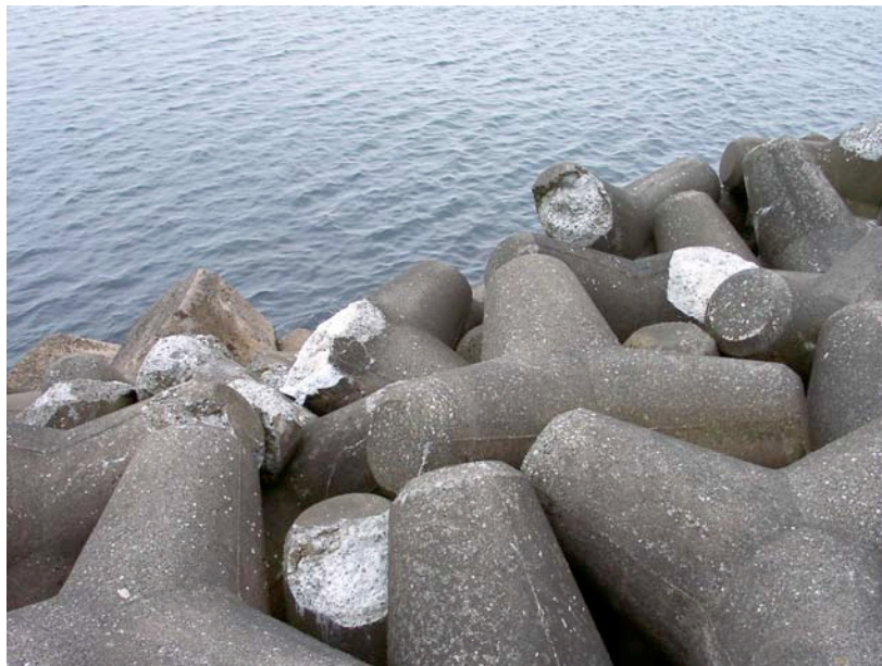
Figure 8.15: Kashiwazaki Port - Likely earthquake-related damage to tetrapod wave armor units (Located near site RK25/SA25/YT4, N37.36713° E138.53210°, photo taken 7/21/07 15:53).
