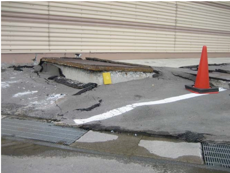
Figure 4.36: Plant 5 Store - Ground settlement in dune sand was observed around the building and an underground storage tank had been uplifted (Site RK41, N37.41468° E138.6084°, 7/22/2007).
