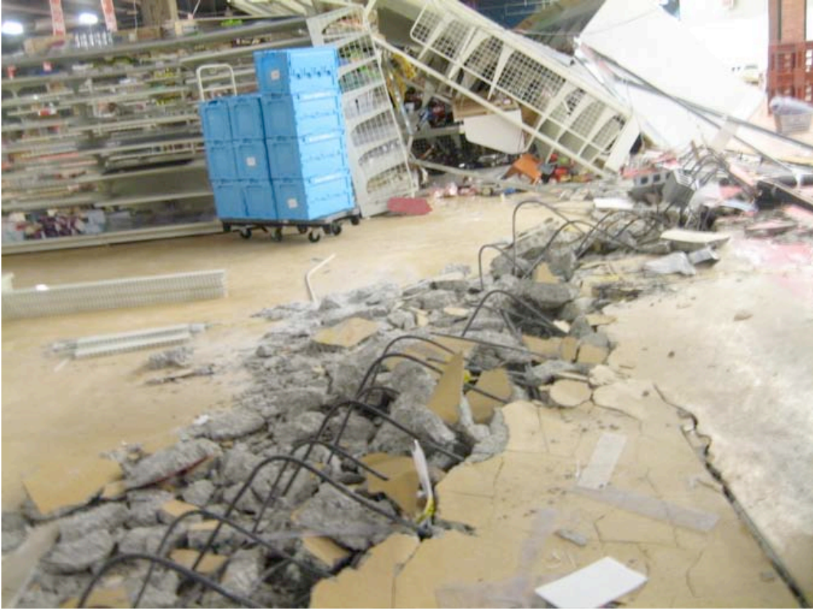
Figure 4.39: Plant 5 – Failure of slab on grade with buckled reinforcing bars. (Site RK41, N37.41468° E138.60840°, 7/22/2007).
