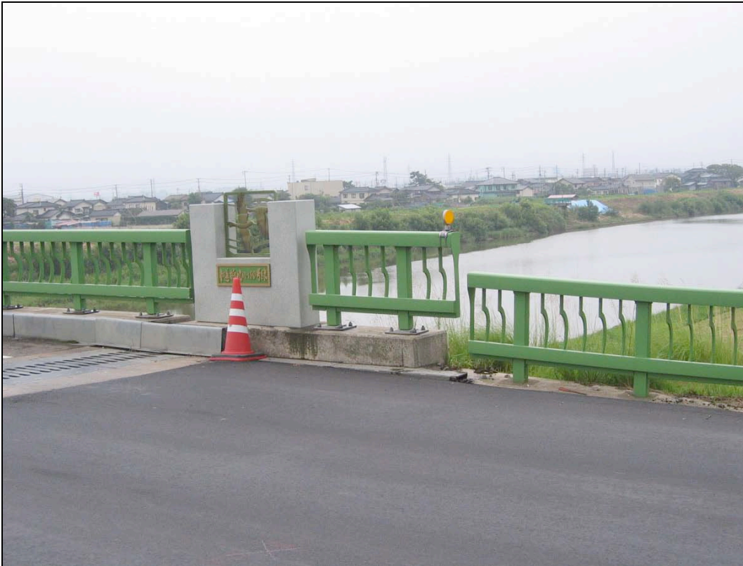
Fig. 6.35. Settlement of north bridge approach.
