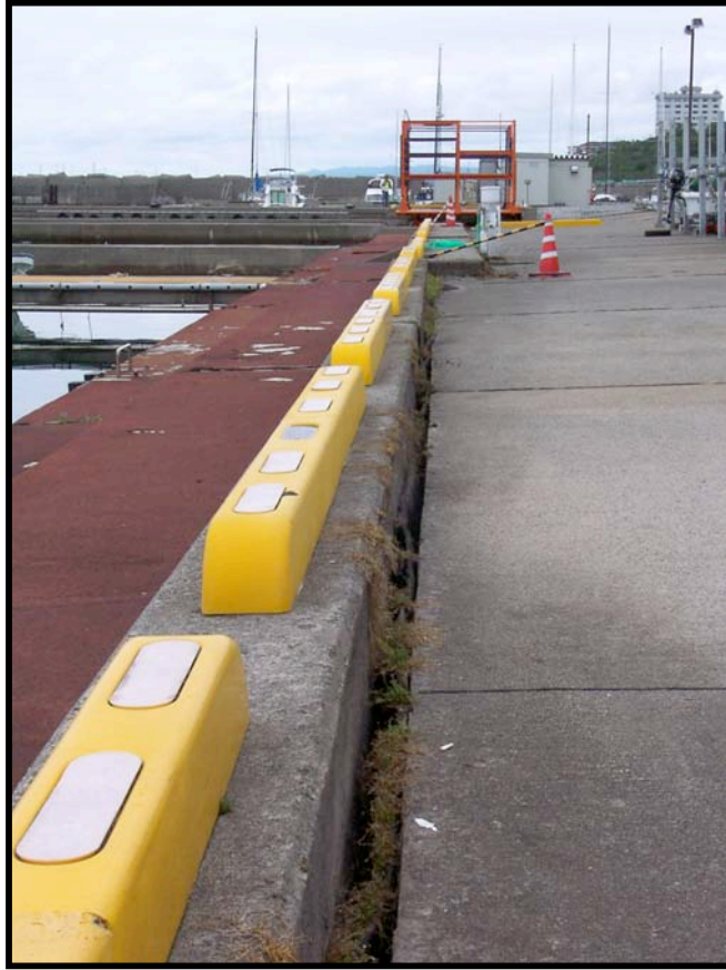
Figure 8.4: Kashiwazaki Marina - Evidence of minor lateral movement of quay walls and associated settlement of the paved apron (Site SD3, N37.36093° E138.52027°, photo taken 7/22/07 12:59).
