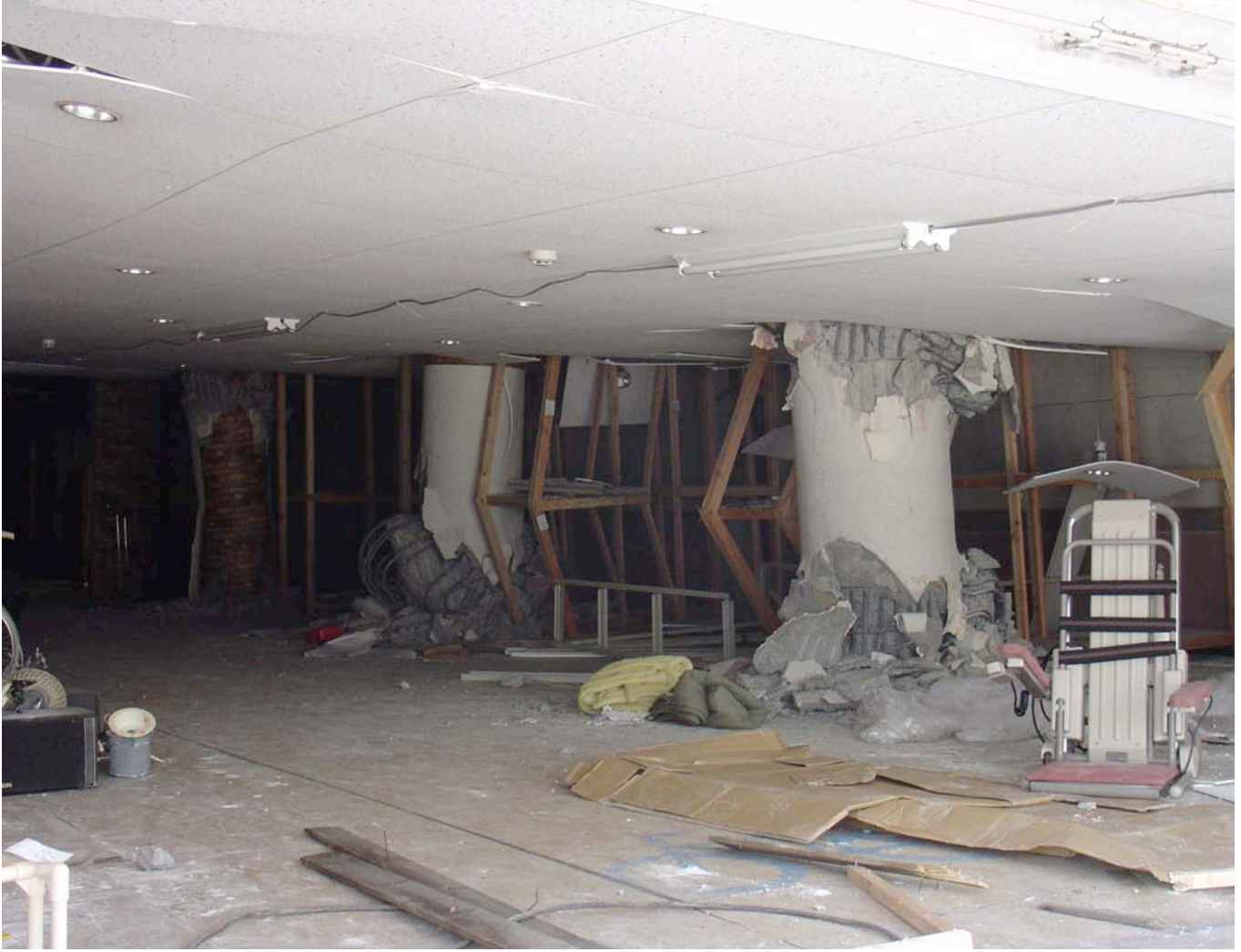
Figure 5.24: Shear failures of reinforced concrete columns (Site NIT-81, N37.37000° E13855825°, photo by Peter Yanev)
