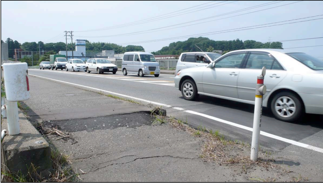
Fig. 6.19. Slight (10cm) settlement at bridge approaches.
