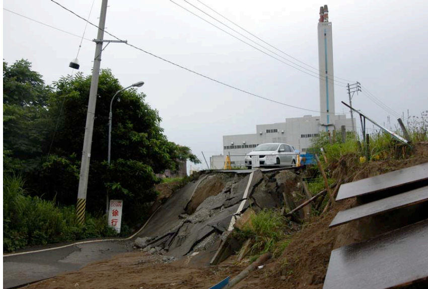
Figure 4.12: North side of Kai-Un Bridge area of the Sabaishi River - Lateral Spread on Road to Kashiwazaki Incinerator (Site RK6, N37.39343° E138.58555°, 7/19/2007). A zone of lateral spreading, sand boils and settlement crossing the present-day Sabaishi River, and that may be associated with a buried shoestring sand deposit of a former channel, resulted in failure of a road on the north side of the river adjacent to the Kashiwazaki Municipal Incinerator.
