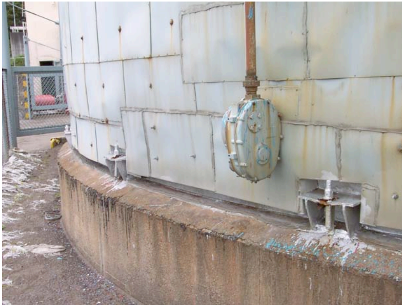
Figure 7.7: Kashiwazaki Port - Anchorage of asphalt storage tank (Located near Site RK25, N37.36713° E138.53210°, photo taken 7/22/07 12:37).
