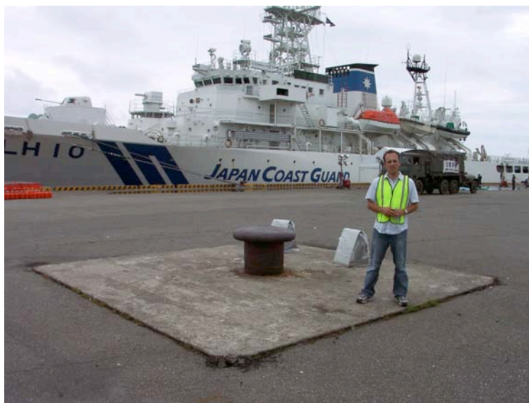
Photo 8.24: Kashiwazaki Port - Evidence of minor settlement adjacent to a pile-supported (?) bollard anchorage located along the northern face of the terminal used as the berth for the Japan Coast Guard (Site SD8, N37.36680° E138.53825°, photo taken 7/22/07 15:21).
