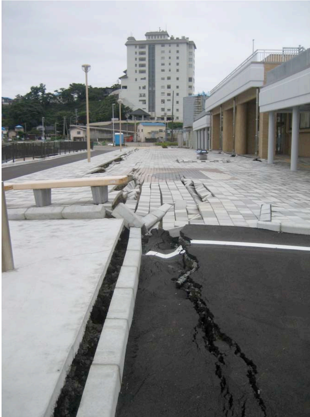
Figure 4.21: Kashiwazaki Harbor - The southern area experienced ground damage from liquefaction-induced lateral spreading and settlement. A harbor-front caisson rotated toward the harbor, to the left of the photo, initiating lateral displacement of the soil behind it, between the caisson and port building (Site RK25, N37.36713° E138.53210°, 7/20/2007).
