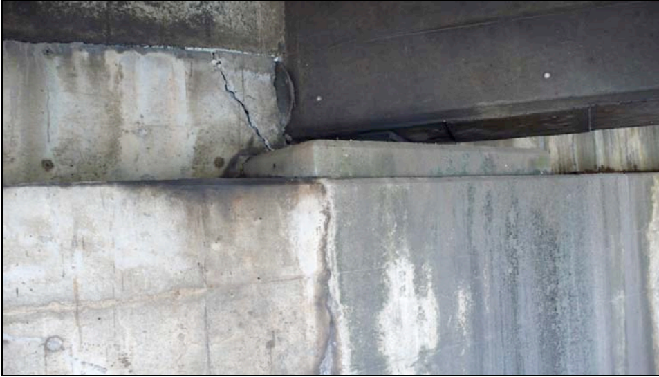
Fig. 6.52. Backwall-Diaphragm damaged by earthquake.
