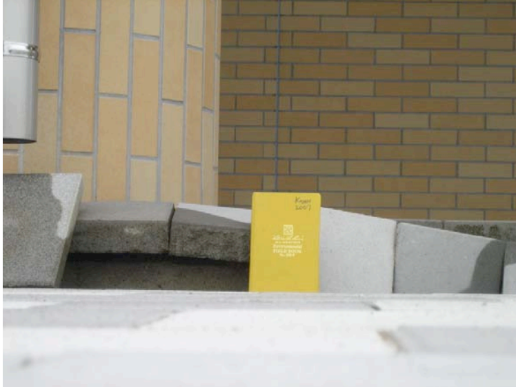
Figure 4.19: Kashiwazaki Harbor - South area experienced ground damage from liquefaction-induced lateral spreading and settlement immediately adjacent to the pile-supported port office building. (Site RK25, N37.36713° E138.53210°, 7/20/2007).
