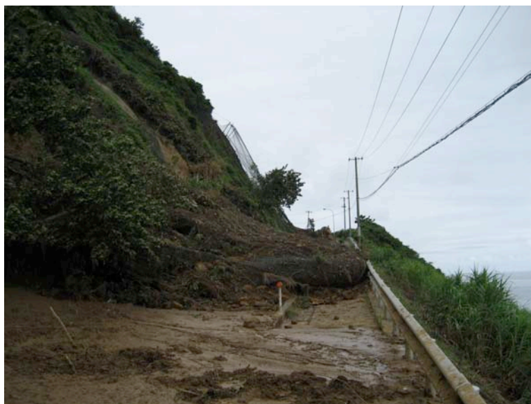
Figure 3.2: Coastal landslides on Highway 352 north of Kashiwazaki-Kariwa Nuclear Power Plant at road closure south of Route 373 (Site RK34; N37.48455° E138.62435°, photos taken 7/22/07 at approx. 10:45). This area consisted of at least eight individual slides. The landslide shown in the bottom photo consists of a slide in an area of previous instability - a shotcrete stabilization system is in effect for the bottom 50 m of this slope (total slope height is ~115 m), and overlain with a wire-mesh rock deflection system. The slide is approximately 50 to 60 m wide, 65 m long, and less than 1 meter thick. The landslide initiated above the shotcrete slope, moved into the wire-mesh and caused failure of the meshing and pull-out of the steel supports. The wire-mesh restrained most of debris, depositing the majority on the road, with only a slight quantity of the debris sliding over the road edge. The failure plane inclination is approximately 60°.
