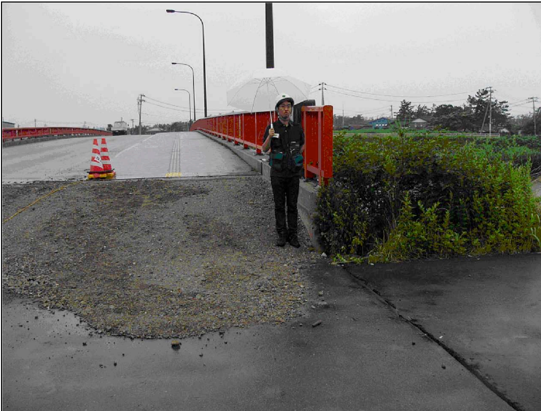
Fig. 6.41. About one meter settlement of south Kaiun bridge approach.
