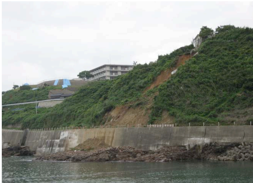
Figure 3.1: Shallow colluvial landslide located just north of the Kasashima Fishing Village, Site RK22/SA10; N37.33802° E138.46995°, photos taken 7/20/07 15:57 (top) and 7/21/07 13:35 (bottom). Dimensions are approximately 36 m wide, 24 m tall, 2 m thick. The lithology is composed of 24 m of weak mudstone overlying 6 m of more indurated, brecciated mudstone, which outcrops at the road. A 10 m tall concrete seawall leads down to the brecciated mudstone shore platform. The slide occurred in weak mudstone/colluvium, sliding over the brecciated mudstone, onto the road, and over the edge of the concrete seawall, spilling debris onto the shore platform at oceans edge.
