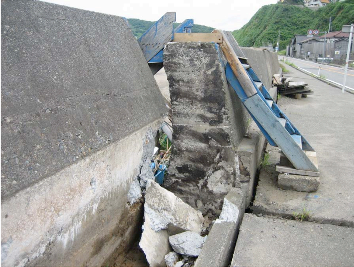
Figure 4.30: Concrete seawall deformations were on the order of 25 cm vertical (failed section up), and up to 64 cm horizontal, with a component of rotation as measured by 32 cm lateral deformation at the base of wall and 64 cm lateral deformation at 2 m height of wall. (Site RK35, N37.48497° E138.62645°, 7/22/2007).
