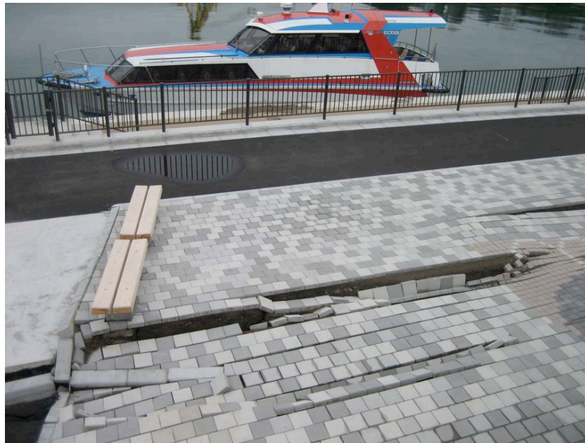
Figure 4.23: Kashiwazaki Harbor - The southern area experienced ground damage from liquefaction-induced lateral spreading and settlement. A harbor-front caisson rotated toward the harbor, uplifting the asphalt and tiled section shown here and initiating lateral displacement of the soil behind it, between the caisson and port building (Site RK25, N37.36713° E138.53210°, 7/20/2007).
