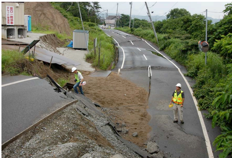
Figure 4.11: North side of Kai-Un Bridge area of the Sabaishi River - Lateral Spread on road to Kashiwazaki Municipal Incinerator (Site RK6, N37.39343° E138.58555°, 7/19/2007). A zone of lateral spreading, sand boils and settlement crossing the present-day Sabaishi River, and that may be associated with a buried shoestring sand deposit of a former channel, resulted in failure of a road on the north side of the river adjacent to the Kashiwazaki Municipal Incinerator.
