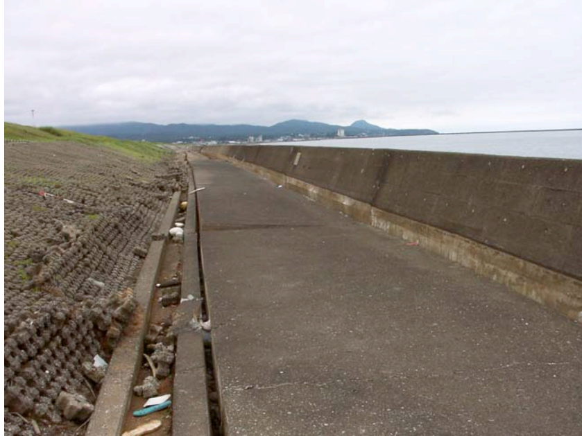
Figure 8.35: Evidence of seawall rotation, ground settlement, and longitudinal cracking of the benched embankment (Moving southwest of Site SD1, approximately N37.38868° E138.56413°, photo taken 7/22/07 11:25).
