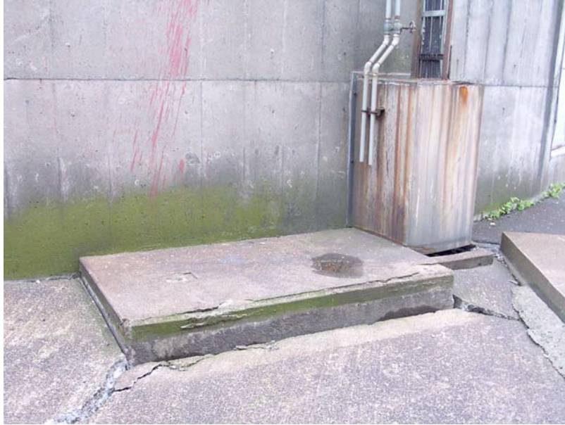
Figure 8.29: Kashiwazaki Port (Taiheiyo Cement Facility) - Evidence of minor to moderate settlement of sandy fill adjacent to one of the large diameter tanks (Site SD9, approximately N37.36665° E138.53983°, photo taken 7/22/07 15:48).
