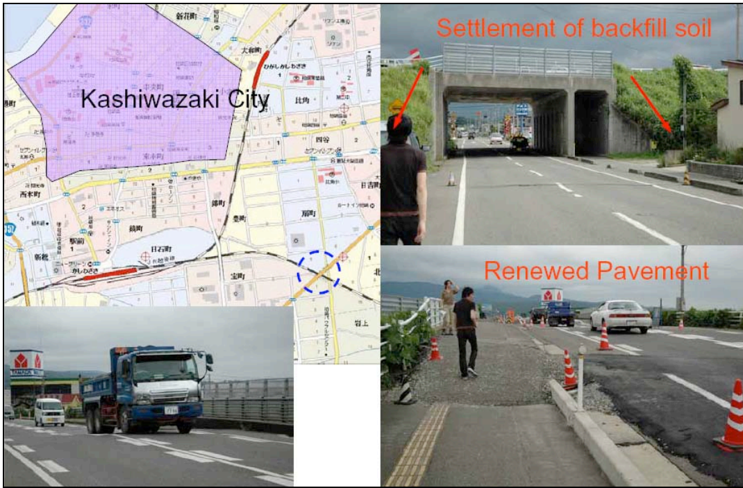
Fig. 6.16. Damage and repairs where Highway 8 crosses Route 522 Bridge (courtesy G. Watanabe, Tokyo Institute of Technology).
