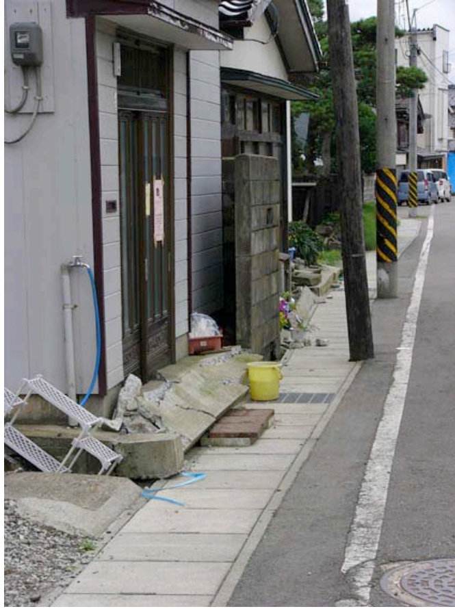
Fig. 4.42: Downtown Kashiwazaki Lateral Spread (SiteYT24, N37.36963°, E138.5486°, photo taken 7/22/07, SiteYT24_YT_03 as shown in Fig. 4.40).
