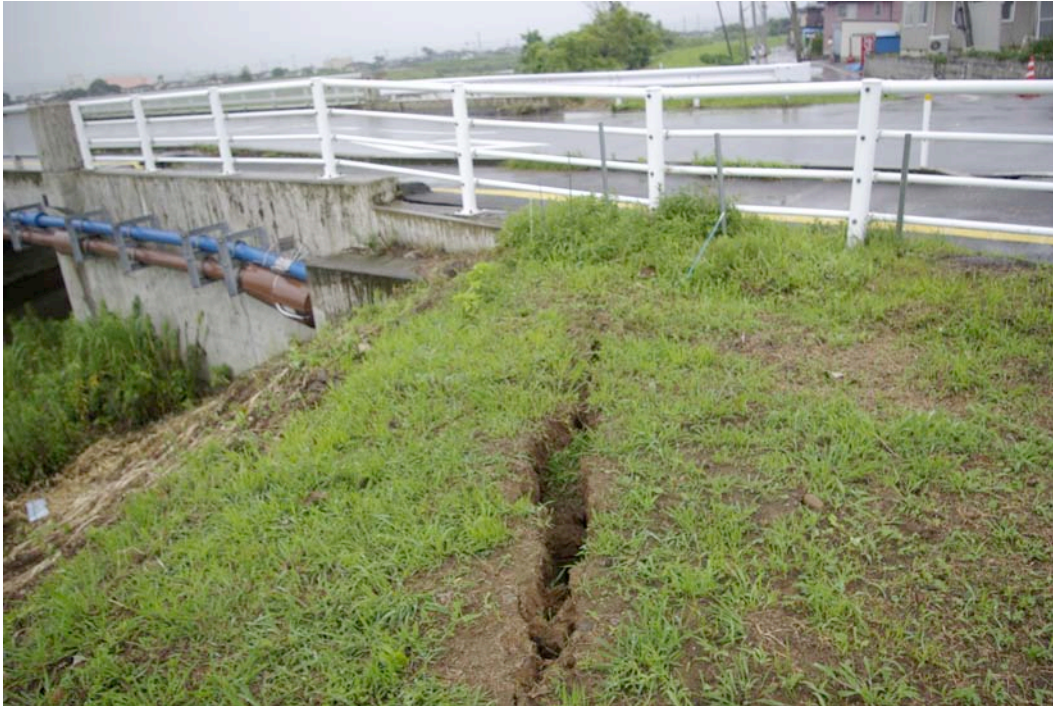
Figure 10.9: Evidence of moderate ground failure in an approach fill. Minor damage to the pipes was observed (Site RK7, N37.38940° E138.57393°, photo taken 7/21/07).
