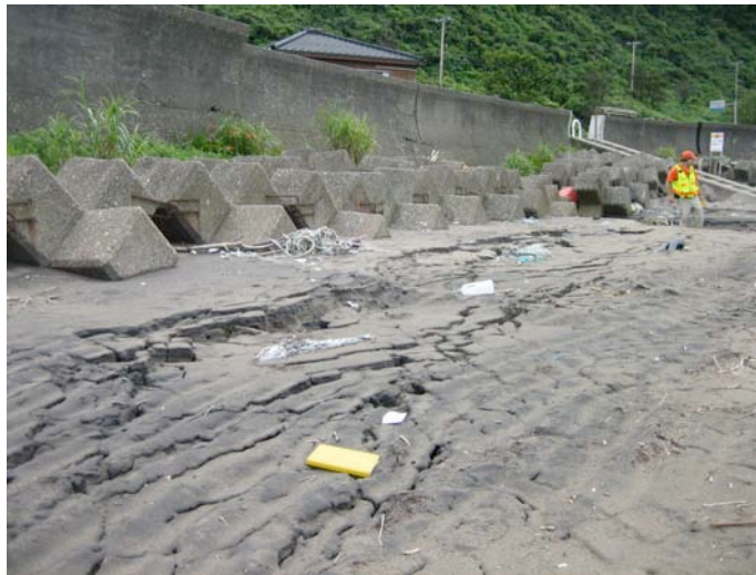
Figure 8.44: Lateral spreading associated with liquefaction of beach sand (Site RK35, N37.48497°, E138.62645°, photo taken 7/23/07).
