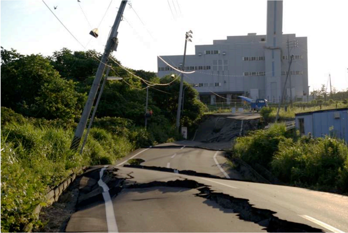
Figure 9.2: Road to Kashiwazaki municipal waste incinerator plant (Site RK6, N37.39343° E138.58555°, photo taken 7/24/07 18:06). Liquefaction-induced lateral spreading led caused the roadbed and associated slope to move southwards towards the Sabaishi River. Photos show formation of a 2.5 meter tall head scarp at the west end.
