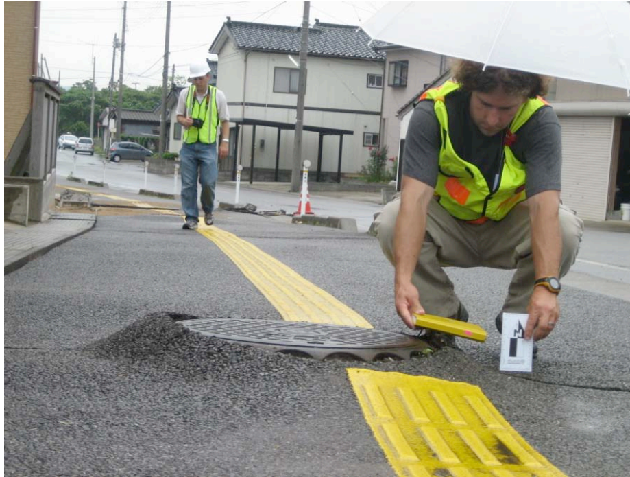
Figure 4.6: Kai-Un Bridge area Sabaishi River (Site RK4 N37.39233° E138.58063°, 7/19/2007, 1:40 p.m.). Numerous manholes on the southeast bank near the Sabaishi River uplifted in liquefied ground.
