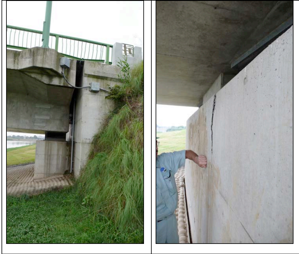
Fig. 6.36. The superstructure and bearings moved back and forth, cracking the abutment.
