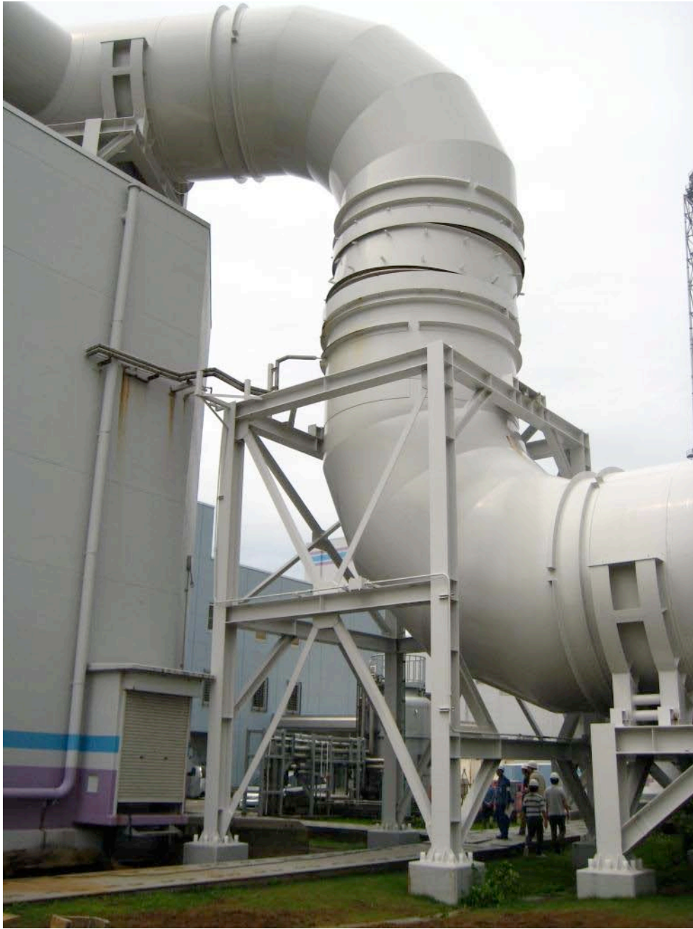
Figure 5.5: Failure of joint in exhaust pipe.
