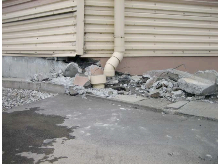
Figure 4.37: Plant 5 Store showing foundation corner area of failed reinforced concrete. (Site RK41, N37.41468° E138.60840°, 7/22/2007).
