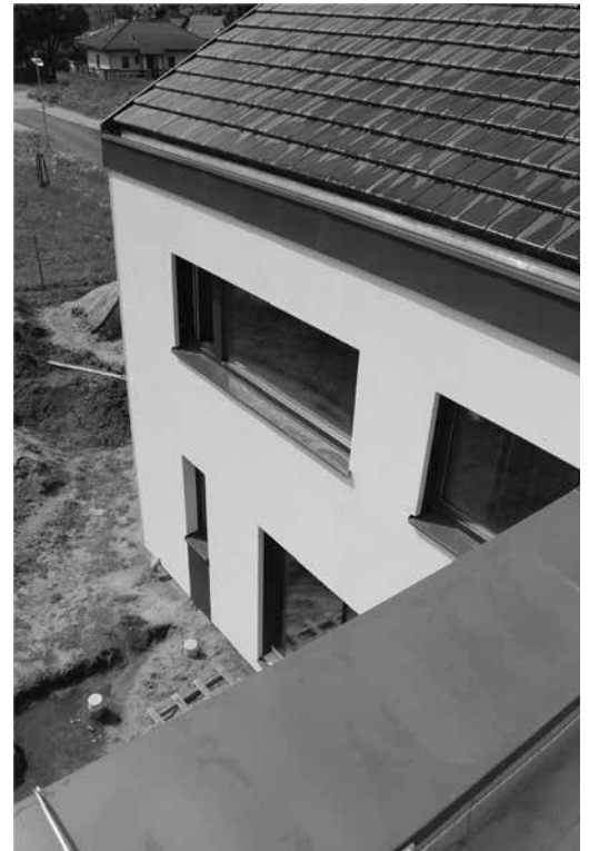
Picture 2: Actual photo of facade and gutter (Source: M. Pavlas)
