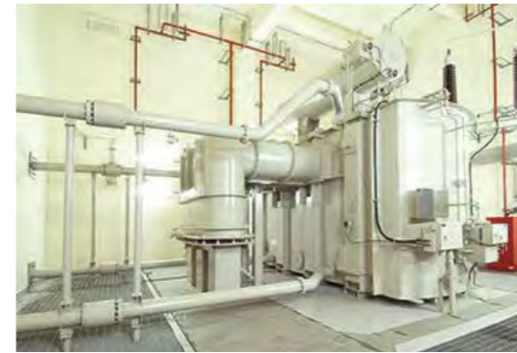
Scott Connected Transformer
