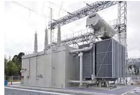
Roof-delta Connected Transformer
