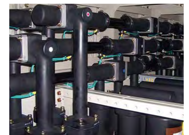
SIS Busbar Compartment
