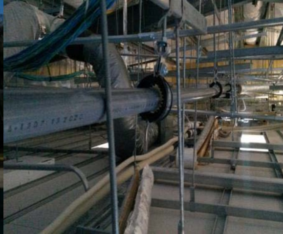
Resloped Condensate Drain
