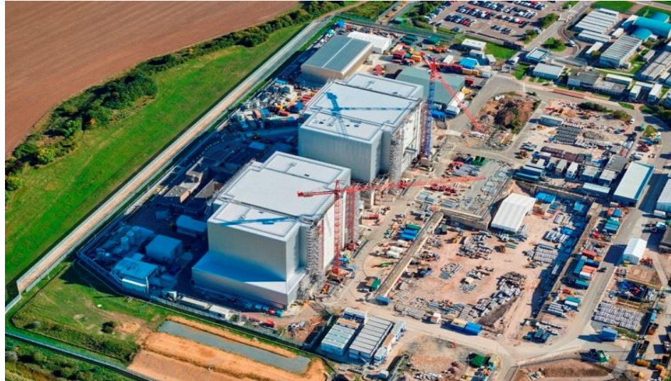
Figure 2. Aerial view of Bradwell in 2015 during the final stages of cladding installation.
