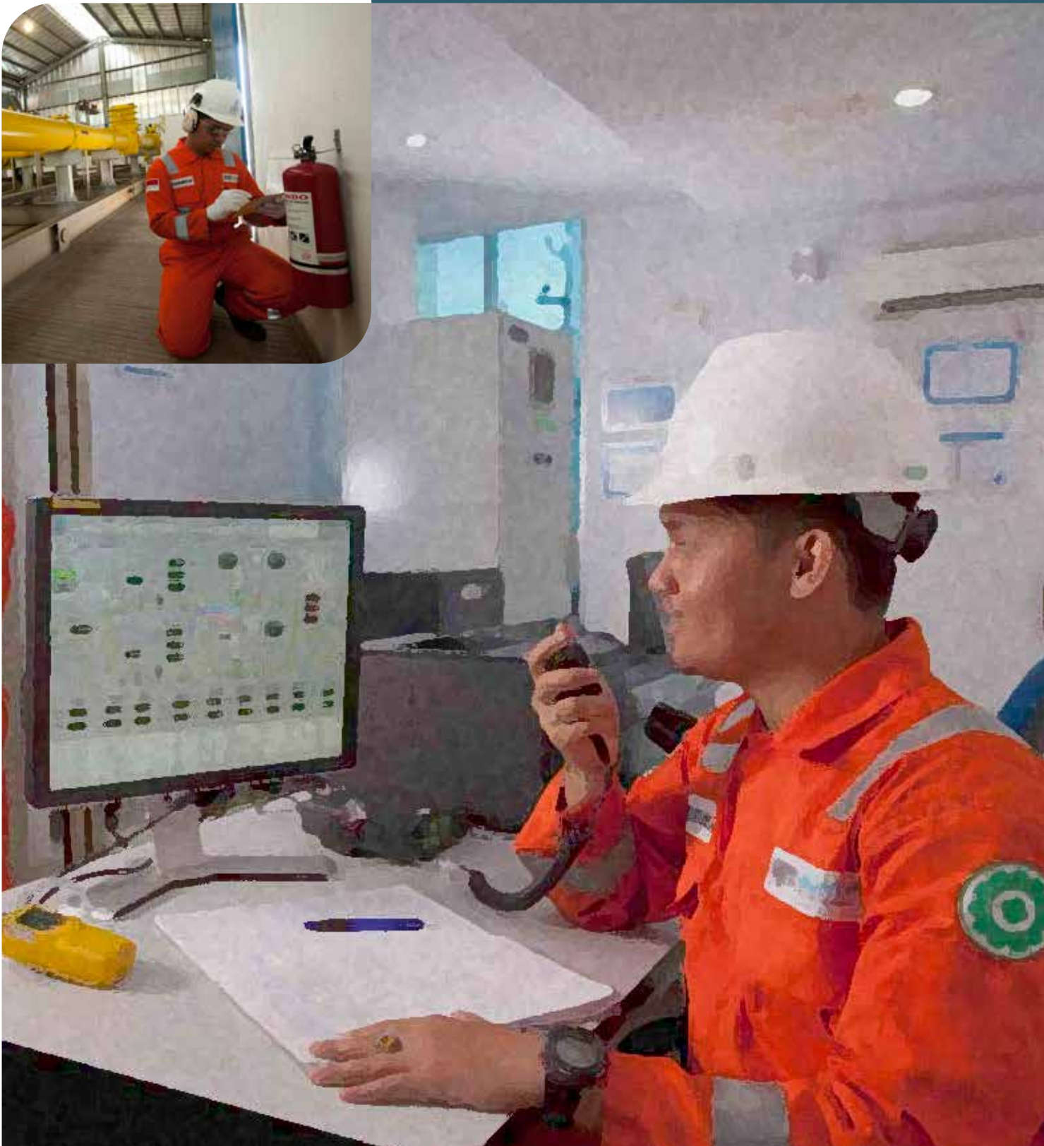
PGN is able to manage and control the pipeline channels long distance through the Supervisory Control and Data Acquisition (SCADA) System .
