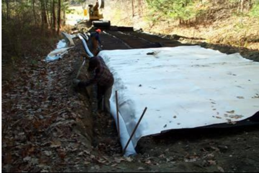
Figure 20. Geosynthetic capillary barrier drain (GCBD) installed on a test section over the subgrade/base interface in Vermont (Henry et al. 2005)
