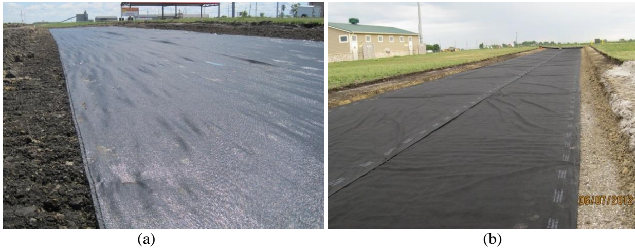
Figure 18. Geotextiles placed at subgrade/aggregate layer interface: (a) woven geotextile, and (b) non-woven geotextile (pictures from Boone County Expo Site, June 2012)
