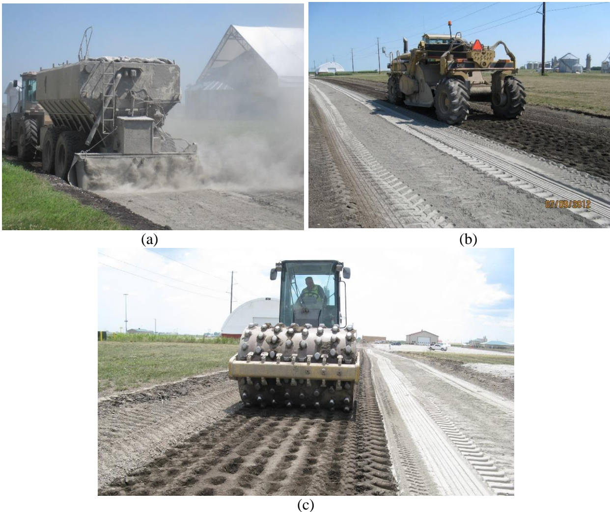
Figure 13. Photos showing typical chemical stabilization process: (a) spreading of cement stabilizer on subgrade, (b) mixing cement with subgrade material using a pulverizer, and (c) compaction of the soil-cement mixture using a padfoot roller (pictures from Boone County Expo Site, June 2012)
