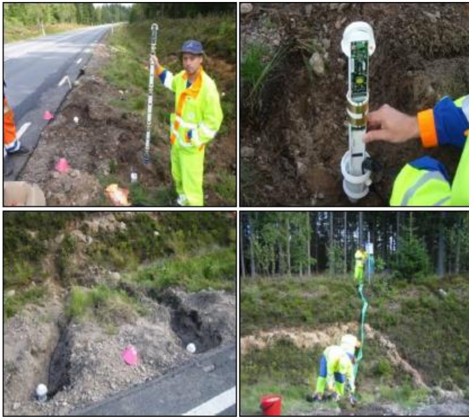
Figure 34. Moisture probes with wireless data transfer installation at a ROADEX project site in Southern Sweden (Saarenketo and Aho 2005)
