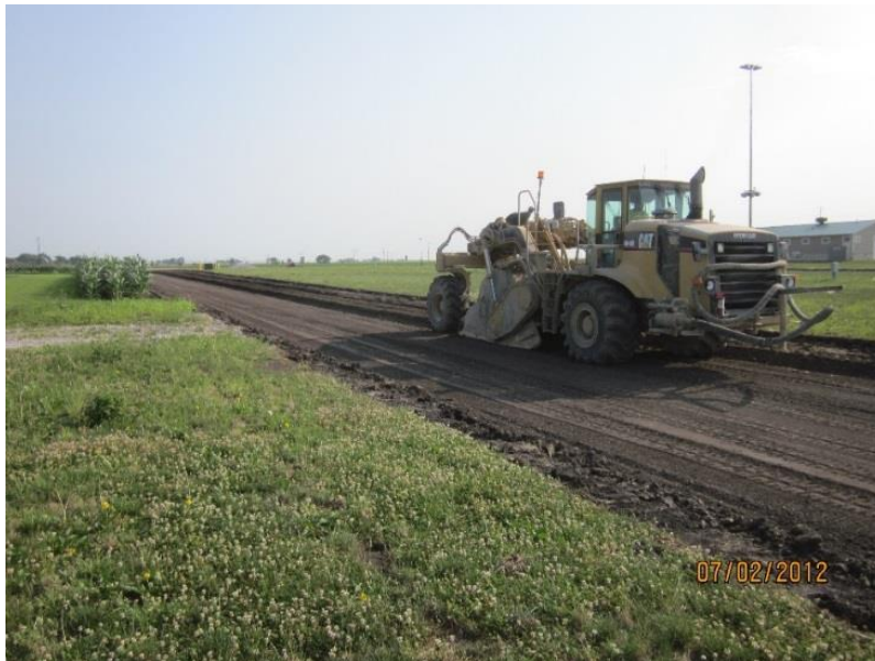
Figure 16. Blending granular material with subgrade using a soil pulverizer (picture from Boone County Expo Site, June 2012)
