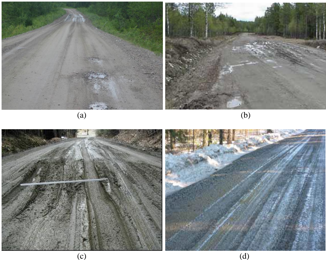
Figure 2. Freeze thaw damage on unpaved roadways: (a) potholes during July 2010 thawing season on a gravel road near Boden, Sweden (Christoffersson and Johansson 2011), (b) structural spring thaw damage on a moraine soil in Kemijarvi, Finland (Saarenketo and Aho 2005). (c) rutting damage on a gravel road in Vermont shortly after adding 6 in. of gravel to saturated subgrade in April 2002 (Henry et al. 2005), (d) early phase of surface thaw weakening on a gravel road in Finland (Saarenketo and Aho (2005))
