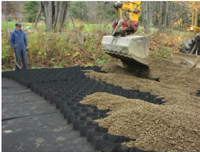
Figure 21. Geocells placed over non-woven geotextile on a test section in Vermont (Henry et al. 2005)
