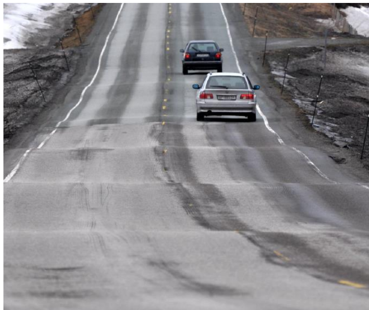
Figure 3. Frost-heave pavement damage in Norway (Ystenes 2011)
