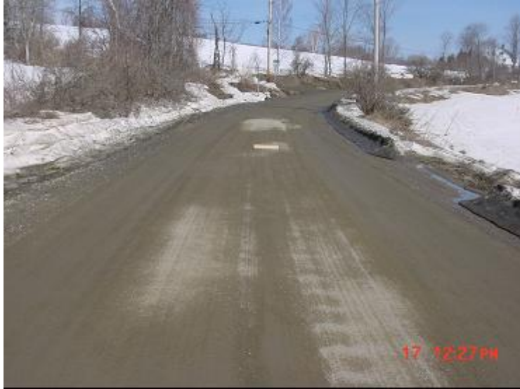
Figure 14. Cement stabilized section during thawing period from a test site in Vermont (picture from March 17, 2003, Henry et al. 2005)
