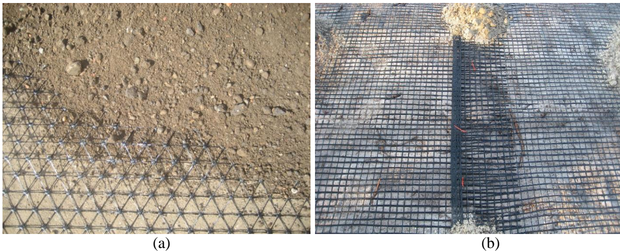
Figure 19. Polymer geogrids placed at subgrade/aggregate layer interface: (a) triaxial geogrid, and (b) bi axial geogrid (pictures from Boone County Expo Site, June 2012)
