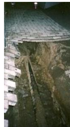
Fig. 5.17. Collapse of sidewalk pavement caused by deterioration of underground water pipelines, leakage and consequent soil erosion.
