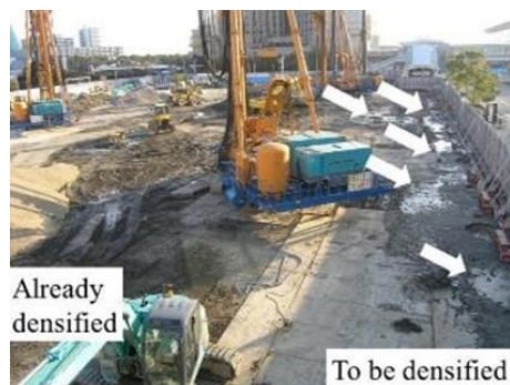
Fig. 4.45 (b) Contrast between densified and untreated parts of a sand compaction project (2011). Liquefaction and sand ejecta only at the surface of the untreated part (see arrows)
