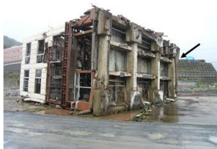
Fig. 4.58. Building in Onagawa Harbor, Japan, toppled by tsunami in 2011; a steel pile is hanging next to the base slab (shown by arrow).
