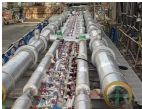
Fig. 5.3. Coolant pipelines for construction of frozen underground wall that prevents water from flowing into the radioactively contaminated basement of reactor buildings.
