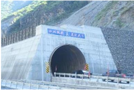
Fig. 4.30. Protection of road traffic by tubular steel tunnel embedded in concrete (Sichuan Province, China)
