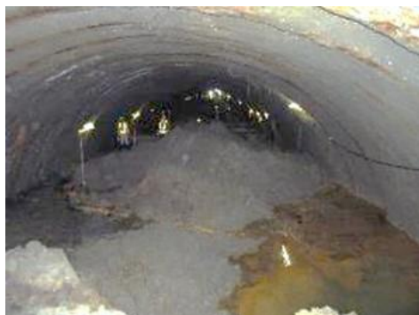
Fig. 3.5. Tunnel collapse after hitting the bottom of an unlithified sand pipe with water.
