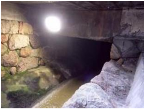
Fig. 4.2. Pre-modern sewage system in Osaka, which was originally constructed in the 16th Century as an open channel and was later covered.
