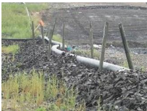
Fig. 5.6. Collection of CH 4 gas from municipal waste landfill in Delaware, USA.
