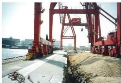
Fig. 4.19. Liquefaction-induced damage in Port Island of Kobe Harbor in 1995.
