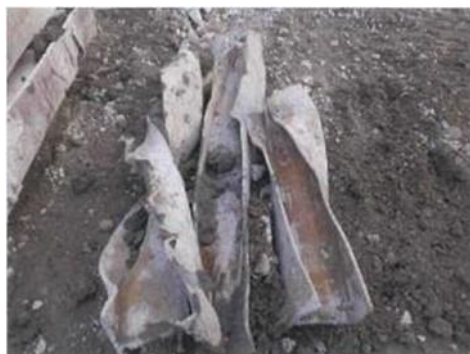
Fig. 3.6. H-steel pile foundation of temporary structures for basement excavation during the construction of previous building 50 years ago (their location was not documented for future construction).
