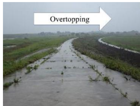
Fig. 4.41. Lower section of river levee where flood water overtops intentionally (Ohkubo Retention Basin, Japan).
