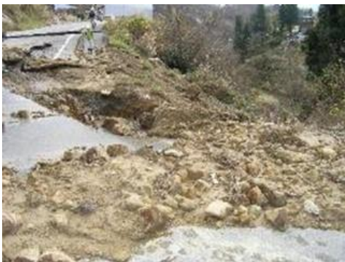
Fig. 5.15. Coseismic failure of road embankment made of crushed mud stone that absorbed water and got deteriorated (slaking) after many years (Niigata Chuetsu earthquake, 2004).
