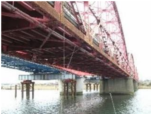
Fig. 5.14. Deteriorated steel bridge immediately before its scheduled demolition.
