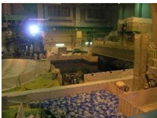
Fig. 5.1. Storage of used nuclear fuel in water pool inside a reactor building (Kashiwazaki-Kariwa Nuclear Power Plant).
