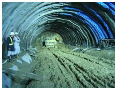
Fig. 4.26. Construction of the Uodzu No. 2 Tunnel in Toyama, Japan, by means of the New Austrian Tunnelling Method.
