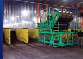
Agitated and Aerated In-vessel type Composting System (ICS)
