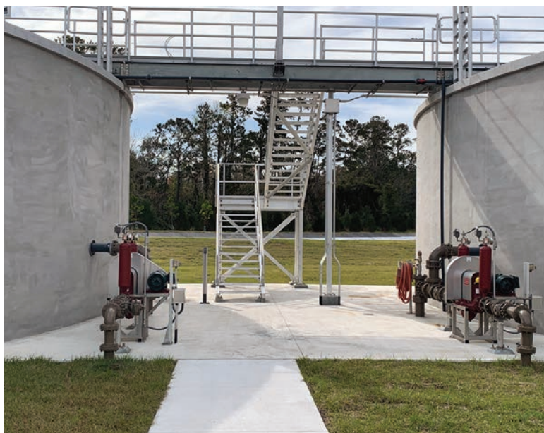
At the Players Club Water Reclamation Facility in St. Johns County, Florida, a scum pump installation was piped directly to the scum collection trough.
