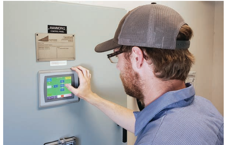
Alex Krause, wastewater operator, optimizes the airflow control on the AnammoPAQ reactor control panel (Ovivo-Paques).
