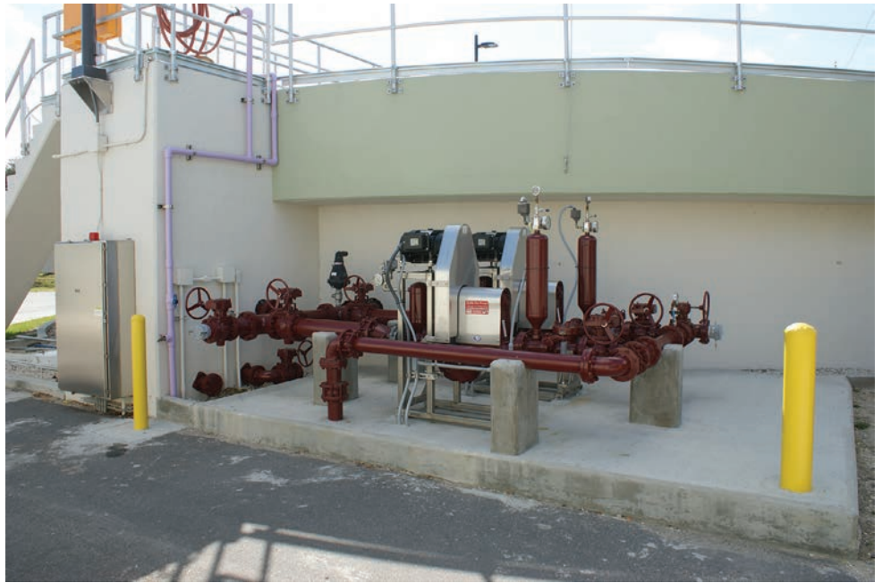
At the Osprey Water Reclamation Facility in Titusville, Florida, a wet well was abandoned and a clarifier was retrofitted with double disc pumps (Penn Valley Pump) piped directly to the scum trough.
