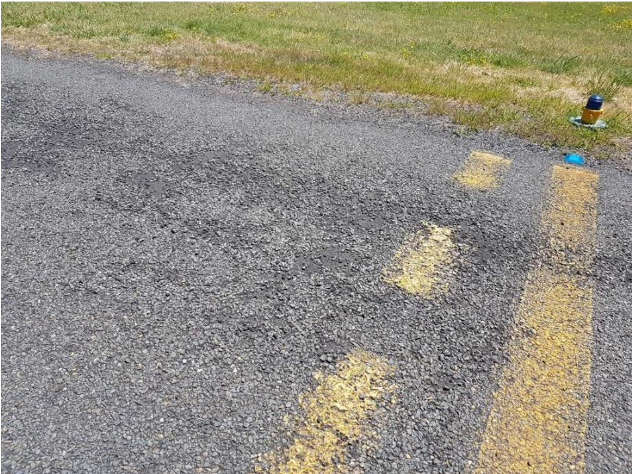
Photo showing chip loss on Taxiway
