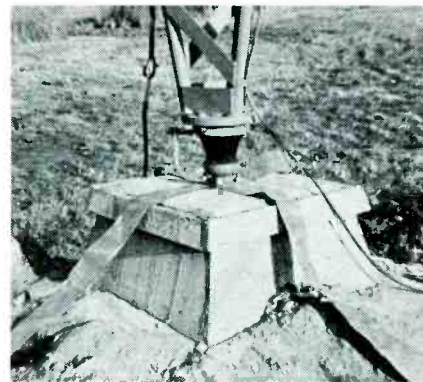
Fig. 10. Power is fed across insulator on both the broadcast and 80-meter bands.
